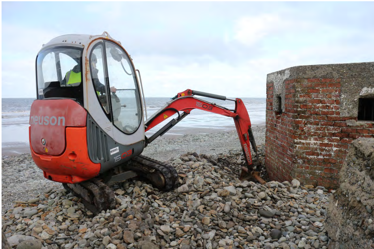
Neuson 1503 mini-excavator cleaning back beach pebbles to reveal lower brickwork courses, IMG_9773, 03.03.2016
