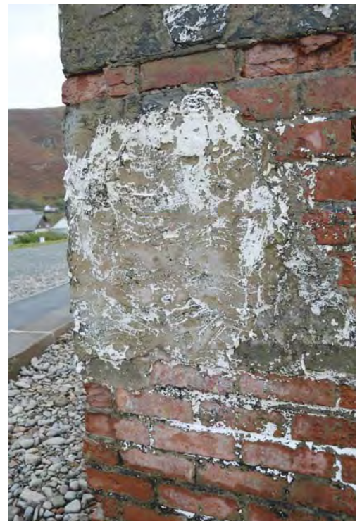
Plate 26. Patch of render on north-east elevation (29/10/2015)
