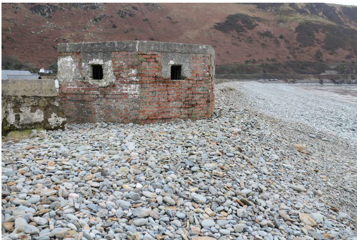
Shingle beach seaward of pillbox after erosion during Storm Imogen, IMG_9764, 03.03.2016
