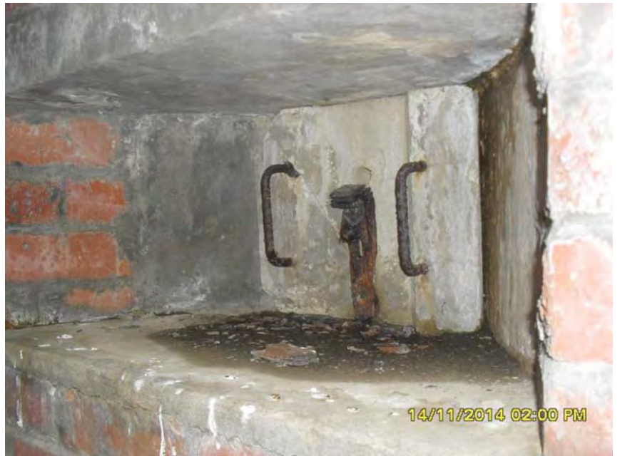
Plate 8. Embrasure plug fitted in position in the pillbox at Egryn, near Llanaber. Internal view. (Photo taken by Matt Rimmer)
