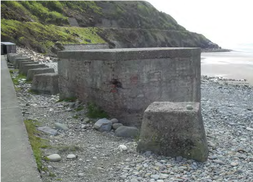
Plate 7. Traces of render surviving on pillbox PRN 34150 before its destruction (Photo taken by Matt Rimmer 2013)
