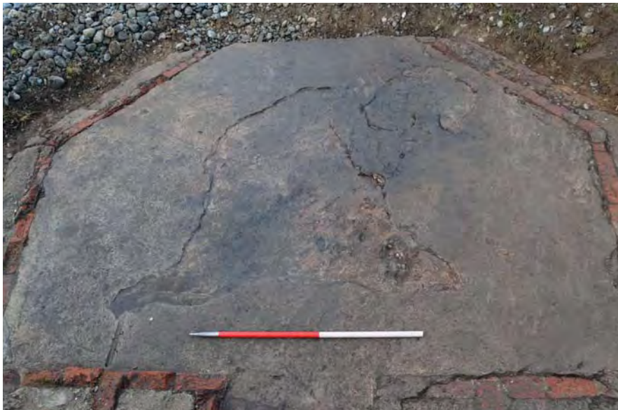
Plate 34. Floor of pillbox showing roughly Y-shaped damage to the screed and impressions in the screed on the southern/left side (28/10/2015)
