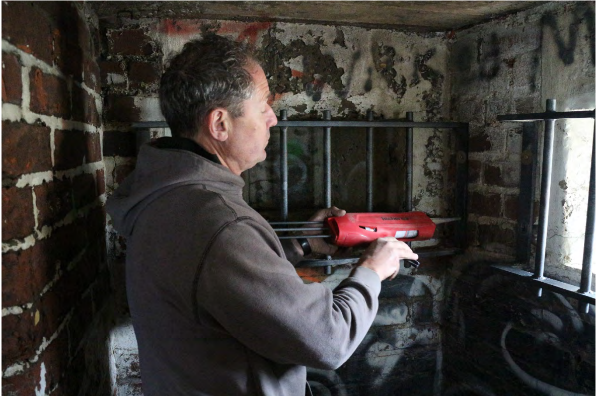
Securing stainless steel anchor pins using Fischer FIS VT 380 C vinyl ester solid injection mortar, IMG_8339, 27.10.2015
