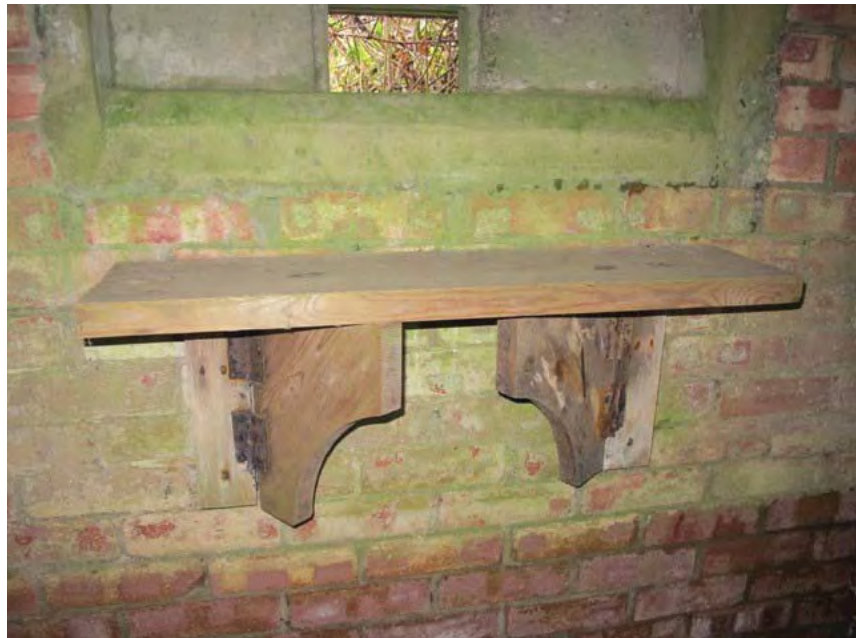
Plate 14. Surviving example of a folding shelf within a pillbox in England; Image courtesy of Tim Denton of the Pillbox Study Group
