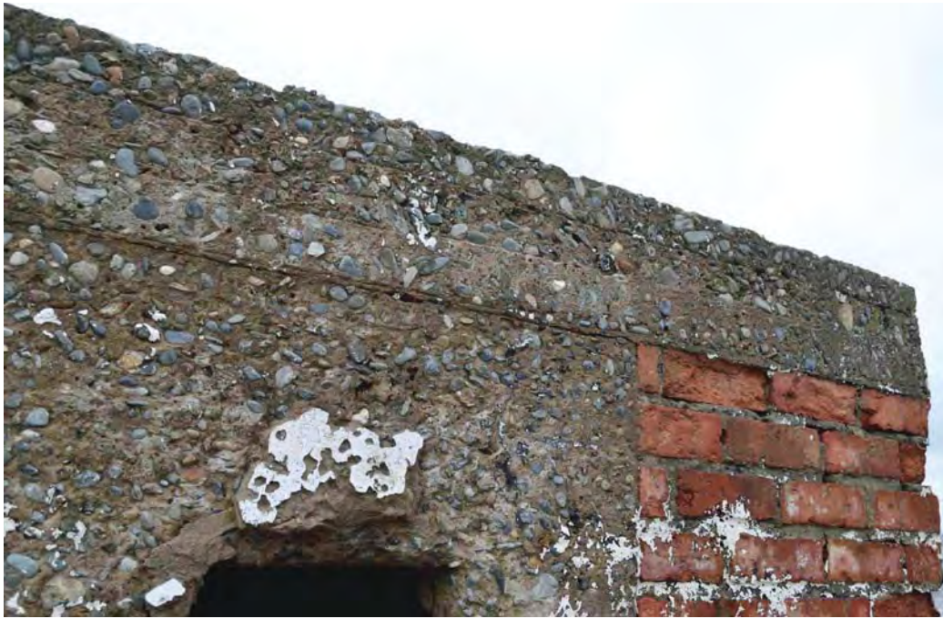
Plate 20. Edge of the roof on the south-east side showing it built up in three layers (29/10/2015)
