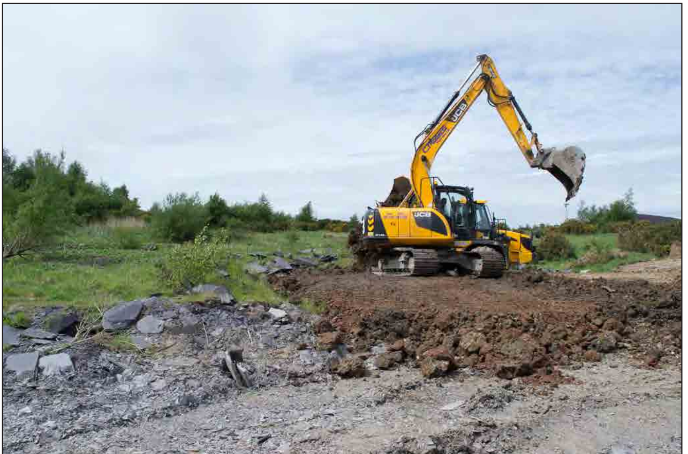
Plate 08: Working shot showing the preservation in situ of the earthwork. View from the south.
