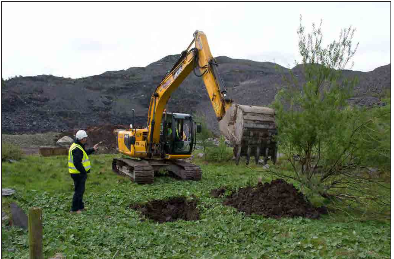
Plate 06: Working shot showing the excavation of a trial hole within the earthwork. View from the north.
