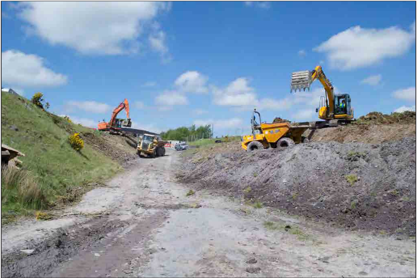
Plate 09: Working shot showing the groundworks at the northern ed of the site. View from the South.
