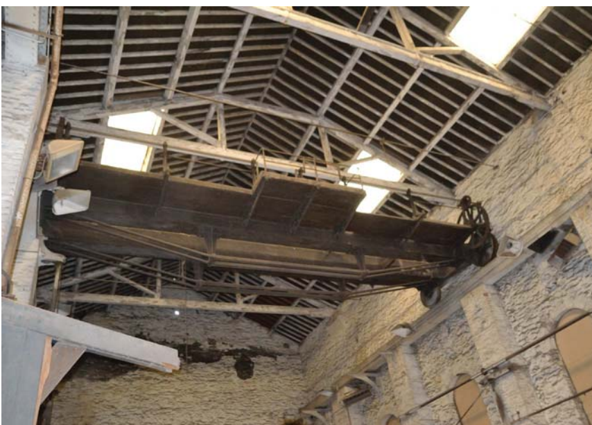
Plate appII.8. Crane in boiler shop (PRN 11824)
