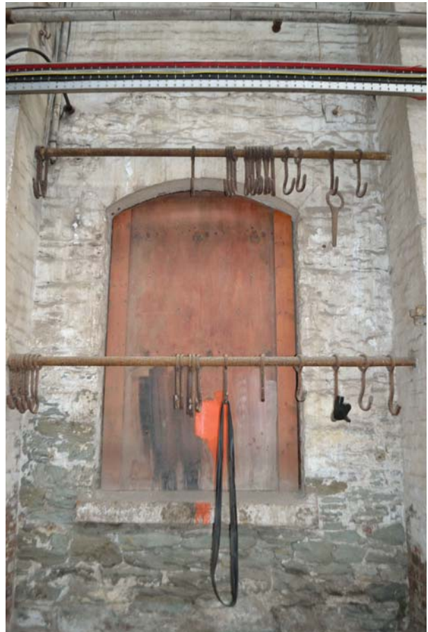
Plate appII.14. Hooks for block and tackle in erecting shop (PRN 33998)
