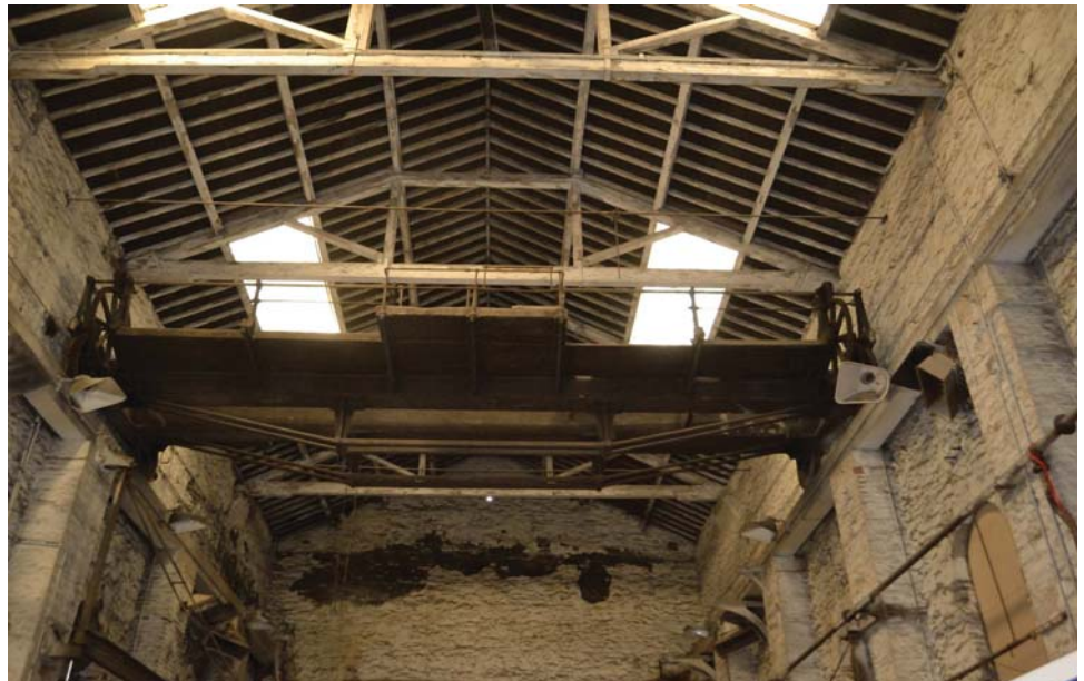
Plate 20. Crane in boiler shop in Marine Yard (photograph by Martin Simpson and Hanna Hillyer)
