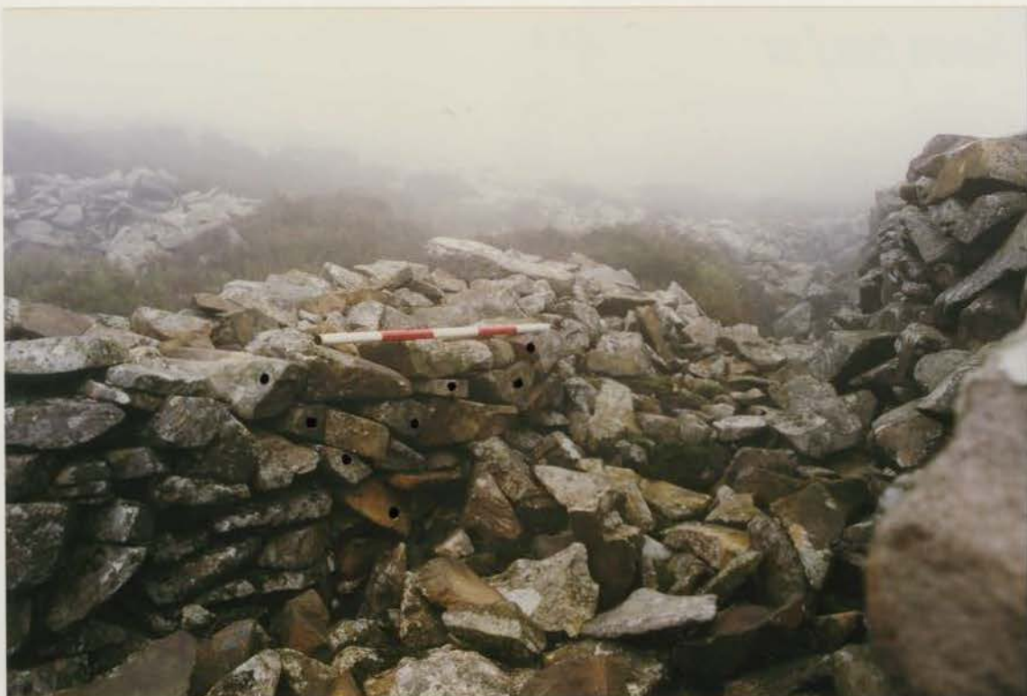
Plate 182 G1022/212/26 ; Collapse 42a after conservation.
