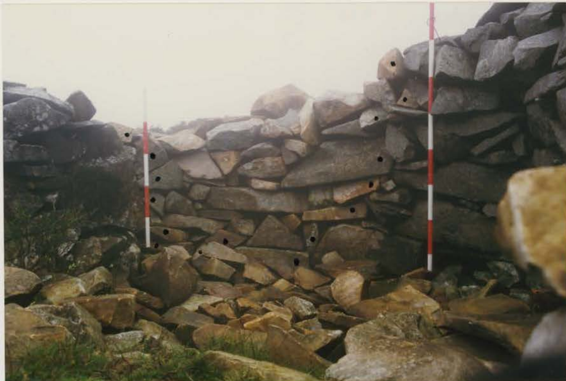
Plate 235 G1022/212/25; Collapse 137a after conservation.
