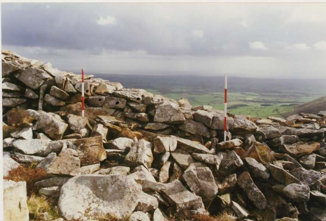
Plate 29 G1022/208/08 ; Collapse S10 after conservation.
