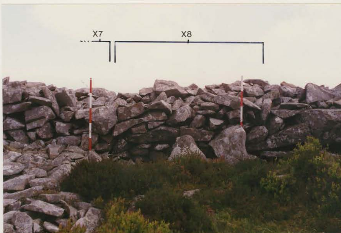
Plate 145 G1022/196/30 ; Collapse X8 before conservation.
