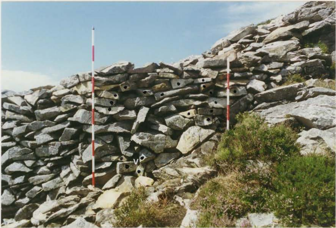
Plate 7 G1022/205/14 ; Collapse S1 after conservation.
