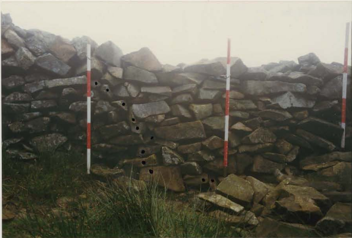
Plate 213 G1022/213/01 ; Collapse 9b (central) after conservation.
