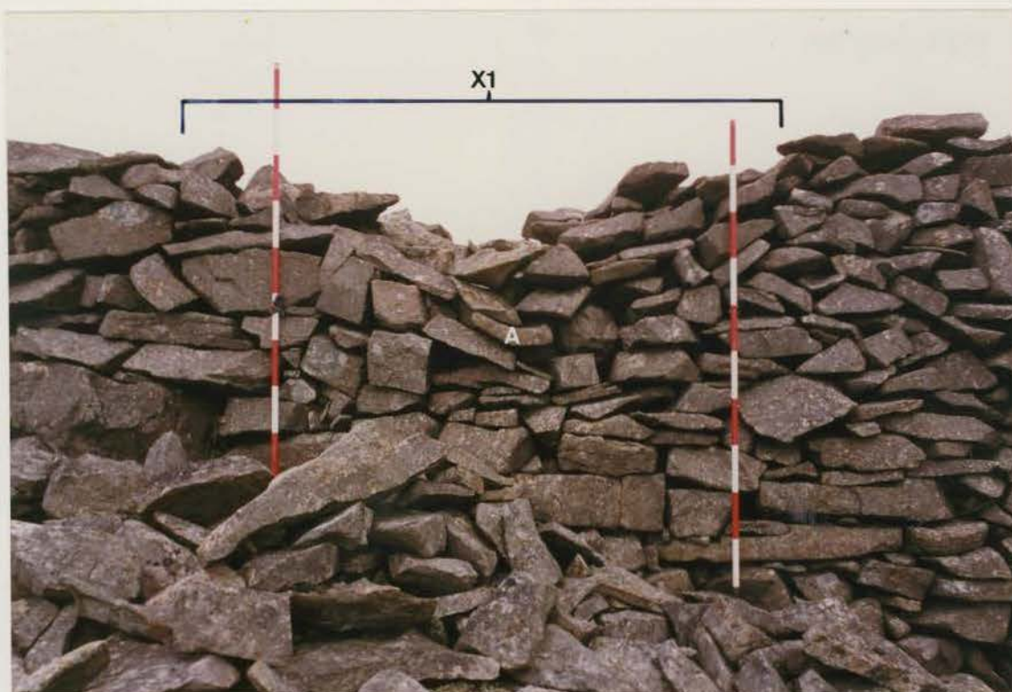
Plate 85 G1022/198/30 ; Collapse X1 before conservation.
