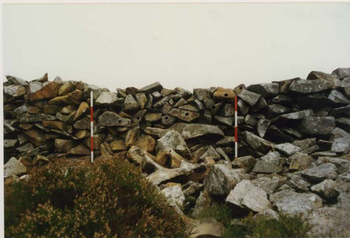
Plate 138 G1022/210/27 ; Collapse X4 after conservation.
