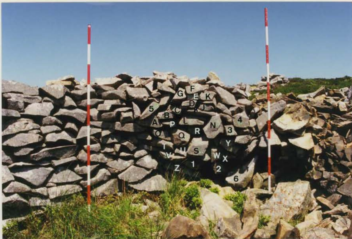
Plate 202 G1022/202/09a; Collapse 9a, unstable masonry, before conservation.
