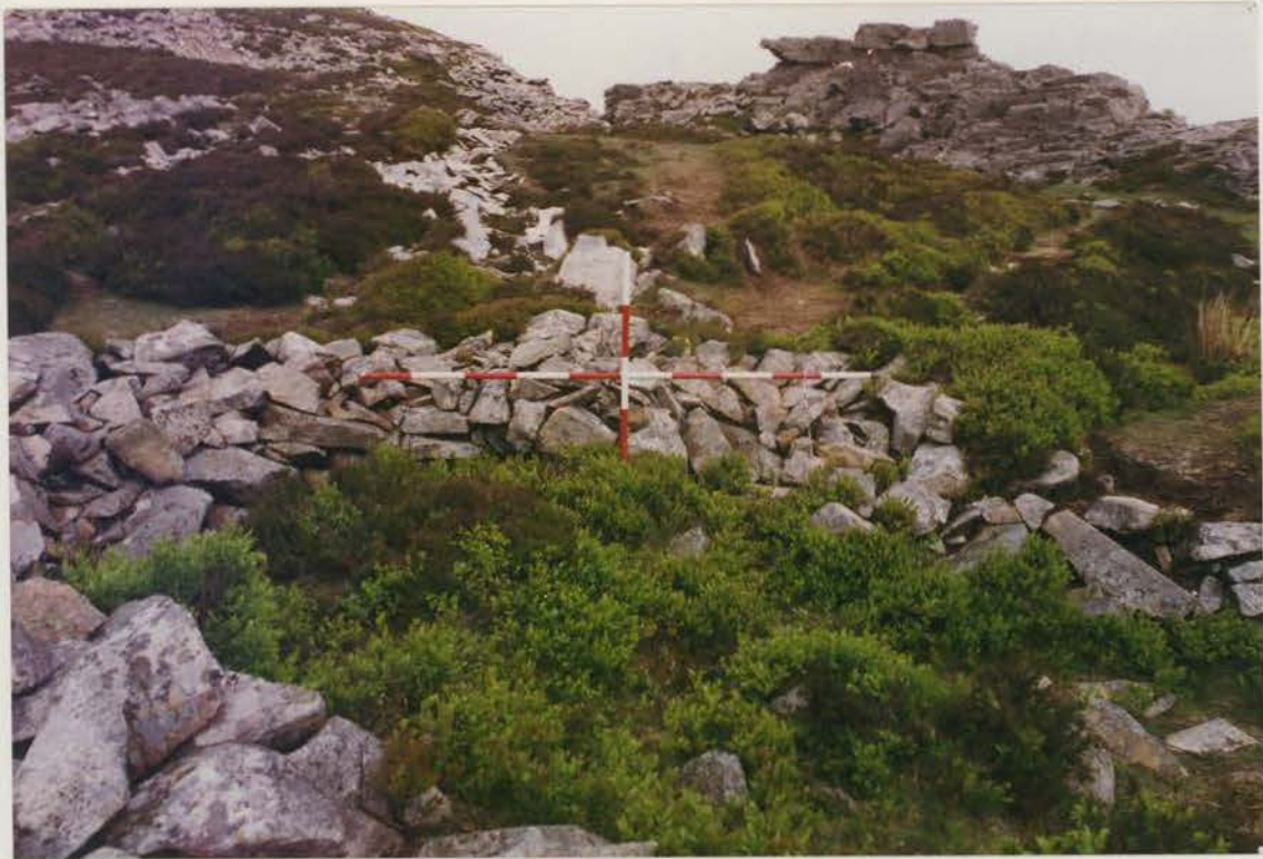
Plate 153 G1022/199/04 ; Collapse 45Ac before conservation.
