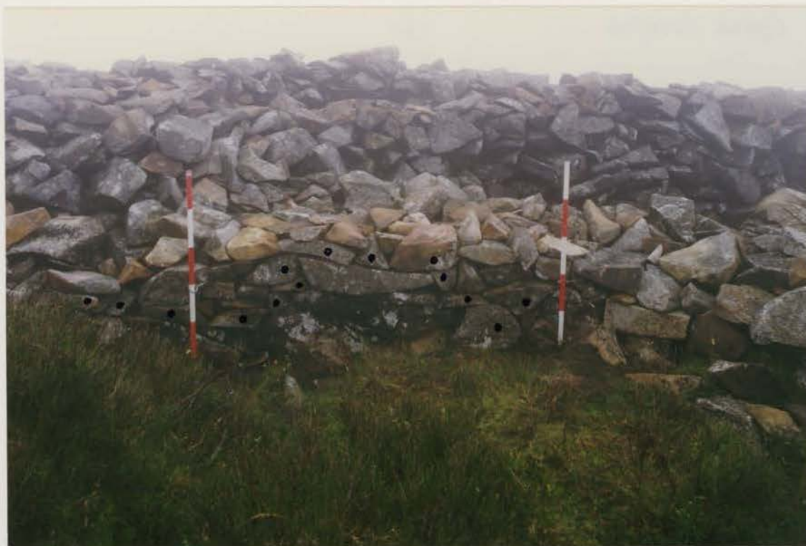
Plate 165 G1022/212/08 ; Collapse 108a after conservation.
