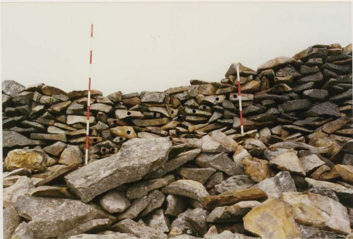
Plate 42 G1022/207/23 ; Collapse S6 after conservation.
