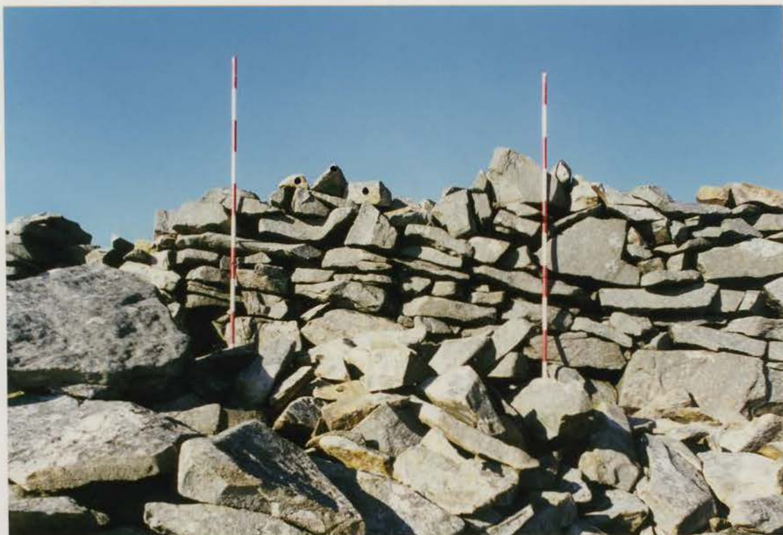
Plate 90 G1022/211/17 ; Collapse X2 after conservation.
