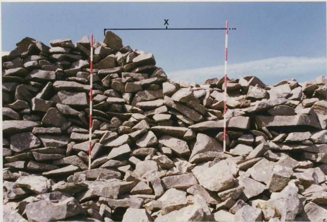
Plate 81 G1022/198/11 ; Collapse X before conservation.
