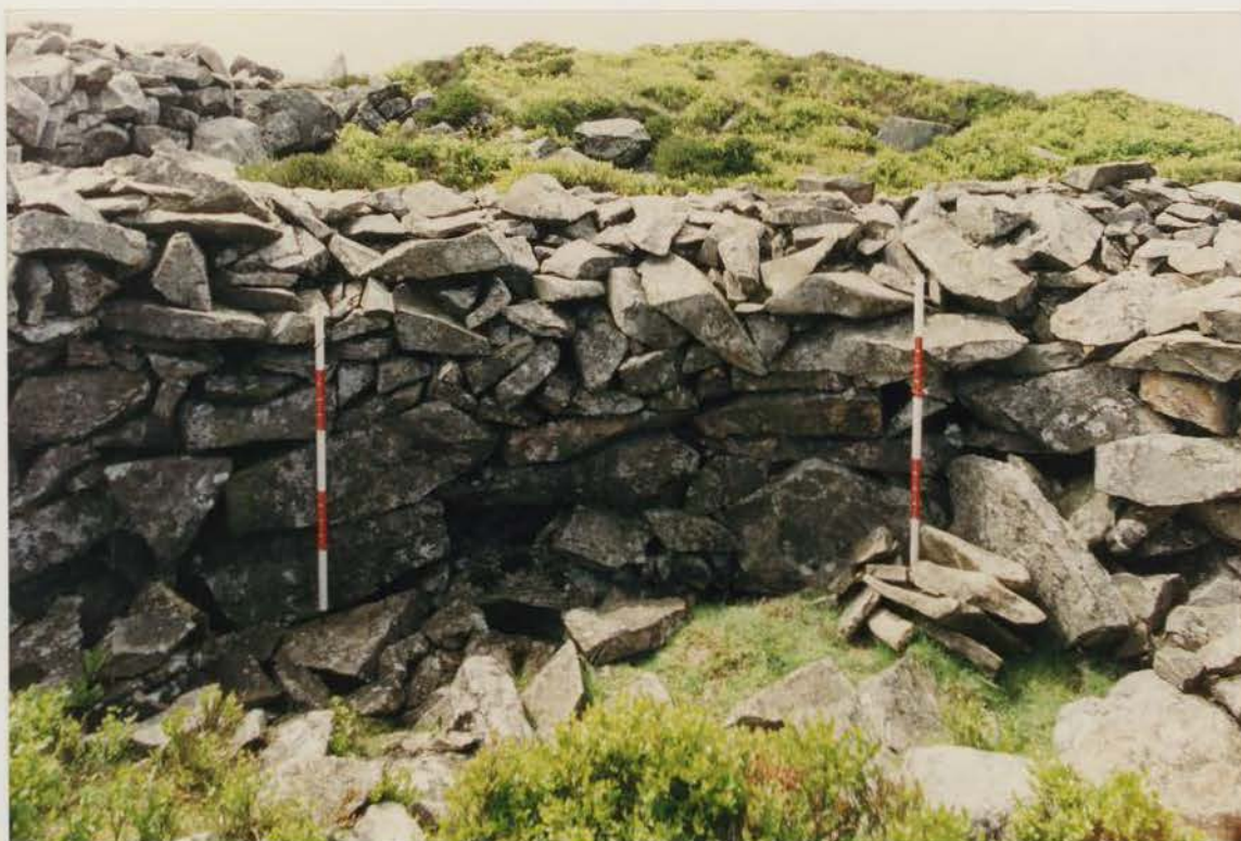
Plate 194 G1022/200/26a; Collapse 41c (central) before conservation.
