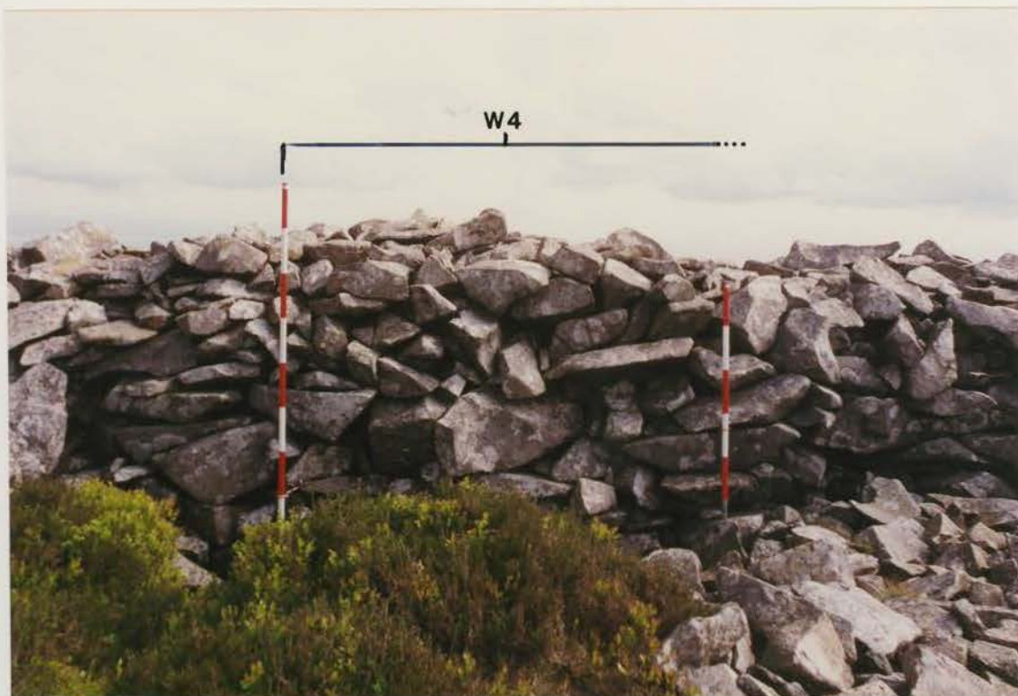
Plate 126 G1022/196/08 ; Collapse W4 before conservation.
