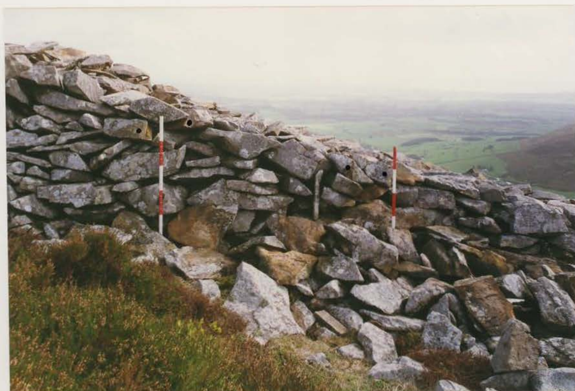
Plate 28 G1022/208/06 ; Collapse S10 after conservation.
