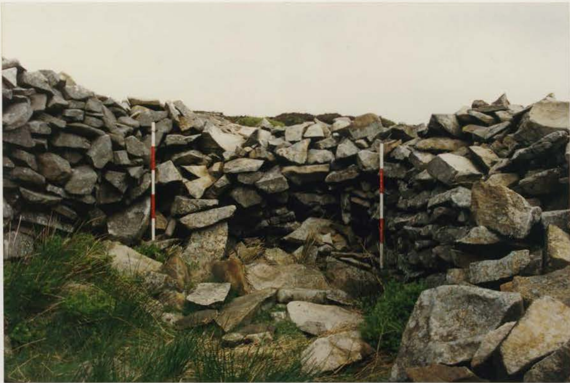
Plate 201 G1022/200/35a; Collapse 9a before conservation.
