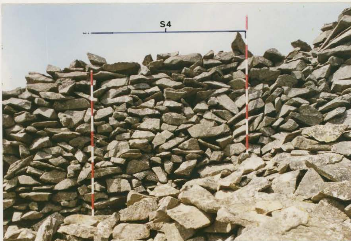
Plate 13 G1022/193/26 ; Collapse S4 before conservation.
