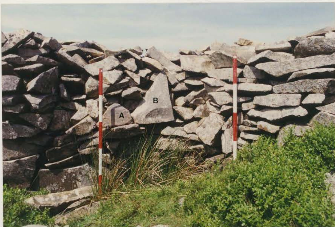
Plate 231 G1022/201/26 ; Collapse 10d before conservation.
