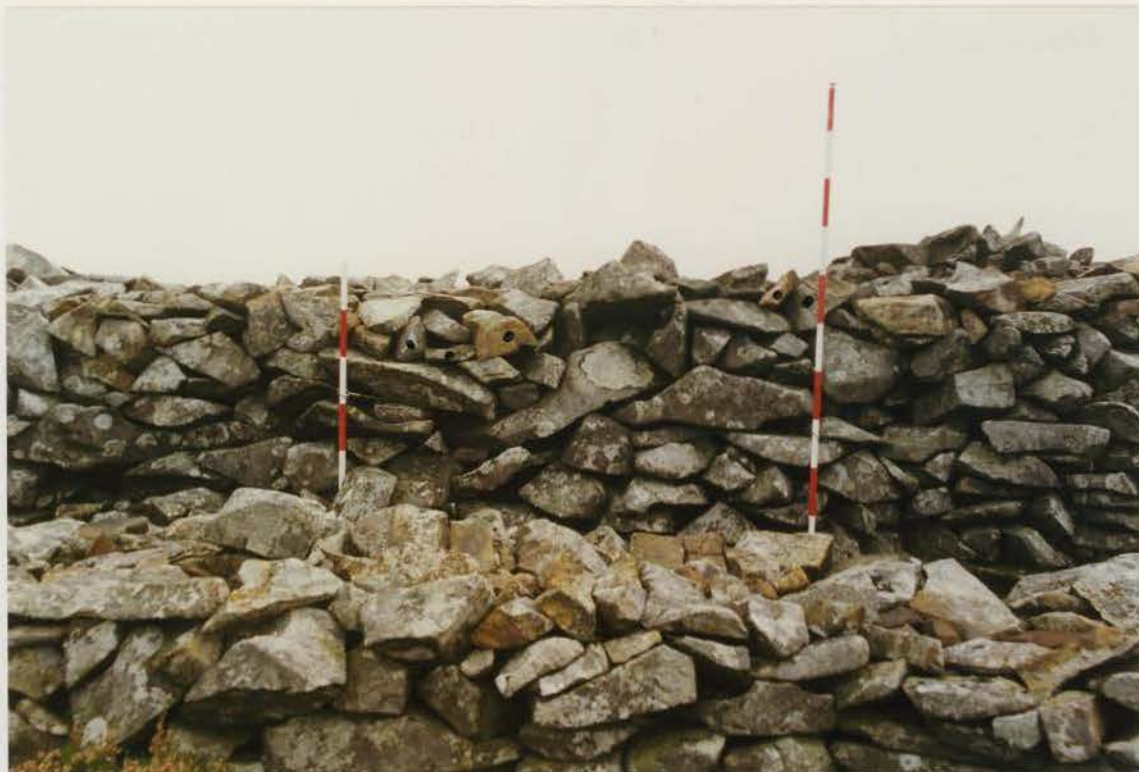
Plate 131 G1022/210/21 ; Collapse X after conservation.
