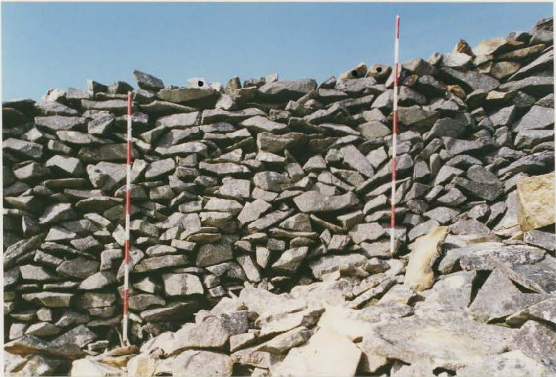
Plate 15 G1022/207/16 ; Collapse S4 after conservation.
