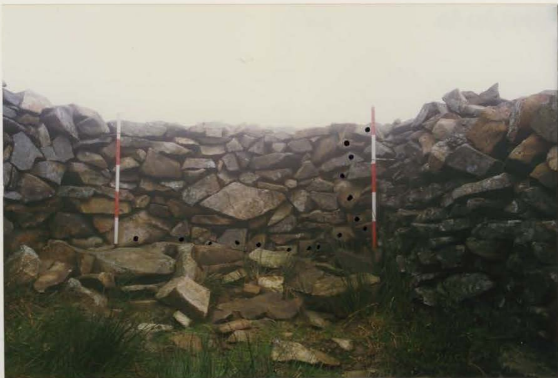
Plate 206 G1022/212/32 ; Collapse 9a after conservation.
