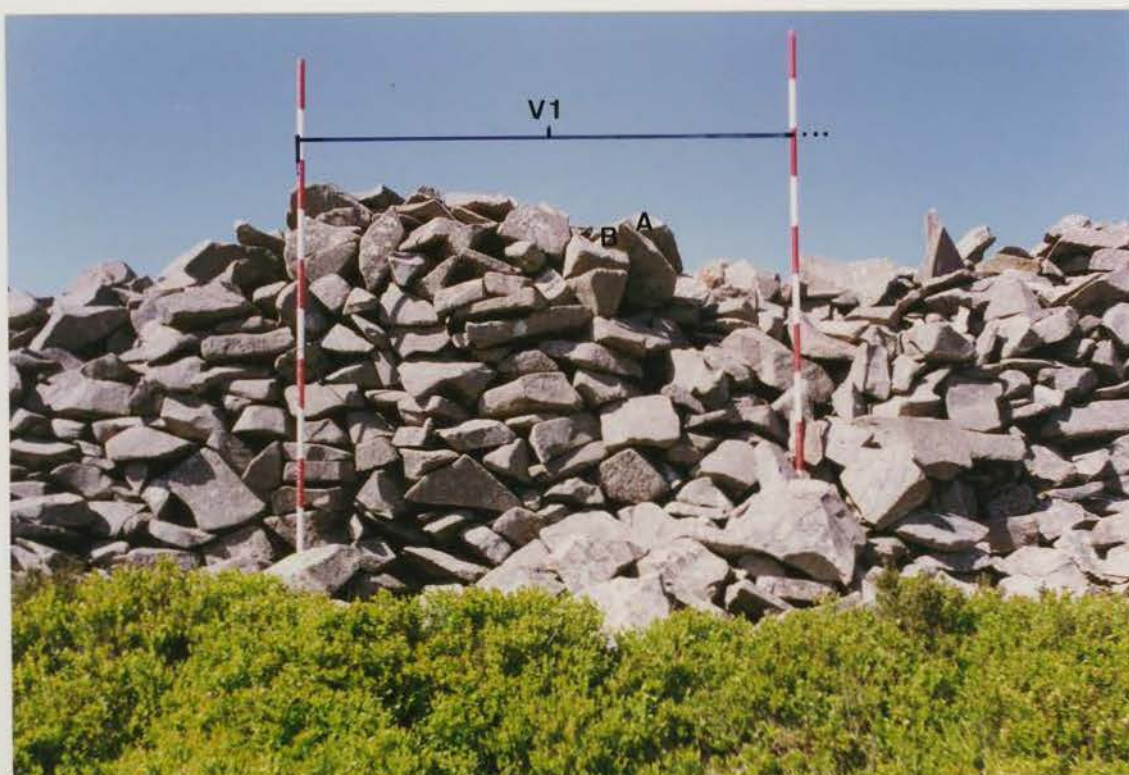
Plate 58 G1022/197/22 ; Collapse V1 before conservation.
