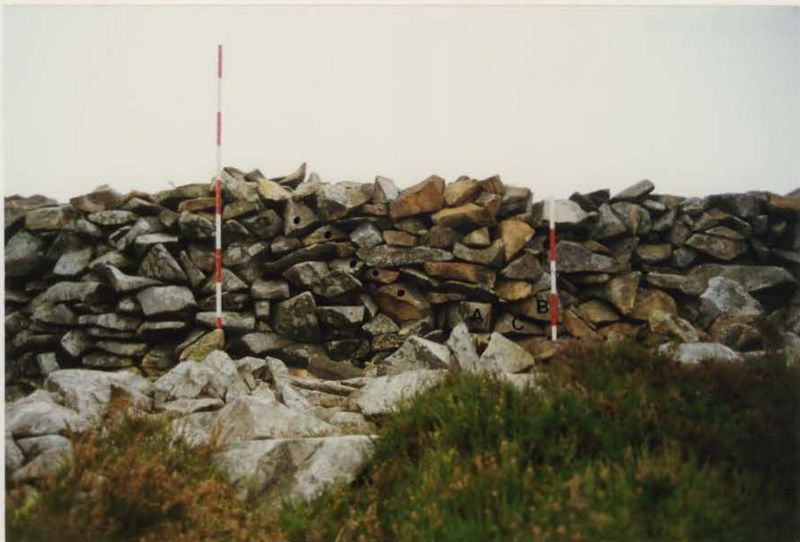
Plate 137 G1022/210/26 ; Collapse X4 after conservation.
