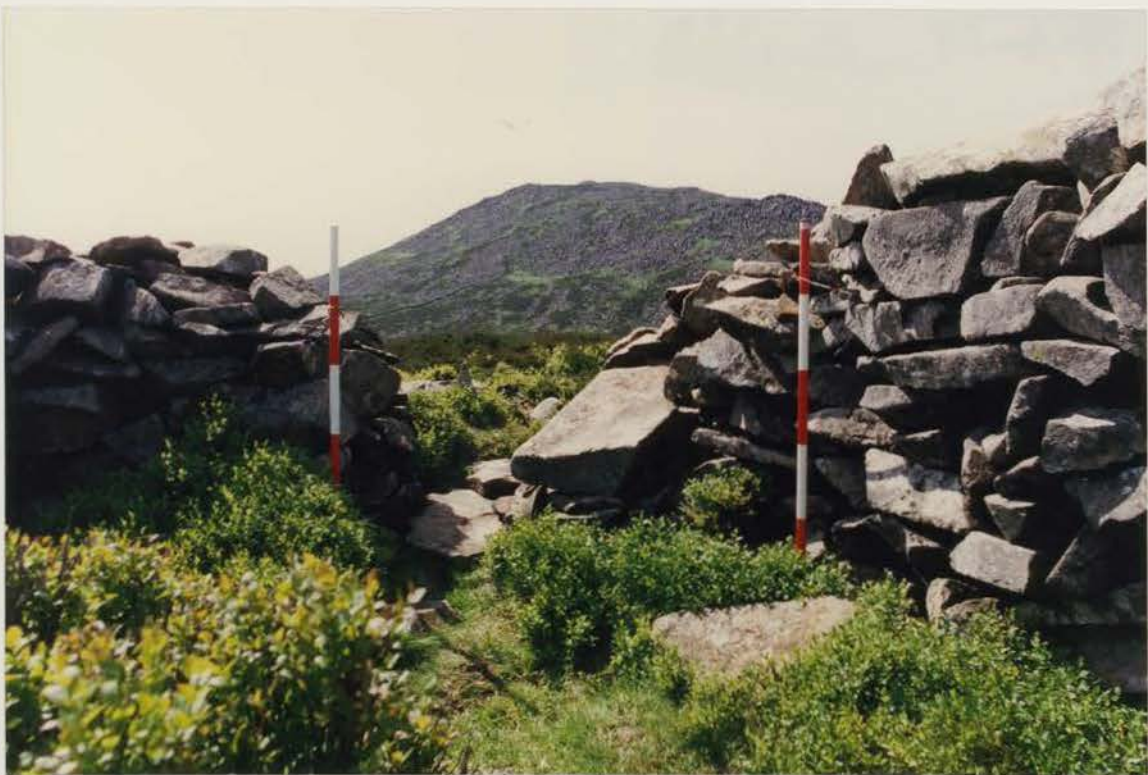
Plate 222 G1022/201/19 ; Collapse 10a before conservation.
