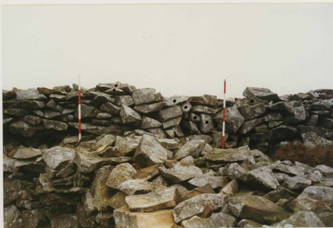
Plate 144 G1022/210/34 ; Collapse X7 after conservation.
