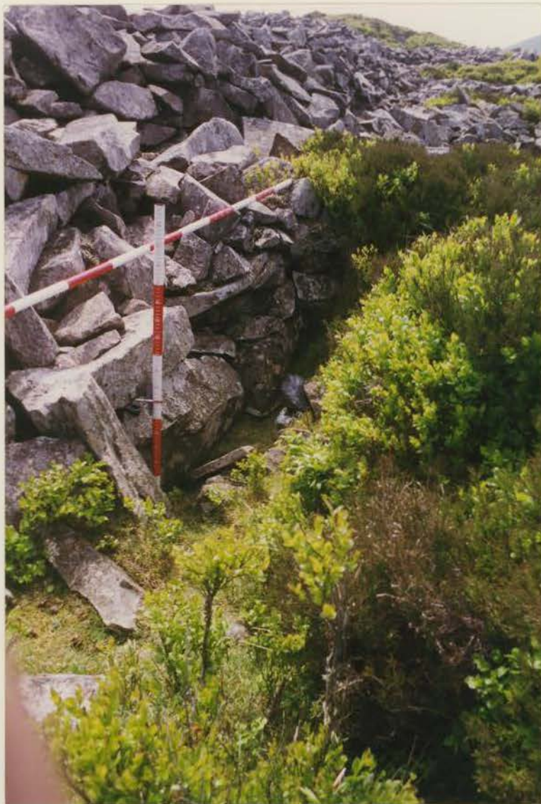
Plate 158 G1022/199/12; Collapse 45Ad before conservation.
