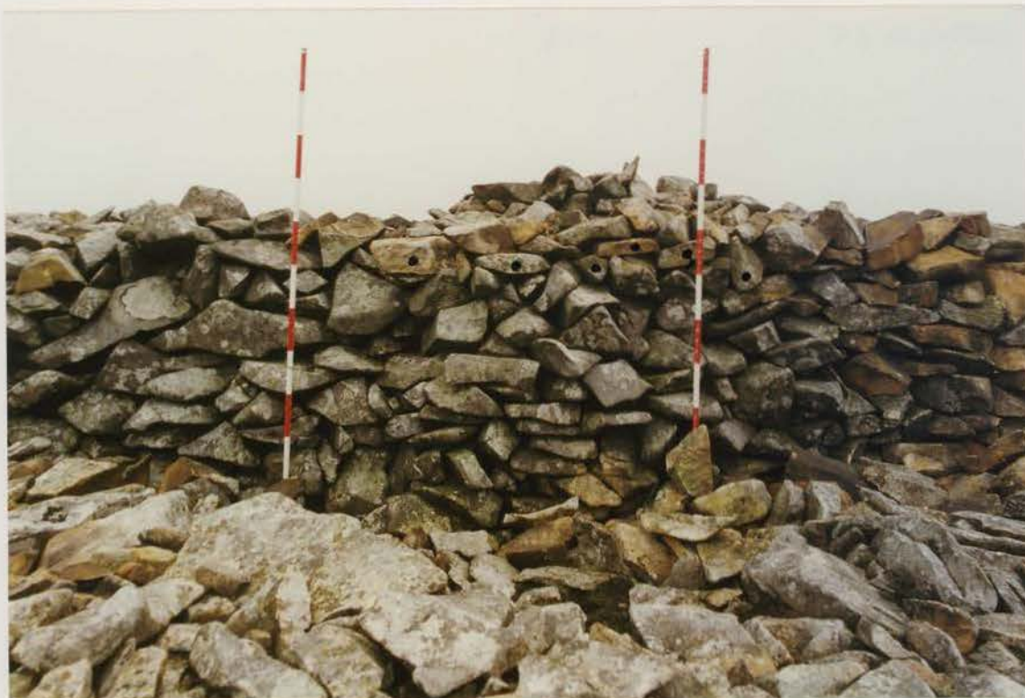
Plate 133 G1022/210/24 ; Collapse X3 after conservation.
