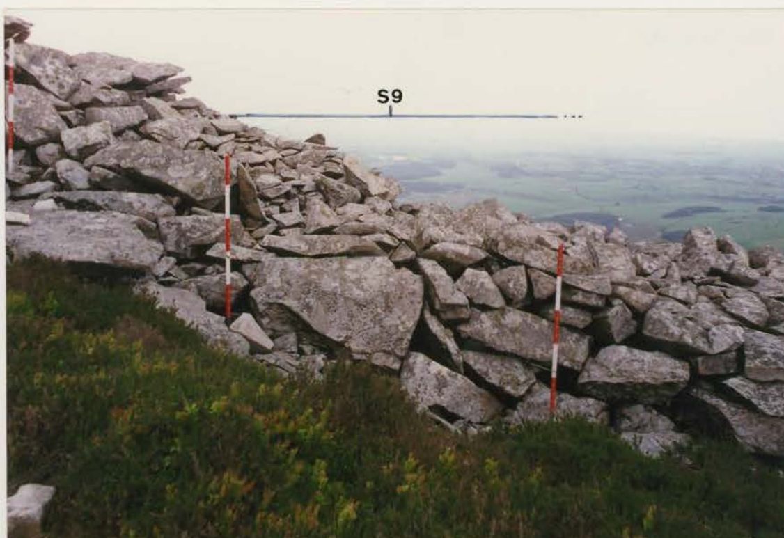
Plate 22 G1022/194/13 ; Collapse S9 before conservation.
