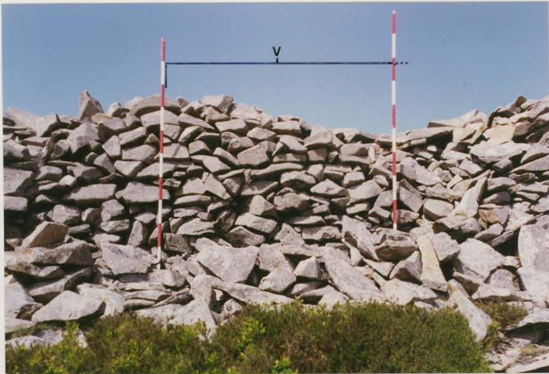
Plate 53 G1022/197/17 ; Collapse V before conservation.
