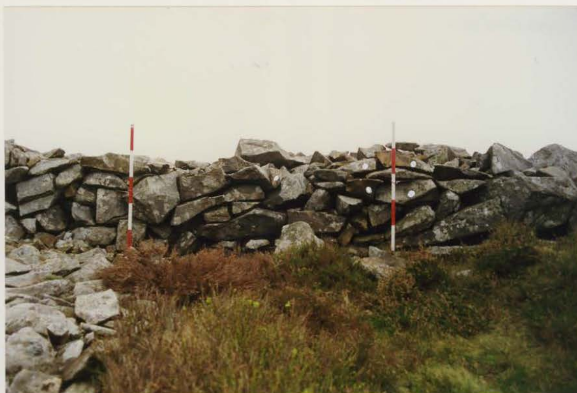
Plate 146 G1022/210/36 ; Collapse X8 after conservation.
