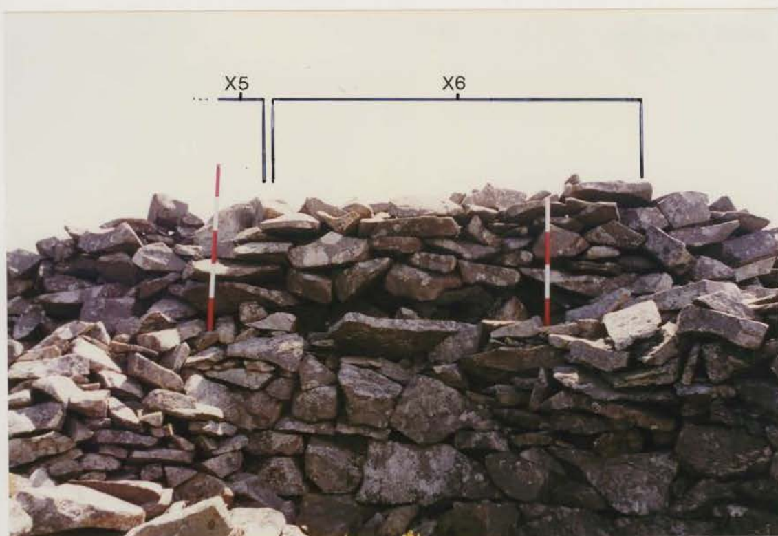
Plate 140 G1022/196/25 ; Collapse X6 before conservation.
