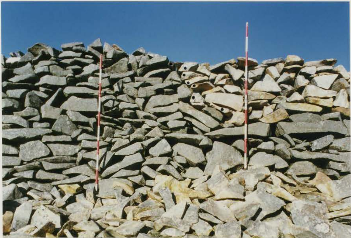
Plate 83 G1022/211/12 ; Collapse X after conservation.
