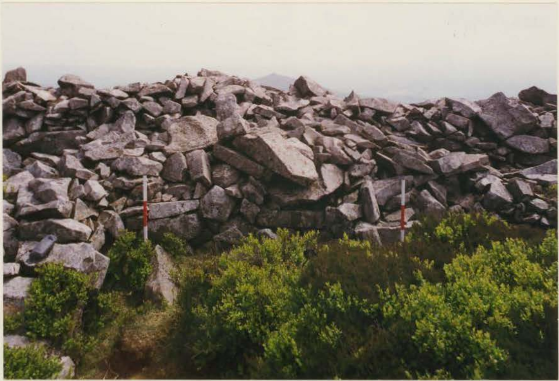
Plate 157 G1022/199/10; Collapse 45Ad before conservation.
