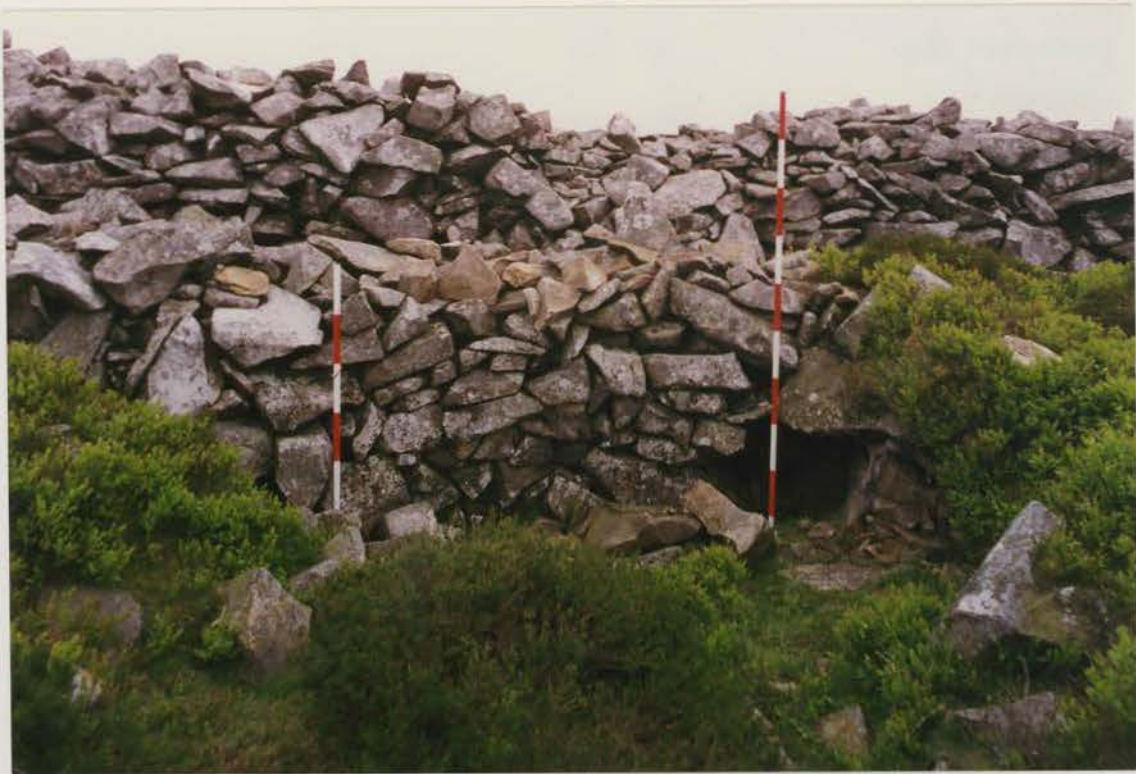
Plate 167 G1022/199/24 ; Collapses 107a and 107d before conservation.
