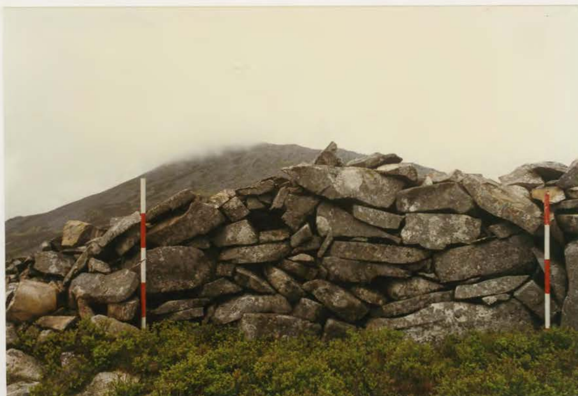
Plate 106. G1022\221\02, collapse 19a before conservation.
