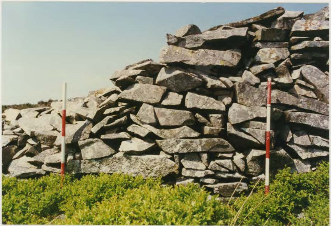
Plate 257. G1022\227\09, collapse 13a before conservation.
