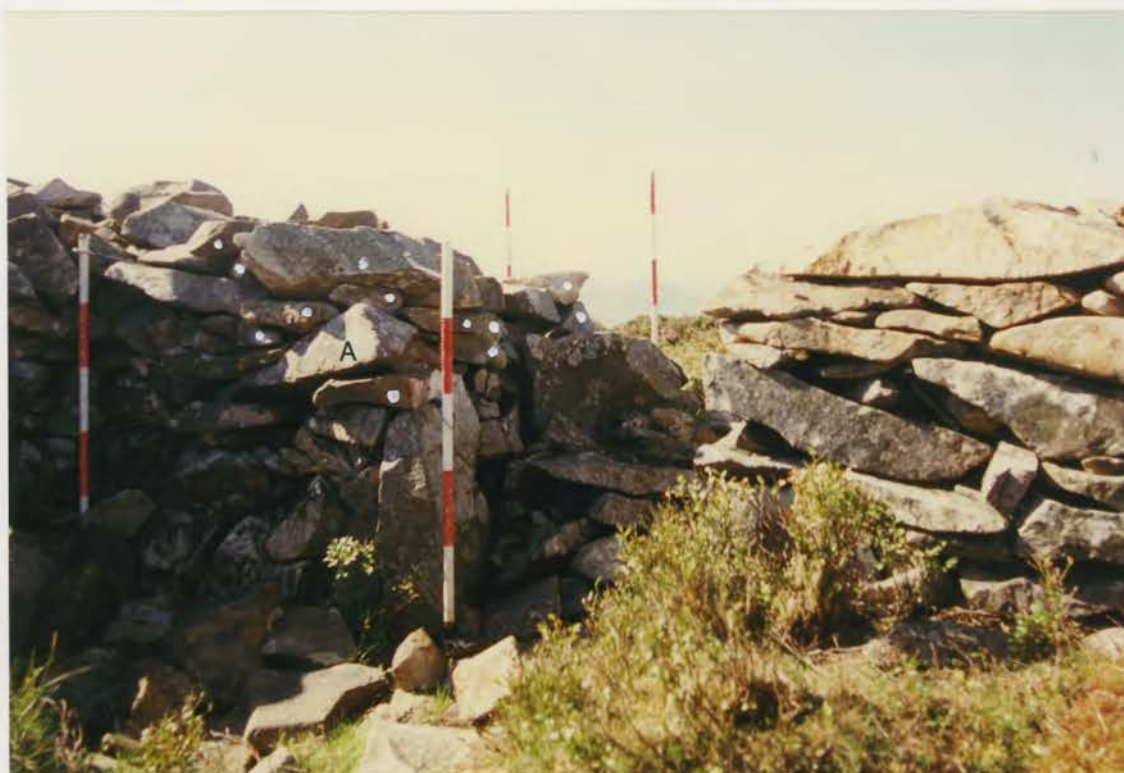
Plate 201. G1022\246\08, collapse 8i after conservation.
