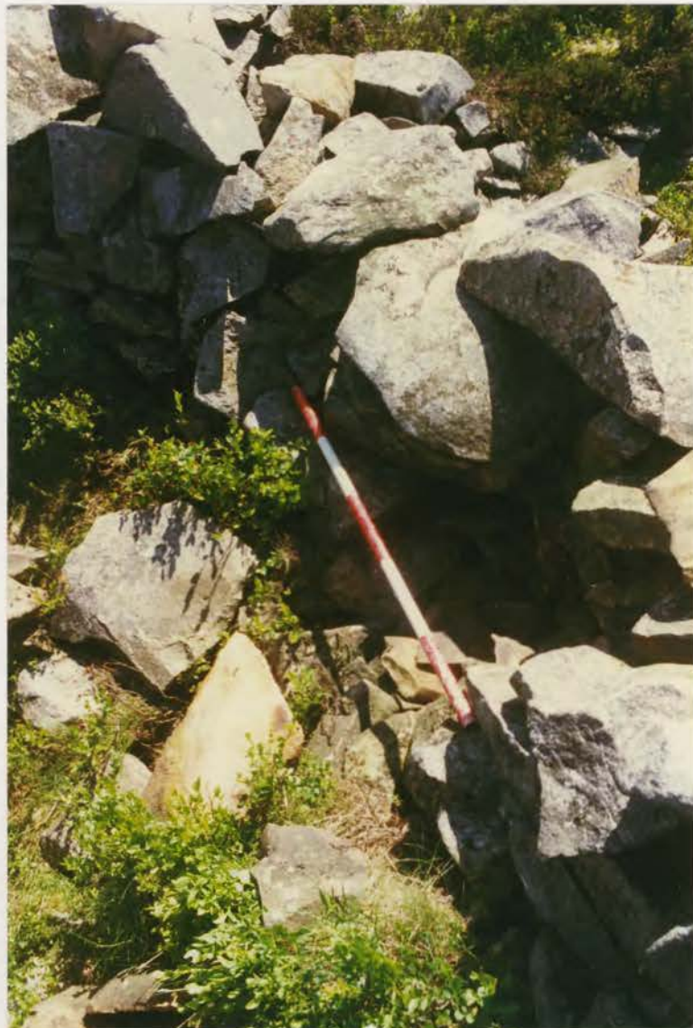
Plate 164. G1022\236\12, collapse 16b after clearance.
