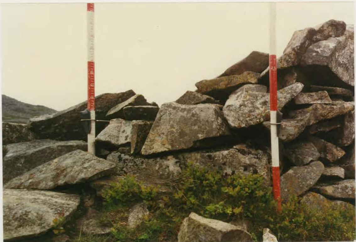
Plate 214. G1022\225\22, collapse 7a before conservation.
