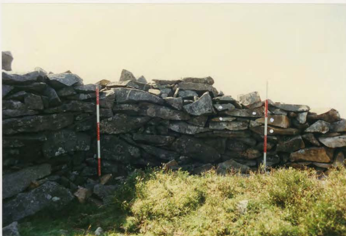
Plate 175. G1022\245\6A, collapse 15b after conservation.
