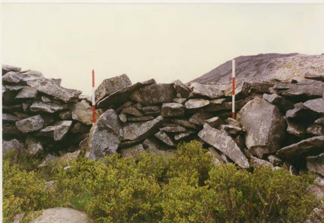
Plate 49. G1022\216\24, collapse 26b before conservation.
