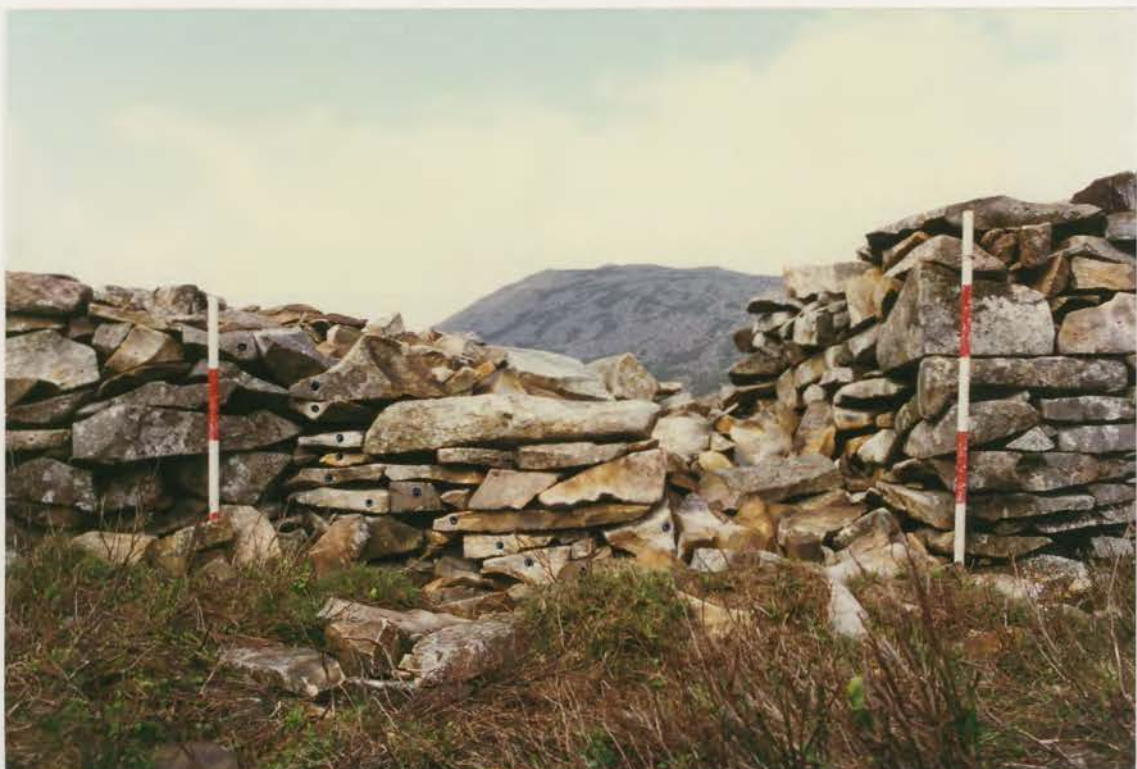
Plate 70. G1022\243\21, collapse 23i after conservation.
