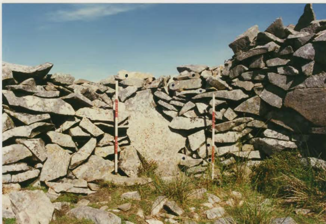
Plate 220. G1022\246\18, collapse 7c after conservation.
