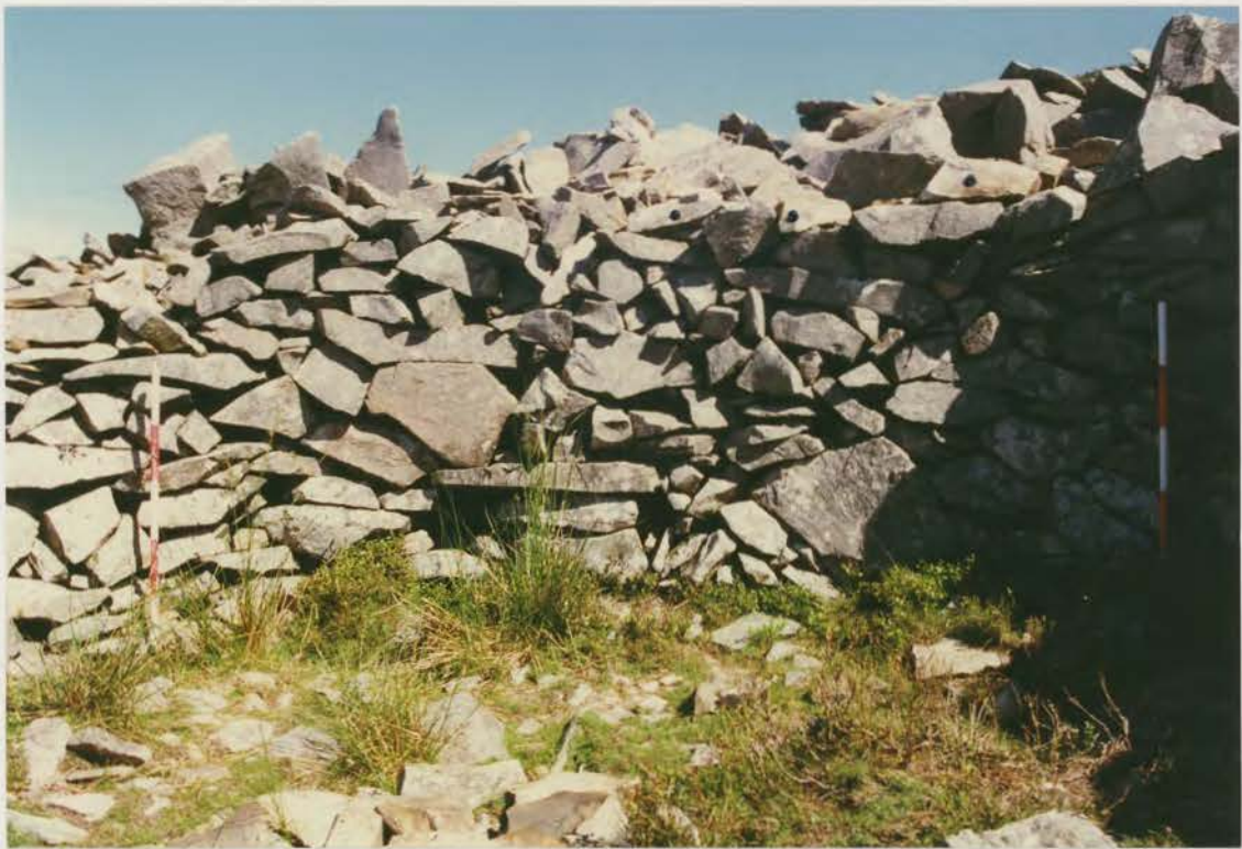
Plate 221. G1022\246\20, collapse 7c after conservation.
