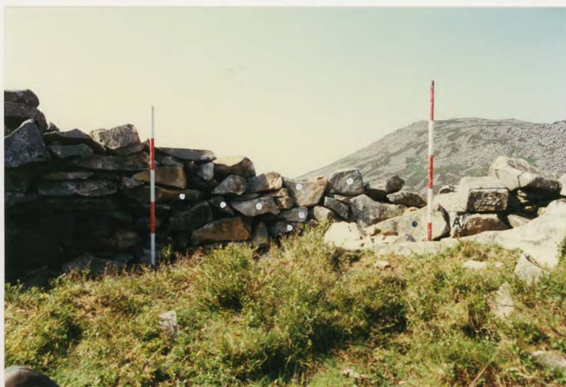
Plate 176. G1022\245\8A, collapse 15b after conservation.
