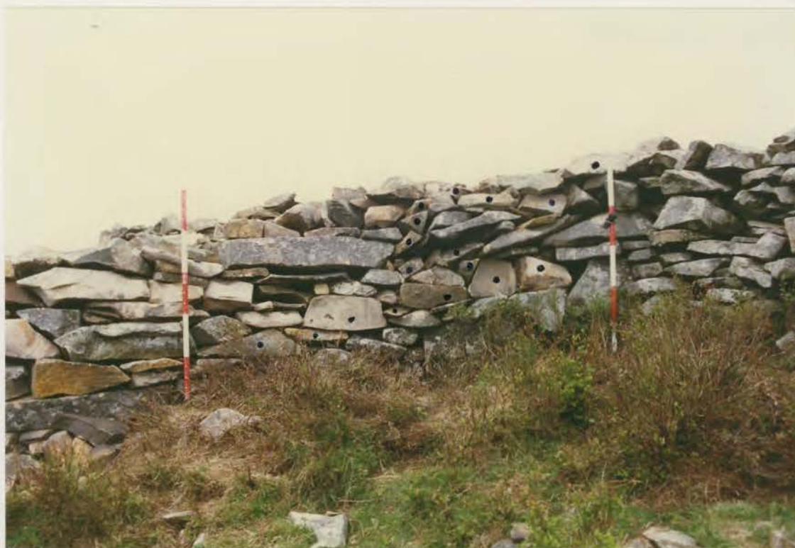
Plate 299. G1022\248\25, collapse 5c after conservation.
