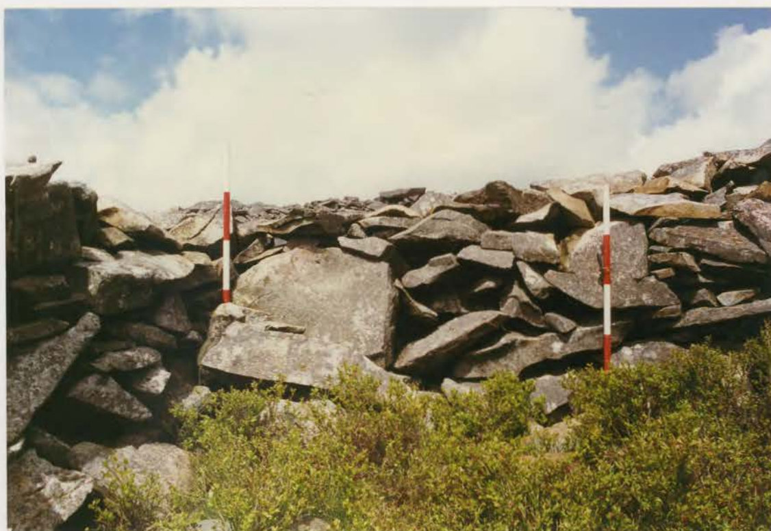
Plate 50. G1022\216\19, collapse 26b before conservation.
