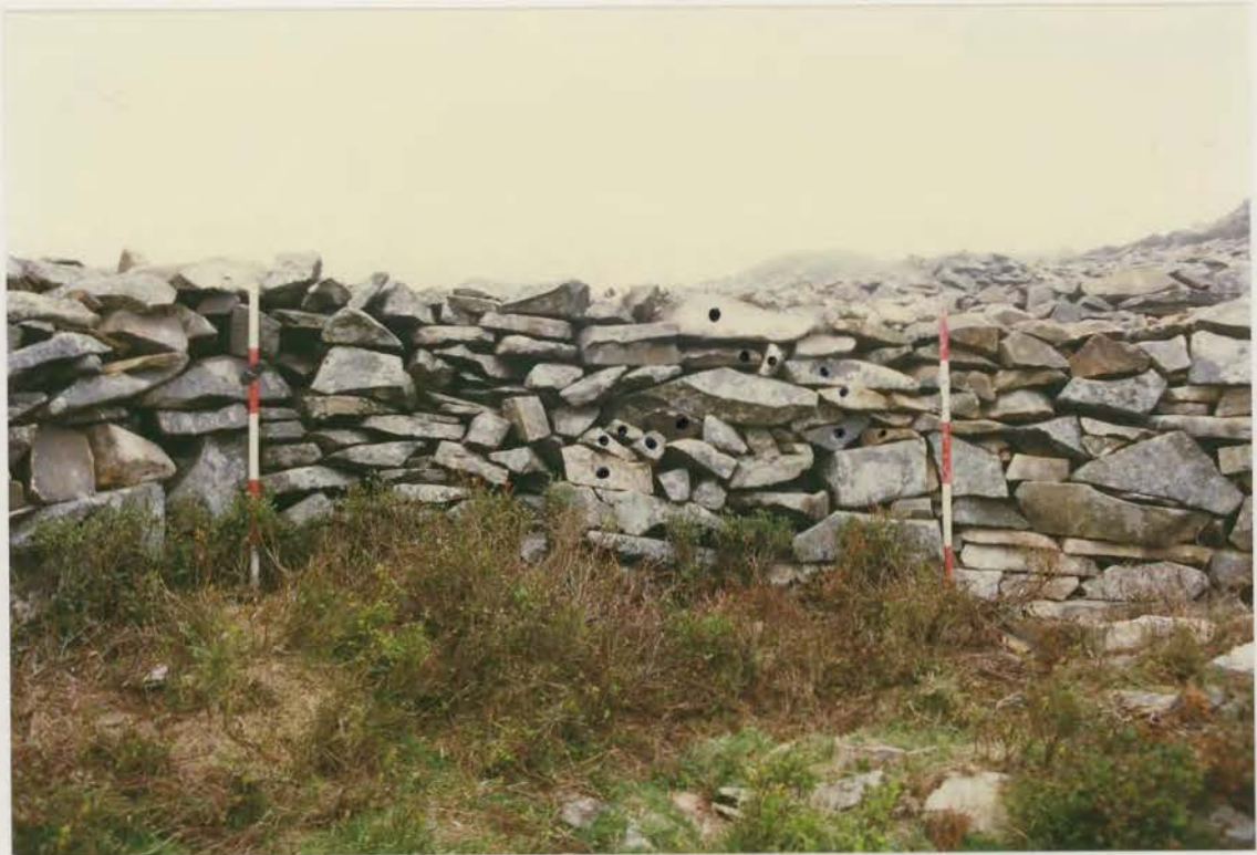
Plate 301. G1022\248\27, collapse 5c after conservation.
