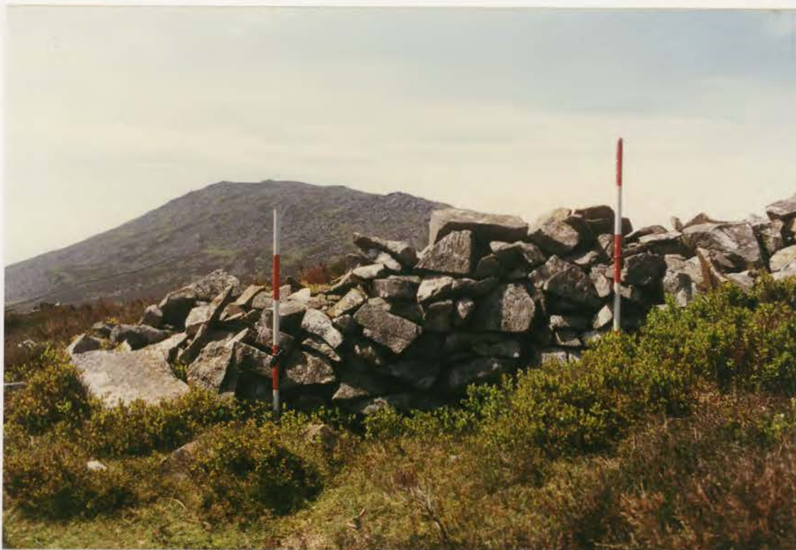
Plate 153. G1022\222\23, collapse 95a before conservation.
