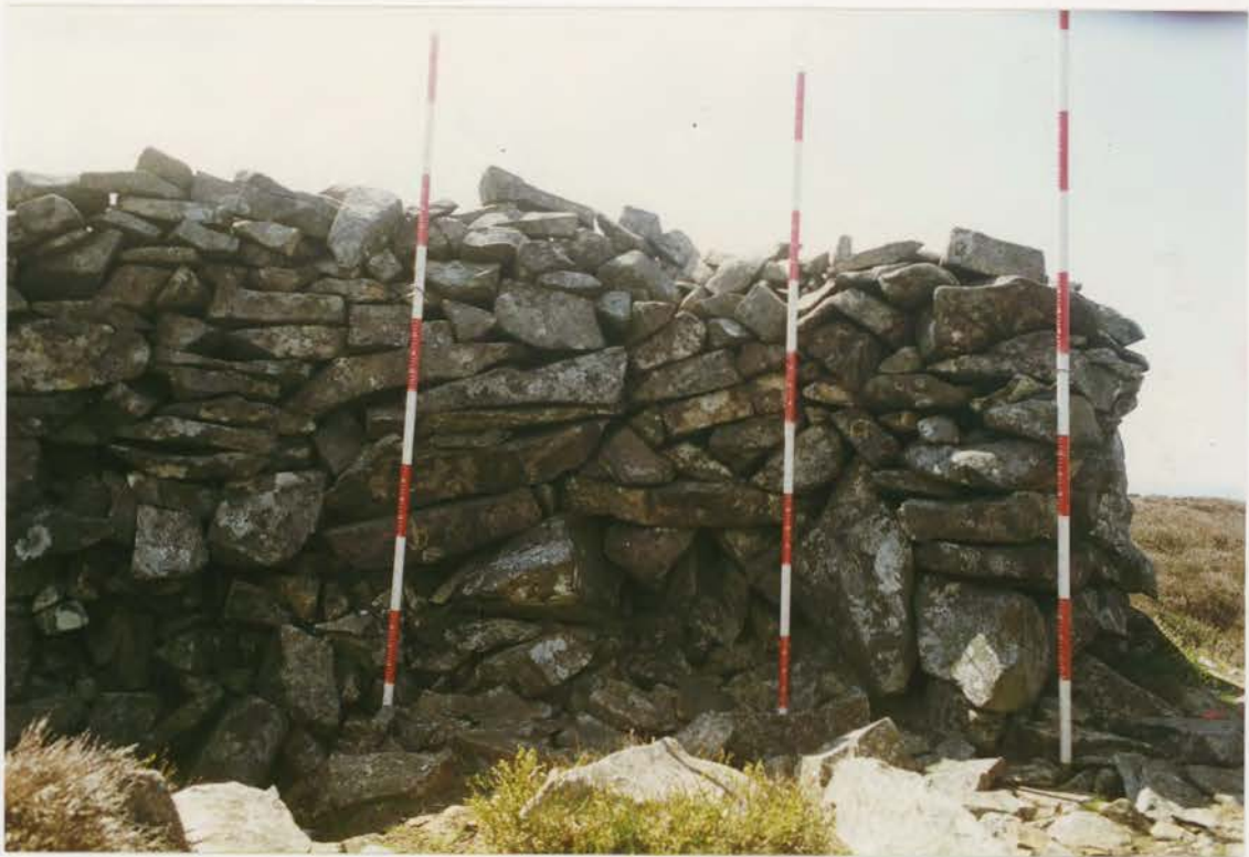
Plate 13. G1022\215\00, collapse 24b before conservation.
