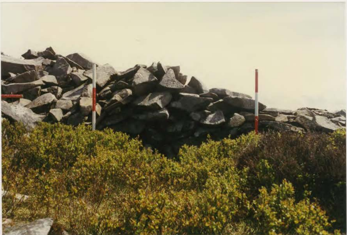
Plate 92. G1022\220\04, collapse 21d before conservation.
