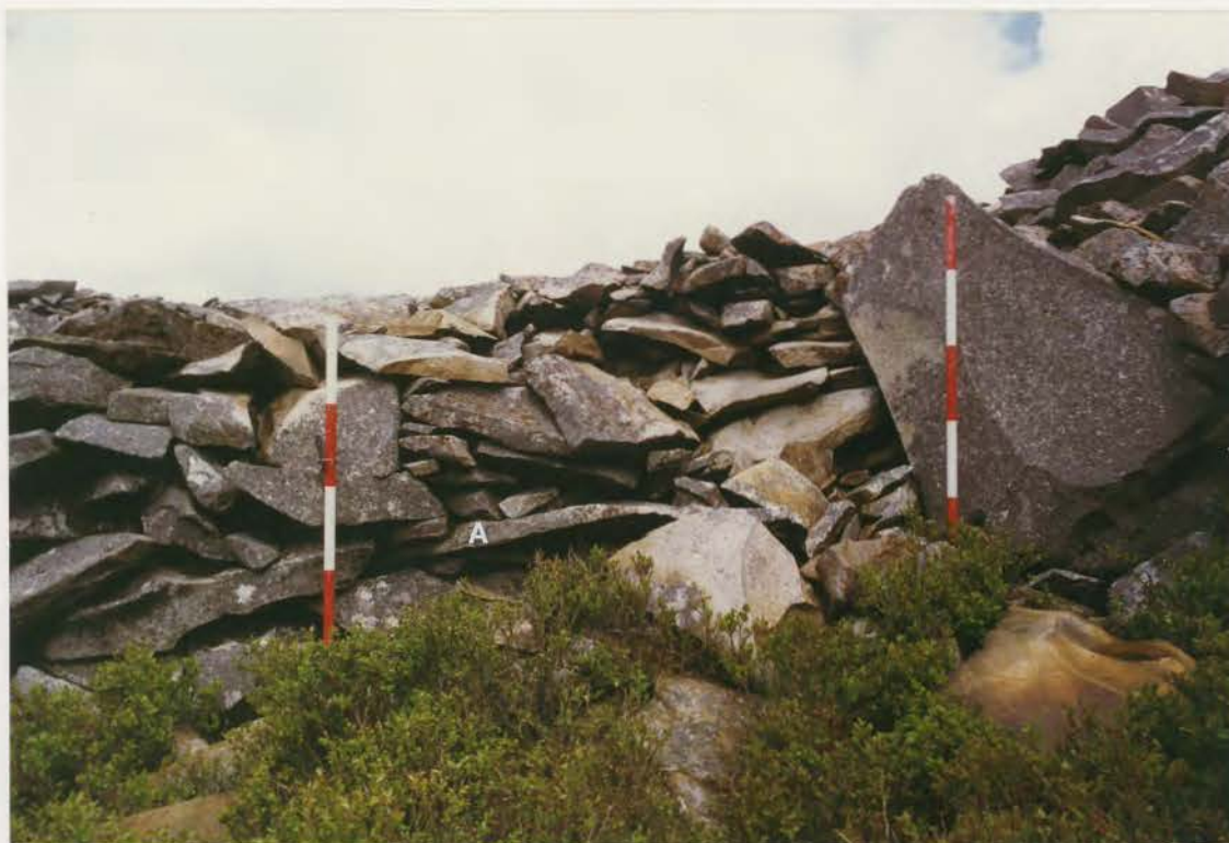
Plate 33. G1022\216\17, collapse 26a before conservation.
