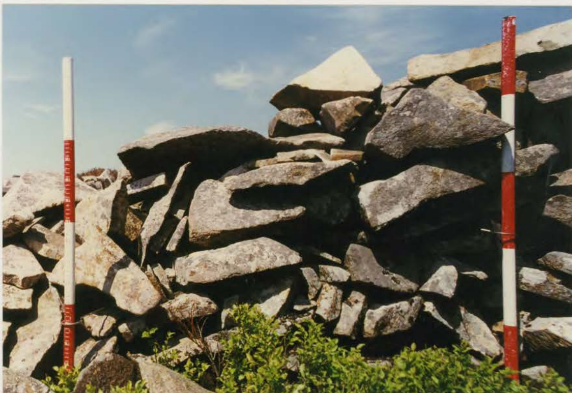
Plate 247. G1022\226\31, collapse 12a before conservation.
