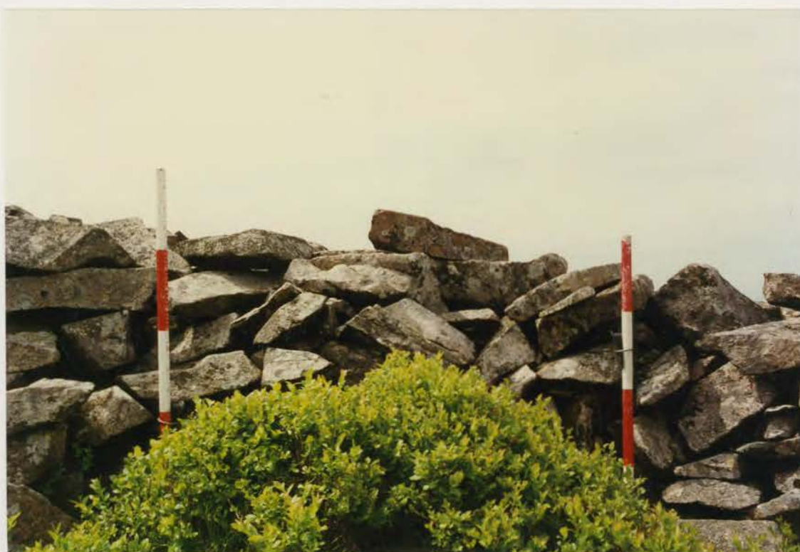
Plate 266. G1022\227\31, collapse 13d before conservation.
