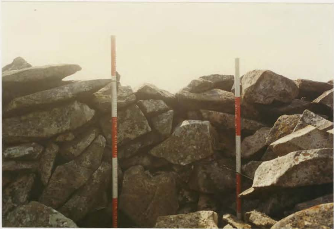
Plate 185. G1022\224\22, collapse 8b before conservation.
