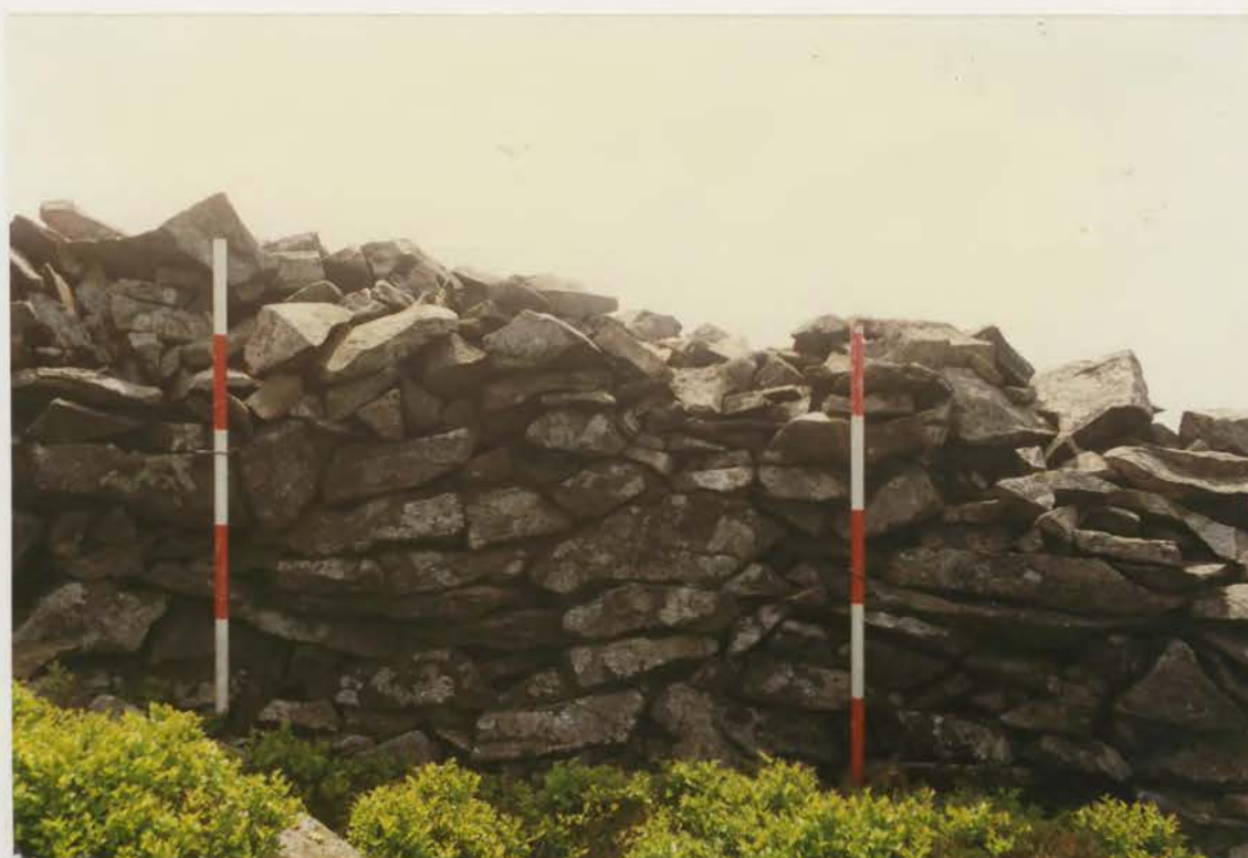
Plate 274. G1022\228\27, collapse 14b before conservation.
