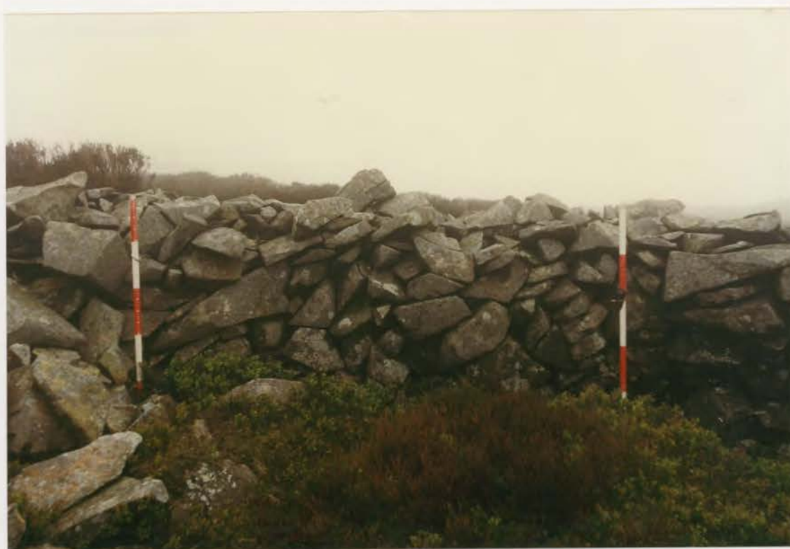
Plate 148. G1022\222\14, collapse 17d before conservation.
