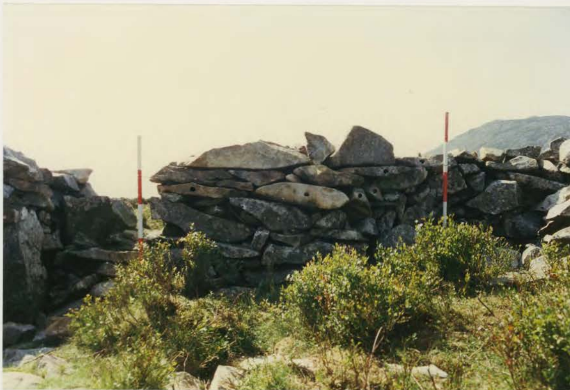
Plate 207. G1022\245\28A, collapse 8a after conservation.
