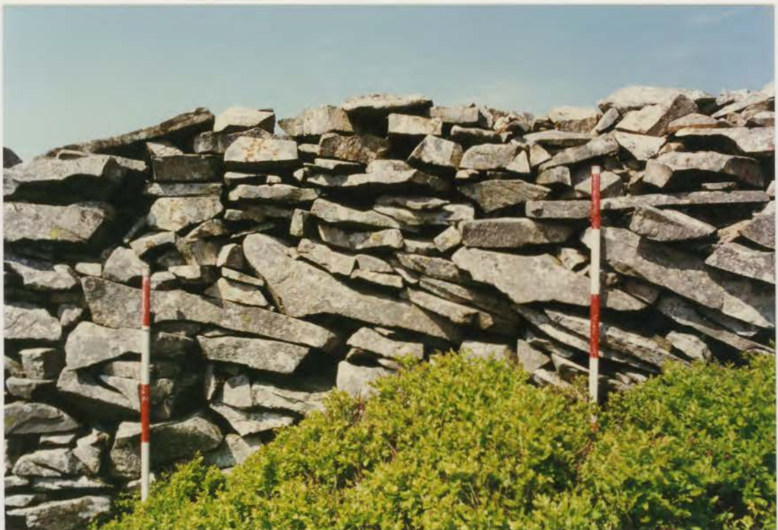
Plate 258. G1022\227\11, collapse 13a before conservation.
