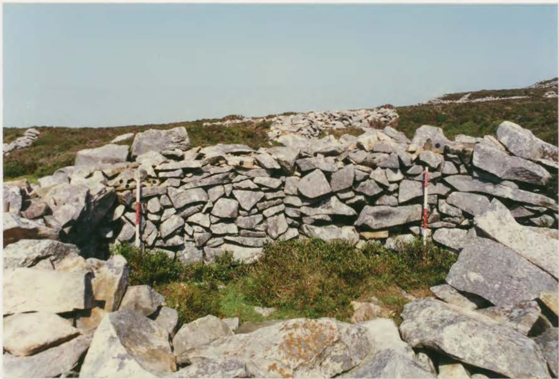
Plate 167. G1022\245\16A, collapse 16d after conservation.
