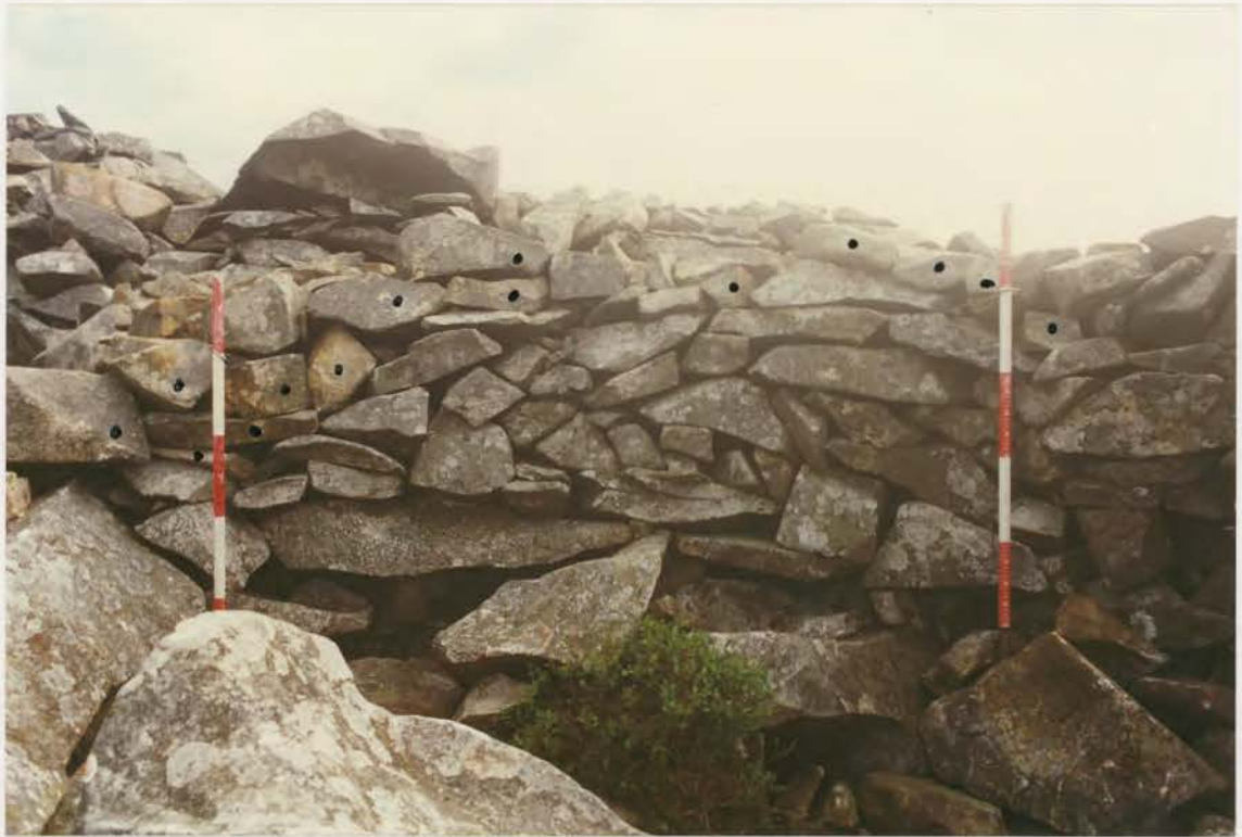
Plate 11. G1022\242\08, collapse 24c after conservation.
