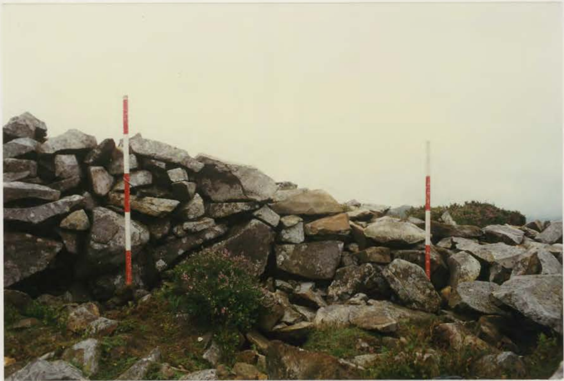
Plate 419. G1022\240\25, collapse 90d before conservation.
