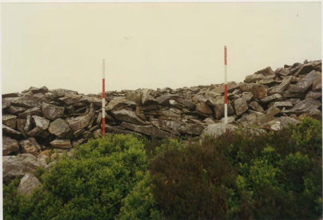
Plate 328. G1022\230\24A, collapse 6e before conservation.
