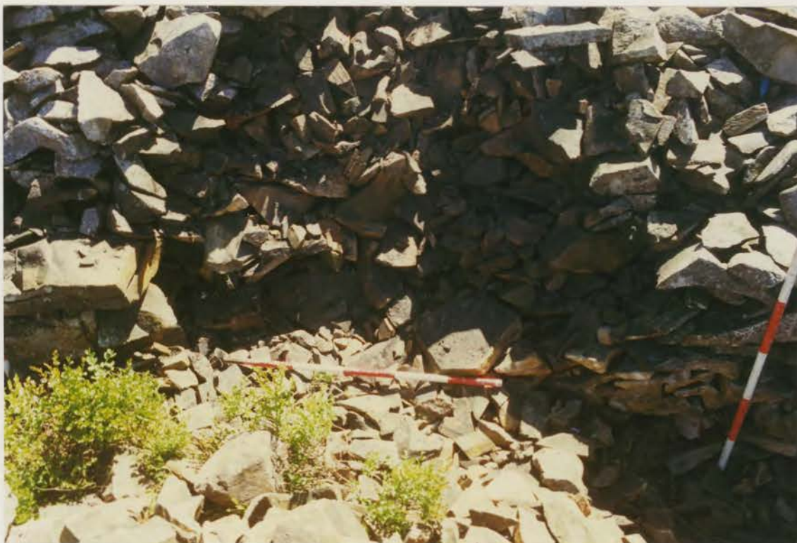
Plate 305. G1022\238\13, collapse 5e after clearance.
