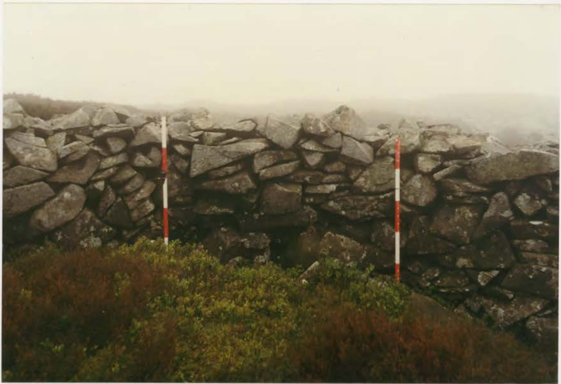
Plate 149. G1022\222\16, collapse 17d before conservation.
