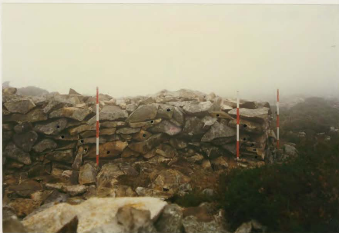
Plate 347. G1022\249\25, collapse 6l after conservation.
