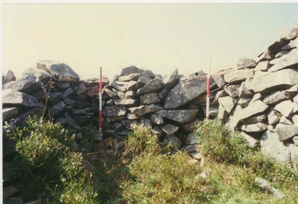
Plate 166. G1022\245\14A, collapse 16c after conservation.
