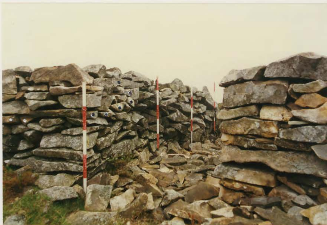
Plate 317. G1022\249\04, collapse 5i after conservation.
