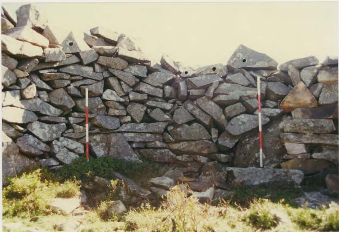
Plate 222. G1022\246\22, collapse 7c after conservation.
