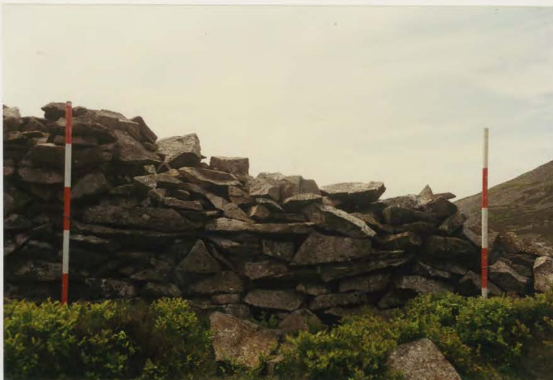
Plate 275. G1022\228\29, collapse 14b before conservation.
