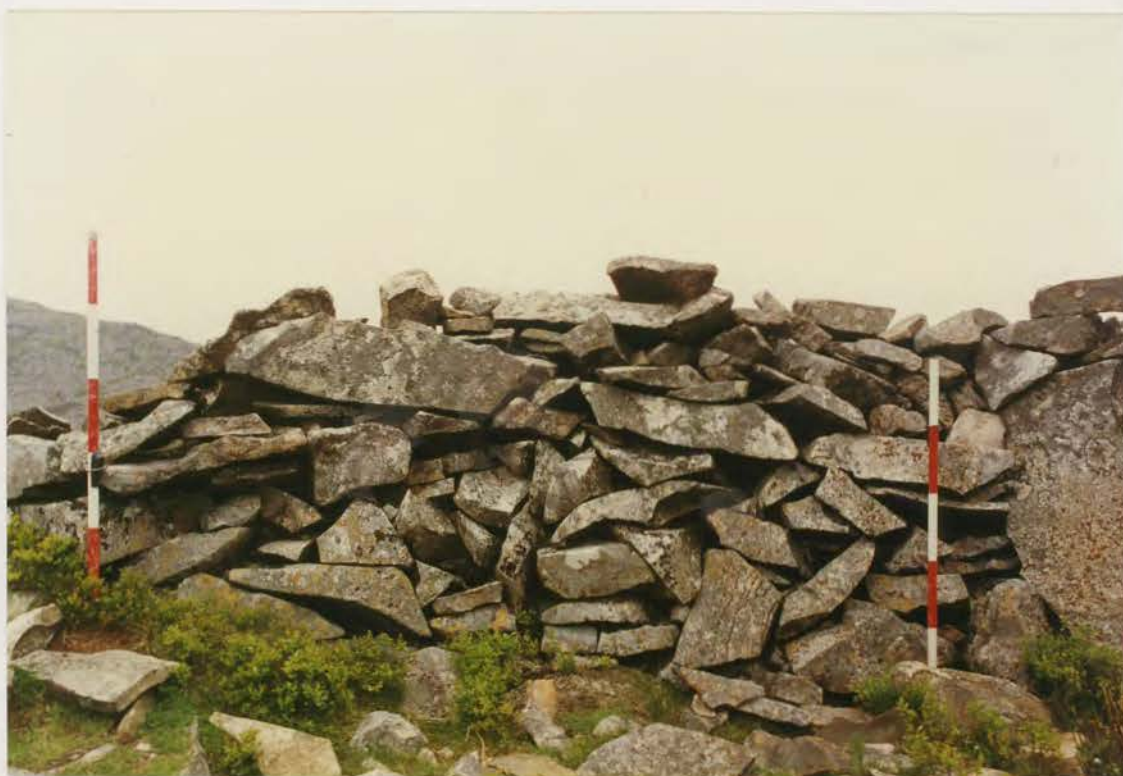
Plate 217. G1022\225\24, collapse 7b before conservation.
