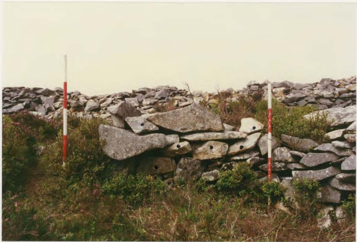
Plate 25. G1022\242\18, collapse 25c after conservation.
