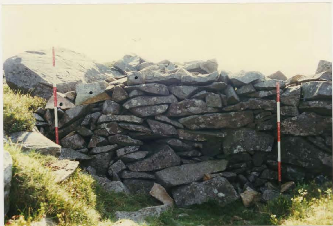
Plate 170. G1022\245\04A, collapse 15a after conservation.
