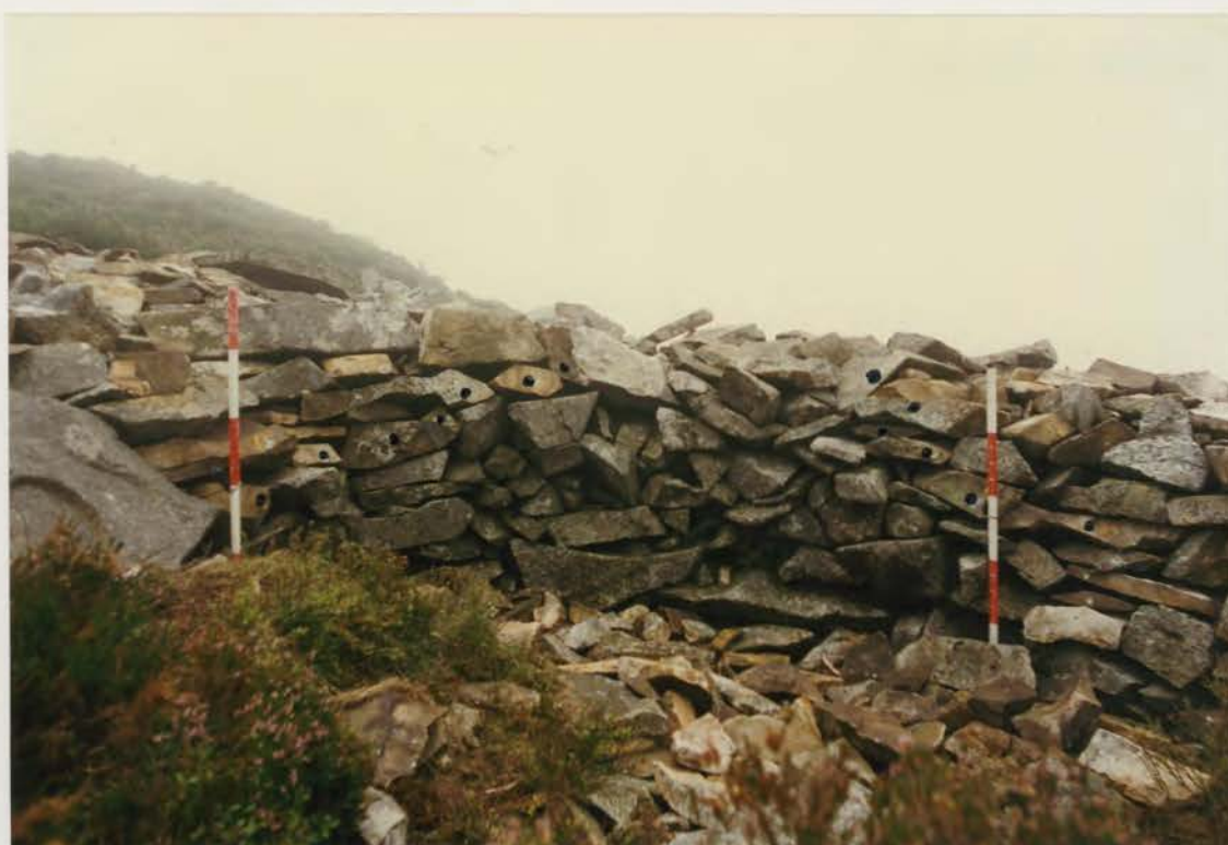
Plate 338. G1022\249\17, collapse 6j after conservation.
