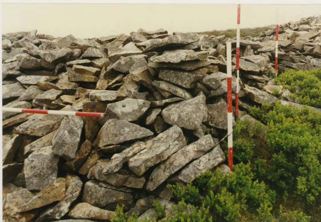
Plate 320. G1022\230\17A, collapse 6b before conservation.
