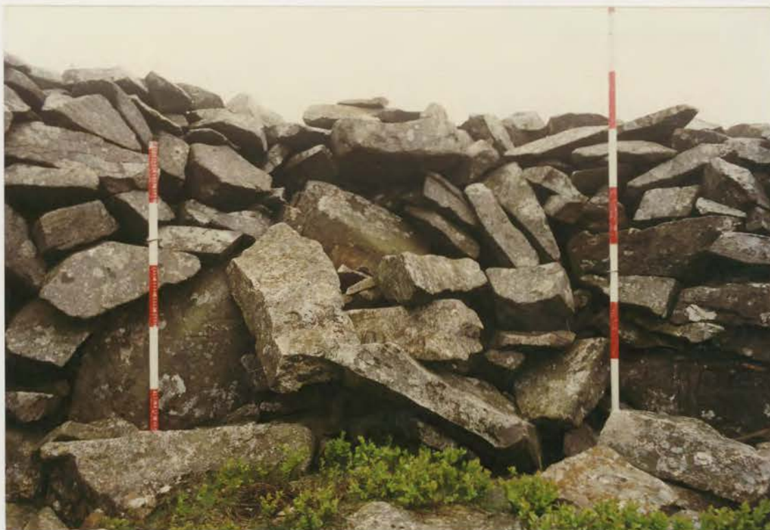
Plate 223. G1022\226\01, collapse 7d before conservation.
