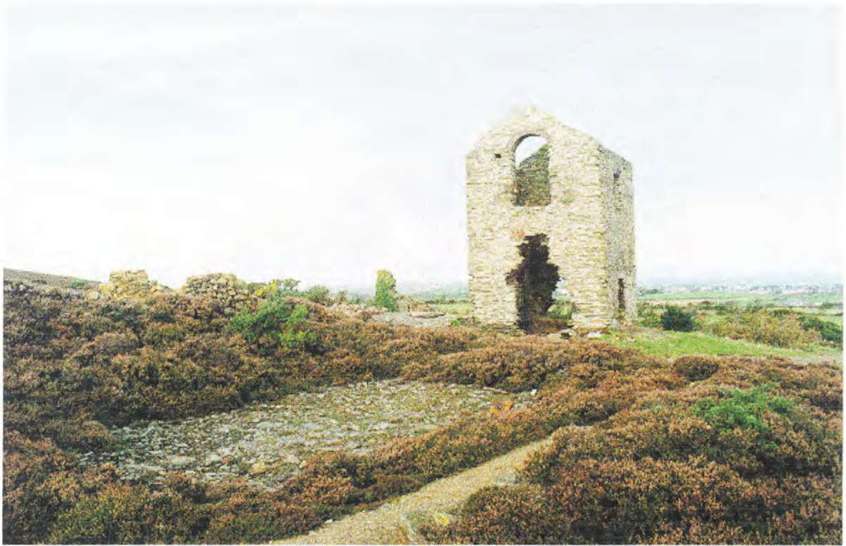
5 The Pearl engine house of 1818/19 (feature no. 122) is a Scheduled Ancient Monument -
