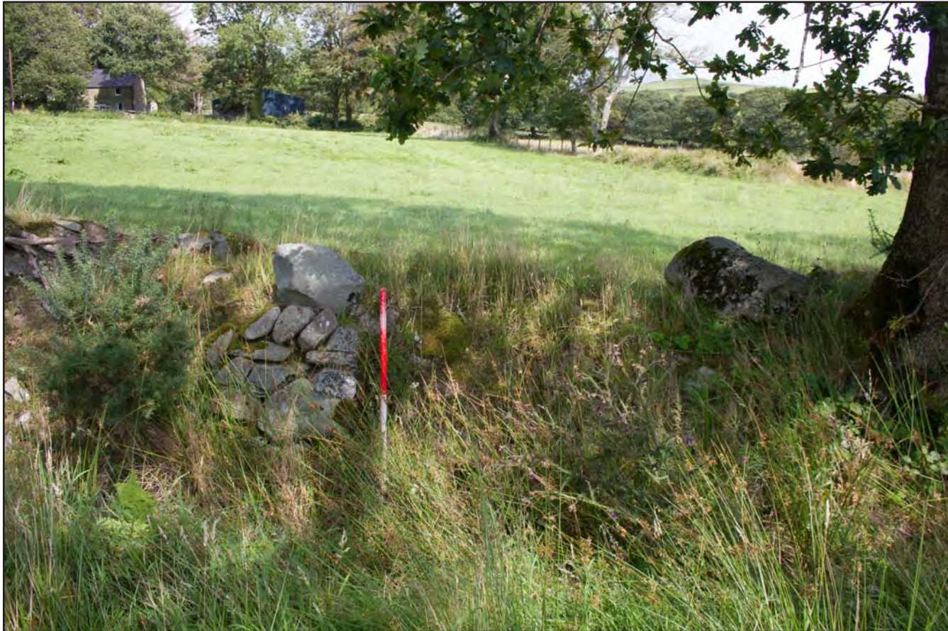
Plate 16: Clawdd boundary wall- field 6 (feature 4 / GAT PRN 81351), from the southwest. Scale 1.0m.
