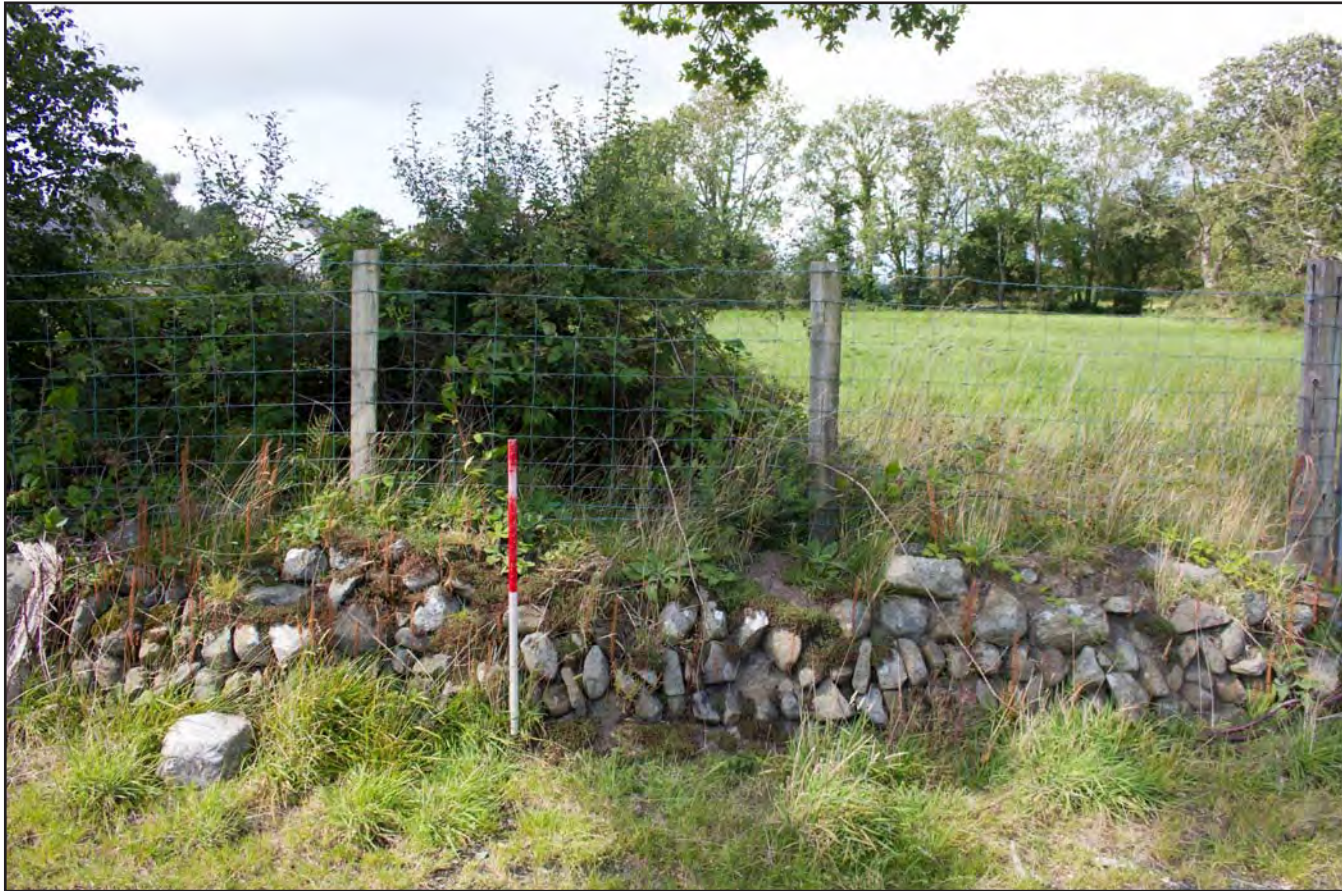
Plate 17: Clawdd boundary wall- fields 5 and 6 (feature 5 / GAT PRN 81352), from the southeast. Scale 1.0m.
