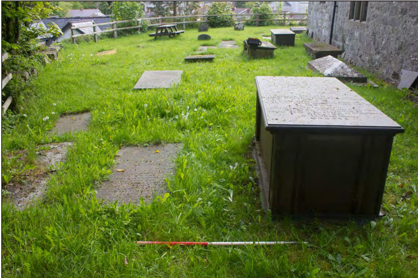
Plate 35: Pre excavation shot of drainage route for septic tank to soakaway (west) , at St. Mary's Church, Church Street, Llanfair Talhaiarn, Conwy - from the west - 1.00m scale
