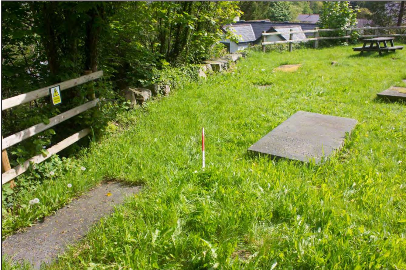
Plate 36: Pre excavation shot of drainage route for septic tank to soakaway (east) , at St. Mary's Church, Church Street, Llanfair Talhaiarn, Conwy - from the southwest - 1.00m scale
