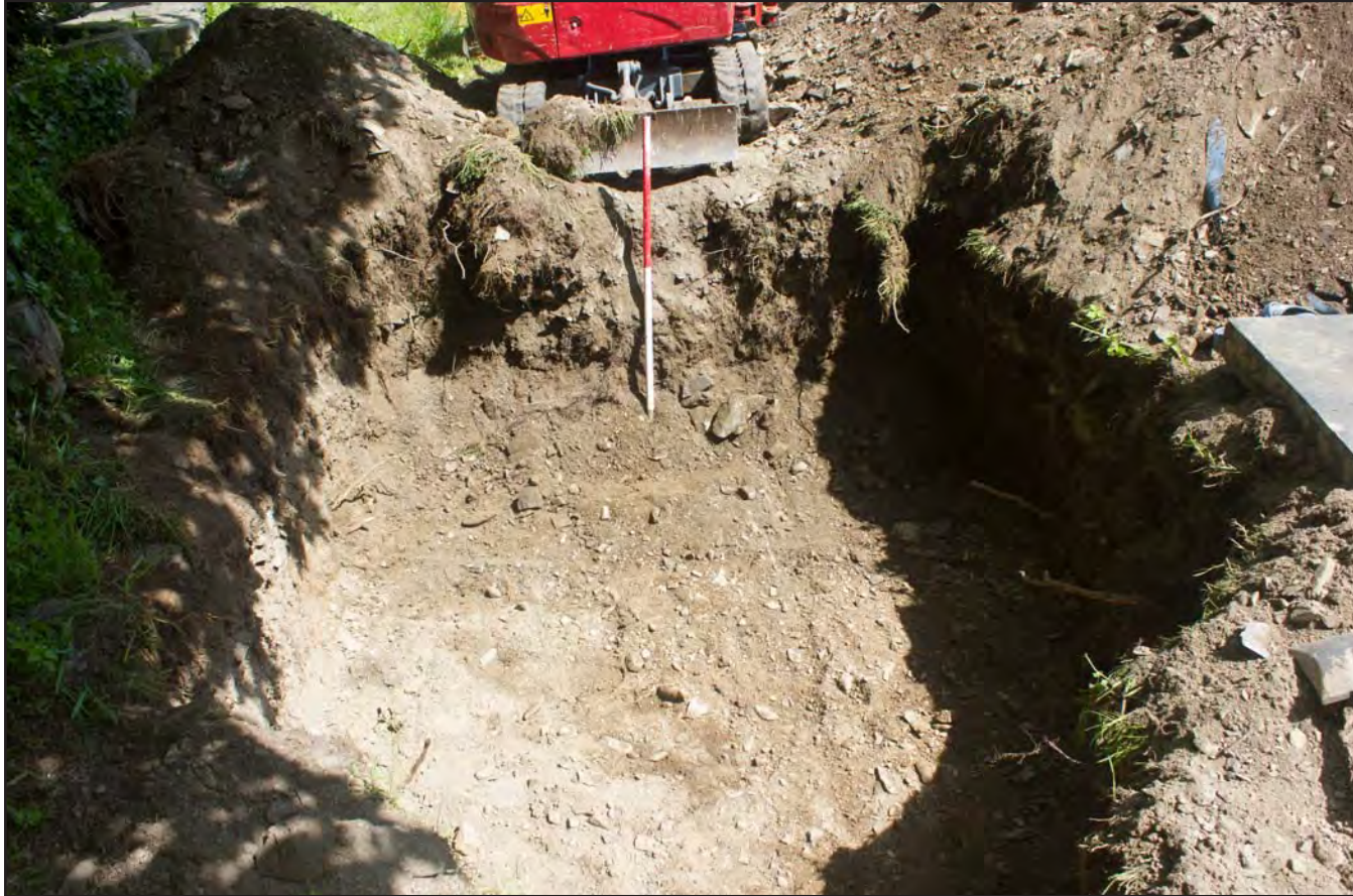
Plate 45: Post excavation shot of soakaway for septic tank, at St. Mary's Church, Church Street, Llanfair Talhaiarn, Conwy - from the west - 1.00m scale
