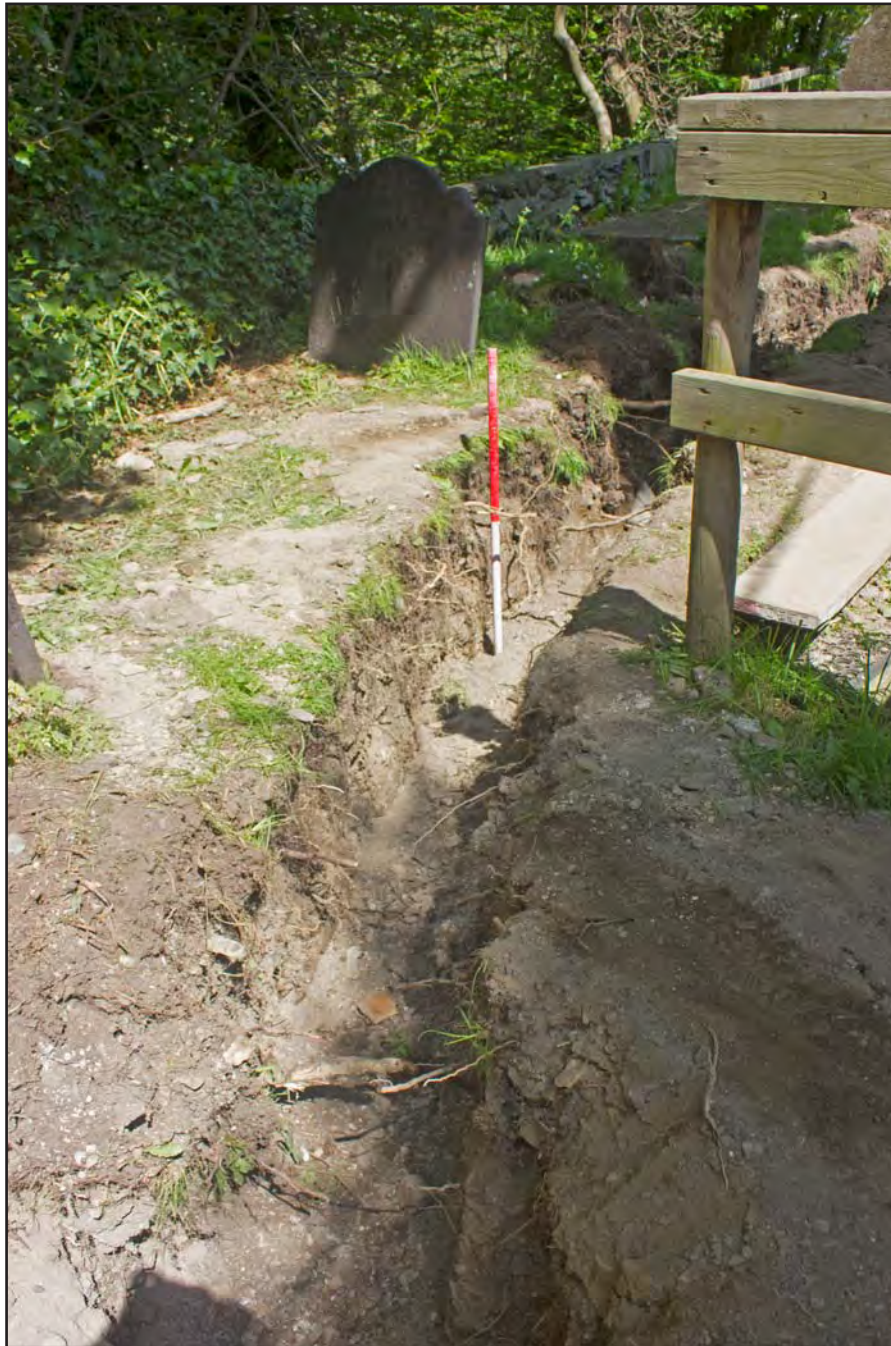
Plate 41: Post excavation shot of drainage route for septic tank to soakaway (west) , at St. Mary's Church, Church Street, Llanfair Talhaiarn, Conwy - from the southwest - 1.00m scale
