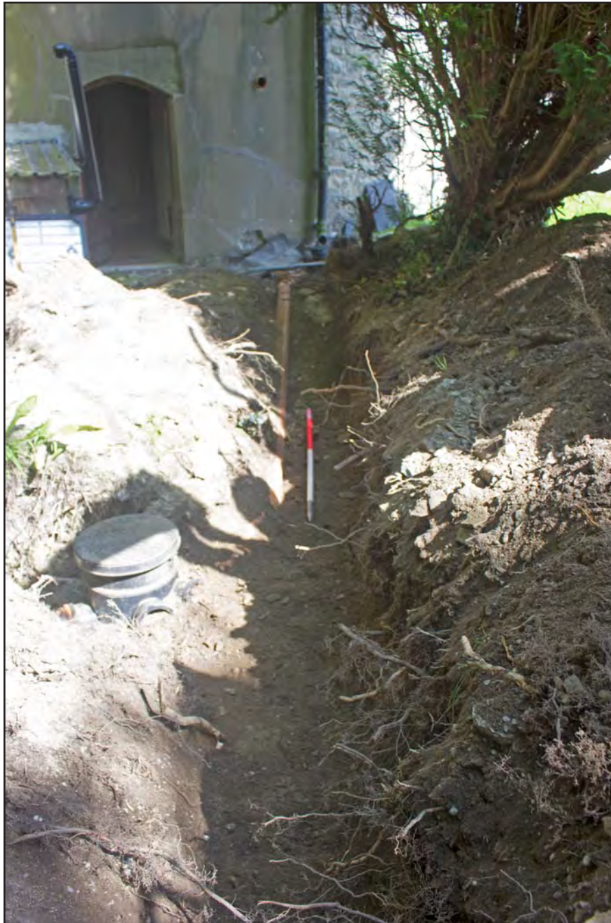
Plate 47: Post excavation shot of surface water drainage route, at St. Mary's Church, Church Street, Llanfair Talhaiarn, Conwy - from the northwest - 1.00m scale
