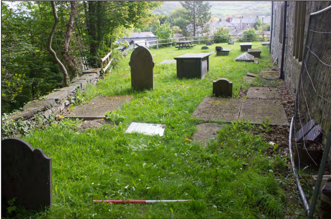
Plate 34: Pre excavation shot of drainage route for septic tank to soakaway (west) , at St. Mary's Church, Church Street, Llanfair Talhaiarn, Conwy - from the west - 1.00m
