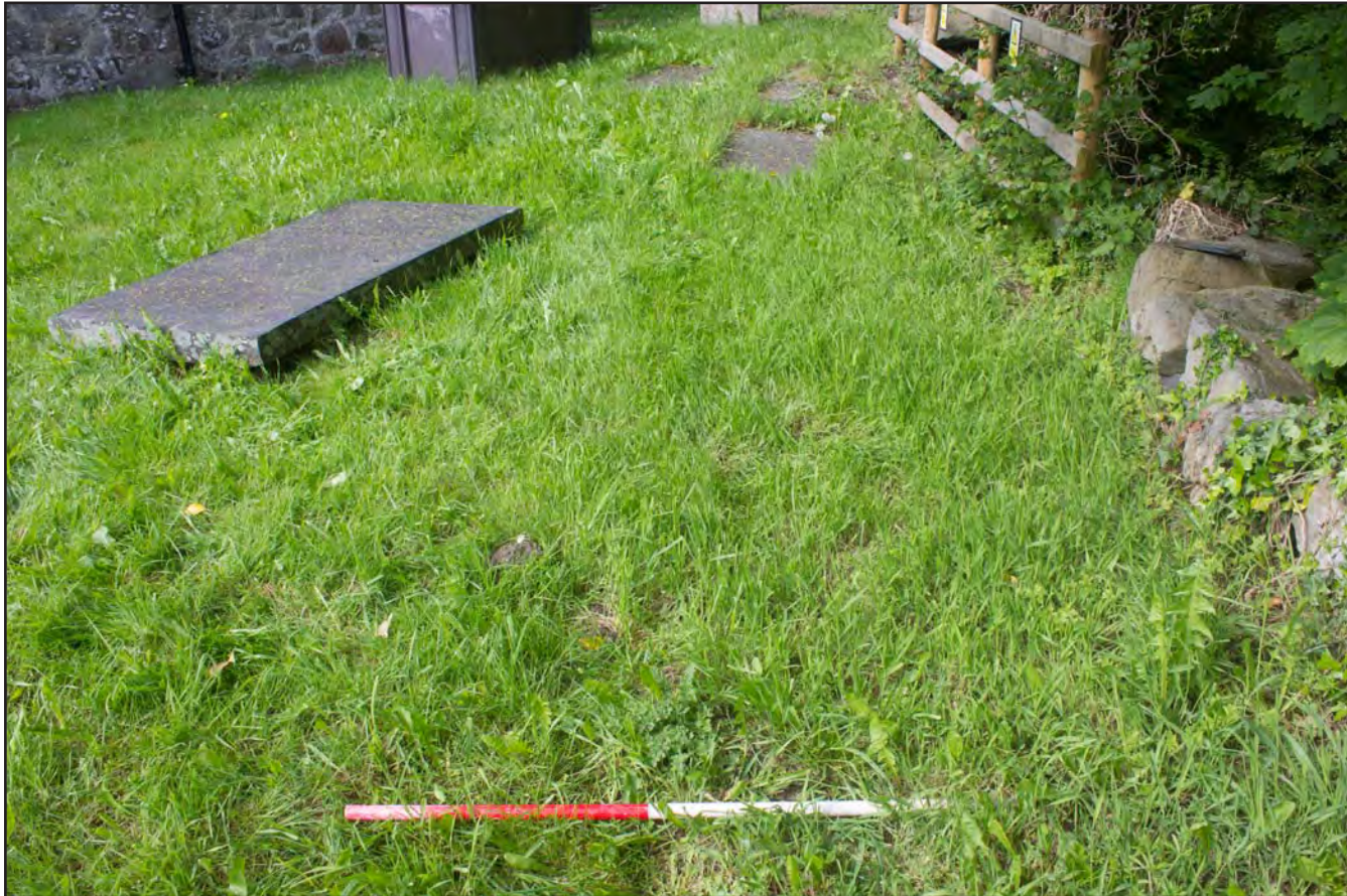
Plate 37: Pre excavation shot of drainage route for septic tank to soakaway (east) , at St. Mary's Church, Church Street, Llanfair Talhaiarn, Conwy - from the east - 1.00m scale
