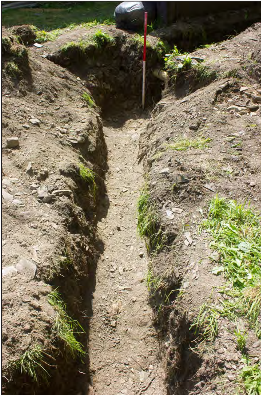
Plate 44: Post excavation shot of drainage route for septic tank to soakaway (east) , at St. Mary's Church, Church Street, Llanfair Talhaiarn, Conwy - from the northeast - 1.00m scale
