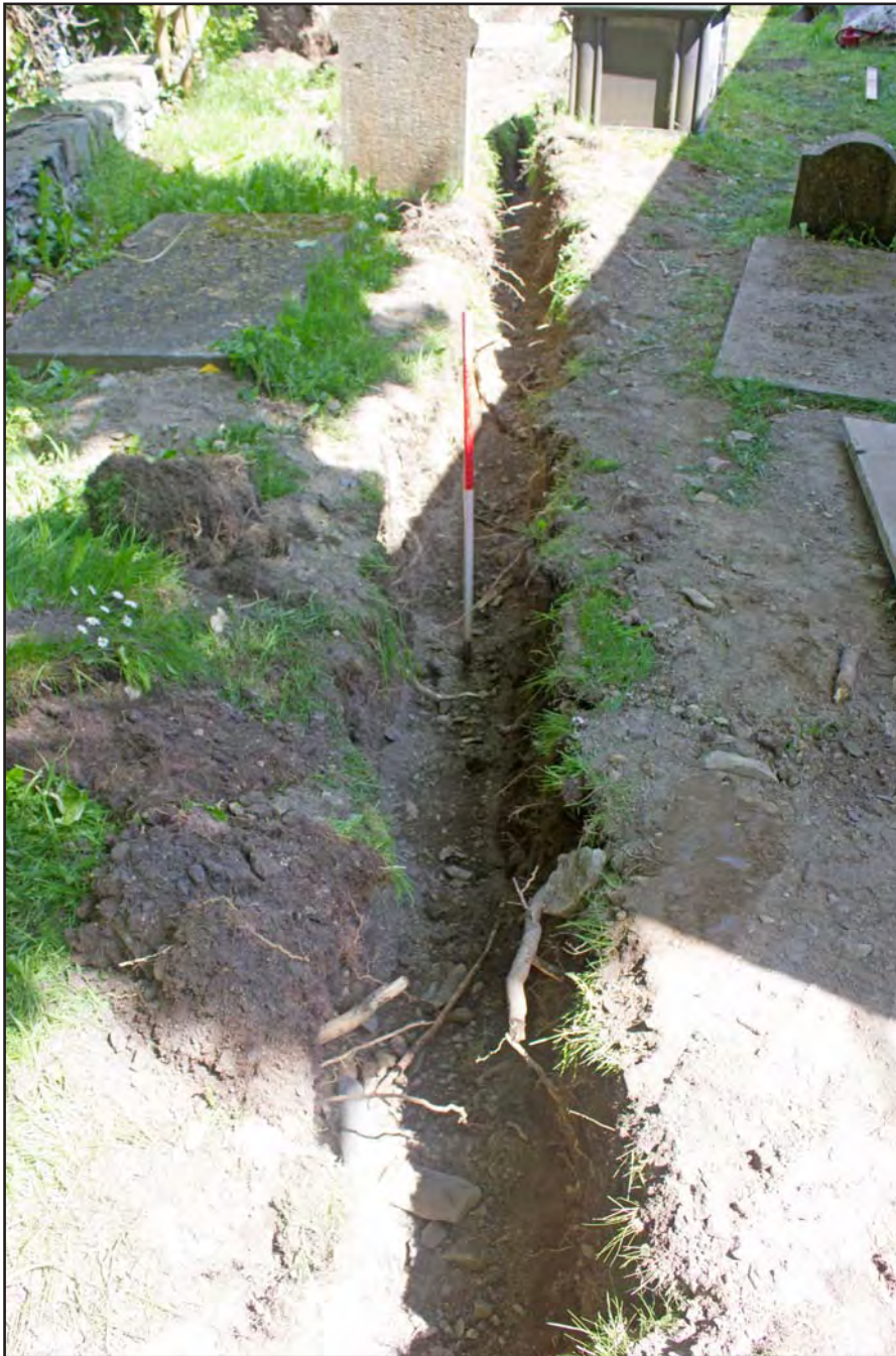
Plate 42: Post excavation shot of drainage route for septic tank to soakaway (west) , at St. Mary's Church, Church Street, Llanfair Talhaiarn, Conwy - from the west - 1.00m scale
