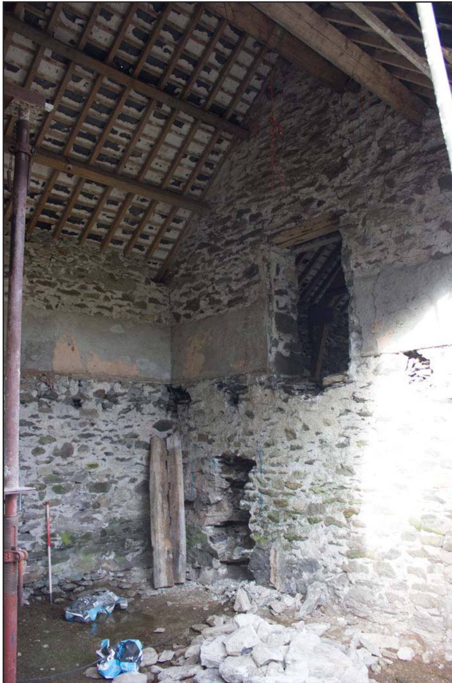
Plate 31: Internal shot of Room 2, within outbuilding at Cefnhirfynydd Isa, Glasfryn, Conwy - from the southeast - 1.00m scale
