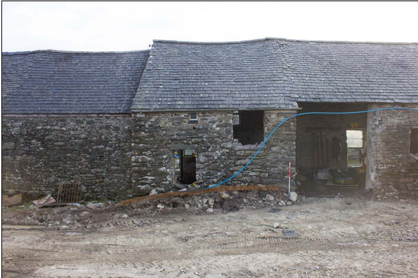
Plate 15: West facing elevation (centre-left) of outbuilding, at Cefnhirfynydd Isa, Glasfryn, Conwy - from the west - 1.00m scale
