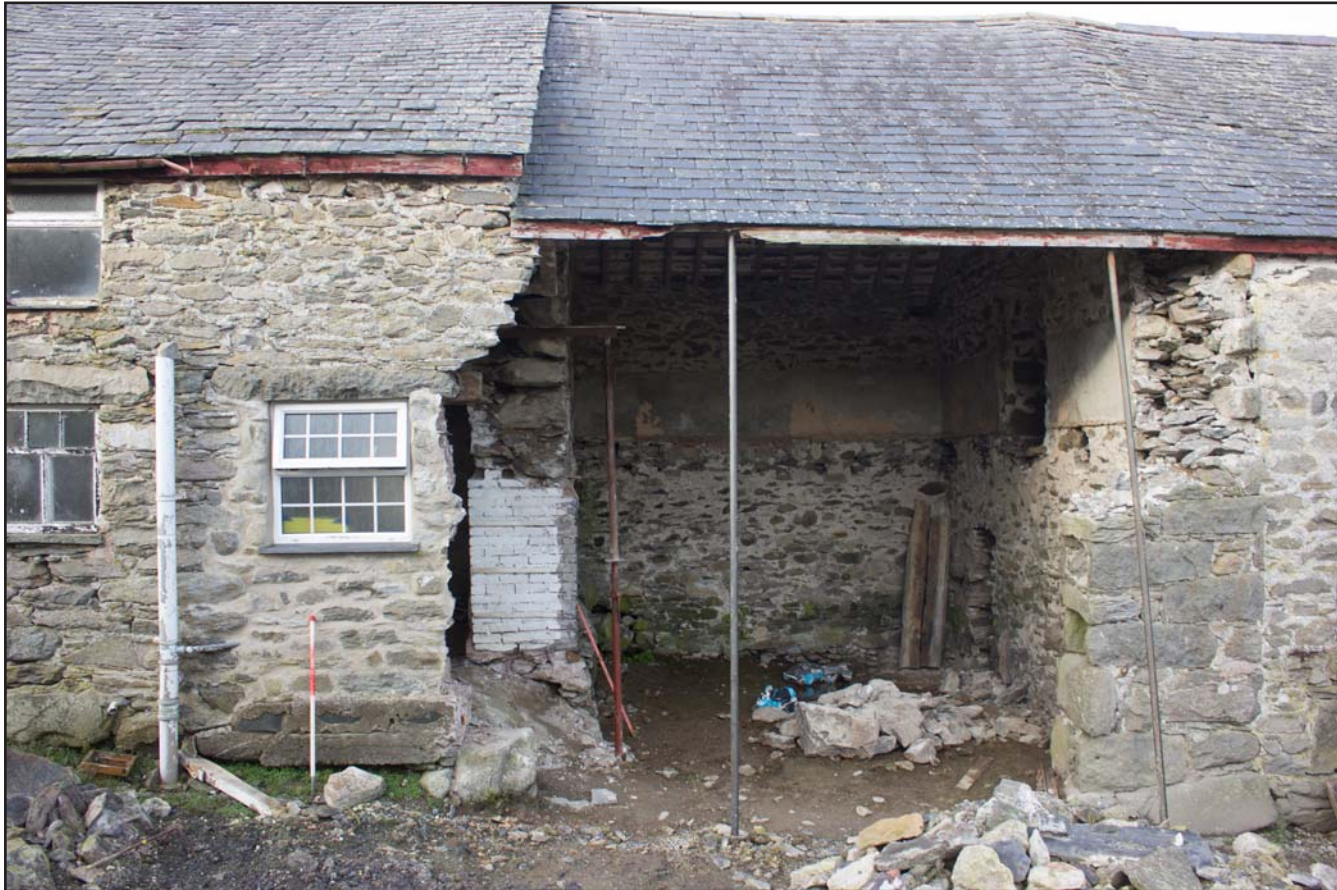
Plate 22: East facing elevation (centre/rooms 2/3) of outbuilding, at Cefnhirfynydd Isa, Glasfryn, Conwy - from the east - 1.00m scale
