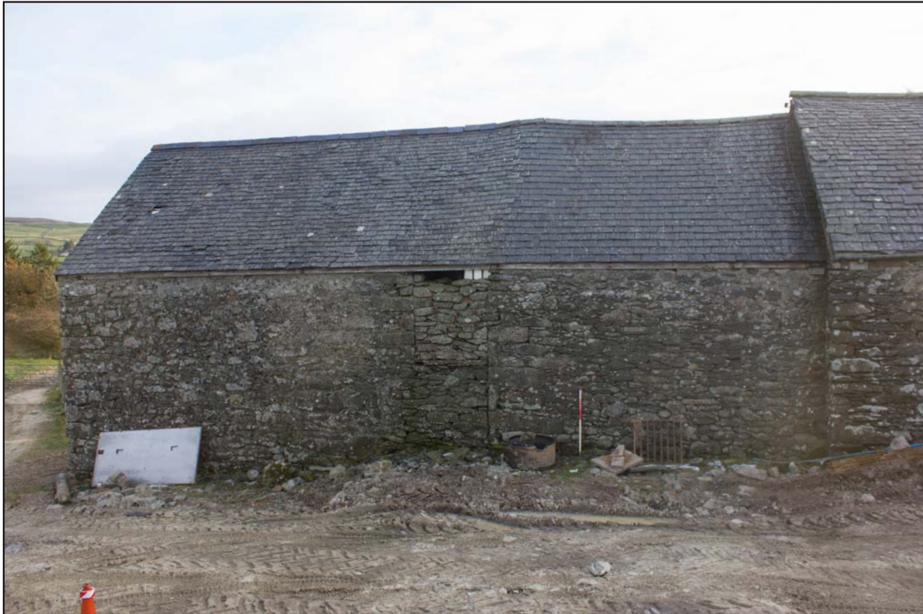
Plate 16: West facing elevation (left) of outbuilding, at Cefnhirfynydd Isa, Glasfryn, Conwy - from the west - 1.00m scale
