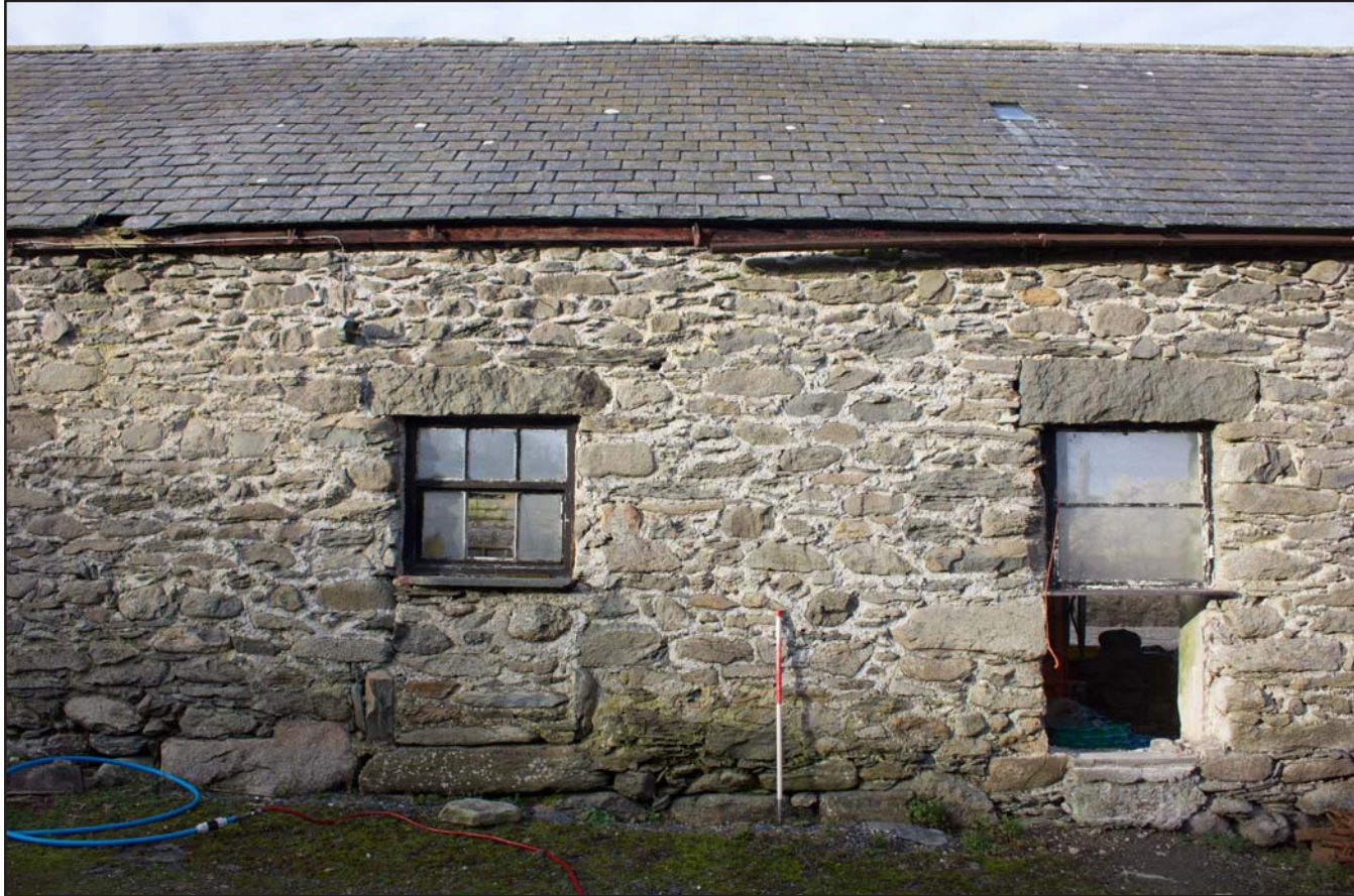
Plate 24: East facing elevation (centre - room 4) of outbuilding, at Cefnhirfynydd Isa, Glasfryn, Conwy - from the east - 1.00m scale
