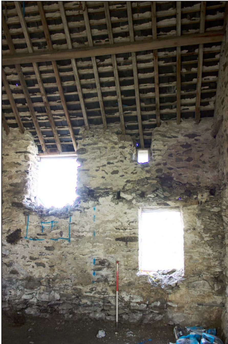
Plate 36: Internal shot of Room 3, within outbuilding at Cefnhirfynydd Isa, Glasfryn, Conwy - from the east - 1.00m scale
