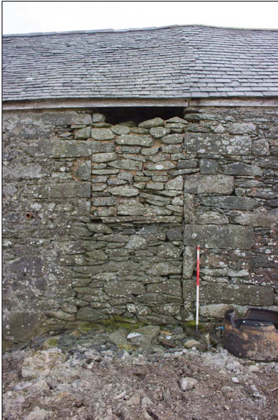
Plate 17: West facing elevation (left) of outbuilding - blocked up doorway, at Cefnhirfynydd Isa, Glasfryn, Conwy - from the west - 1.00m scale
