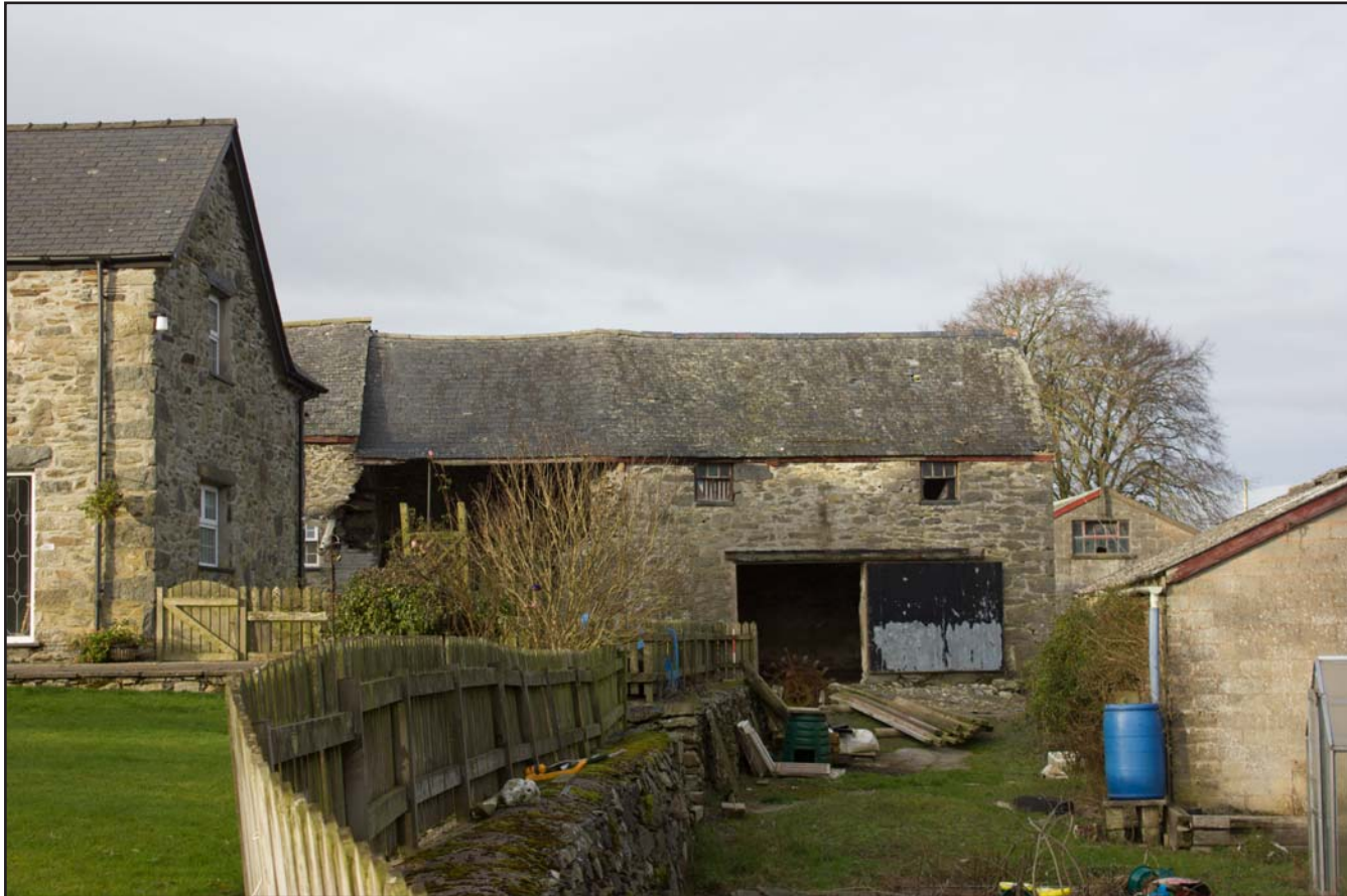
Plate 07: Close up context shot of outbuilding with Farmhouse and NE barn, at Cefnhirfynydd Isa, Glasfryn, Conwy - from the east - no scale
