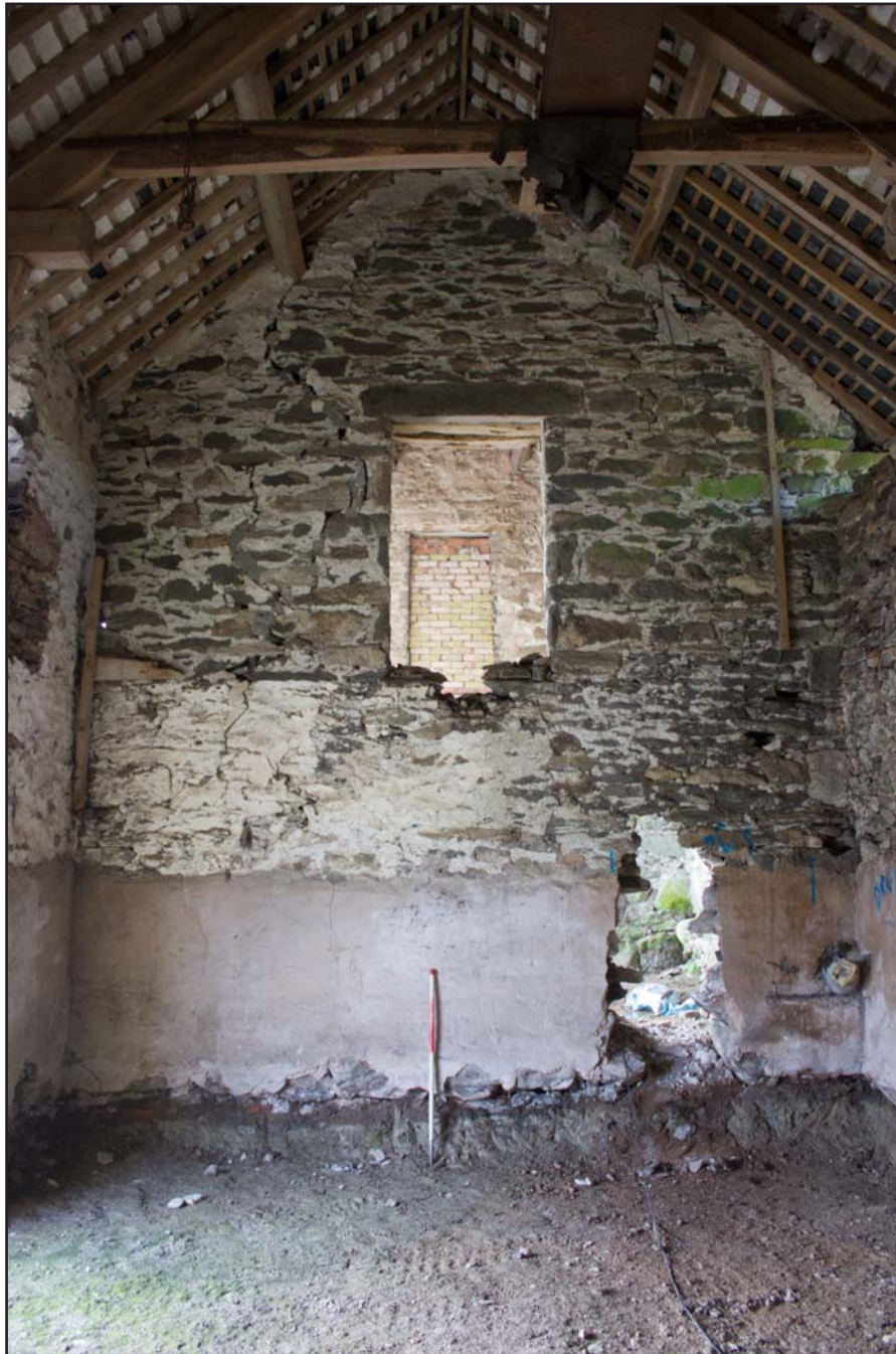
Plate 28: Internal shot of Room 1, within outbuilding at Cefnhirfynydd Isa, Glasfryn, Conwy - from the south - 1.00m scale
