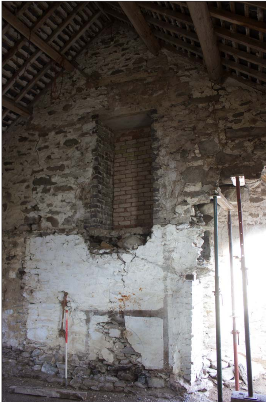
Plate 34: Internal shot of Room 3, within outbuilding at Cefnhirfynydd Isa, Glasfryn, Conwy - from the southeast - 1.00m scale
