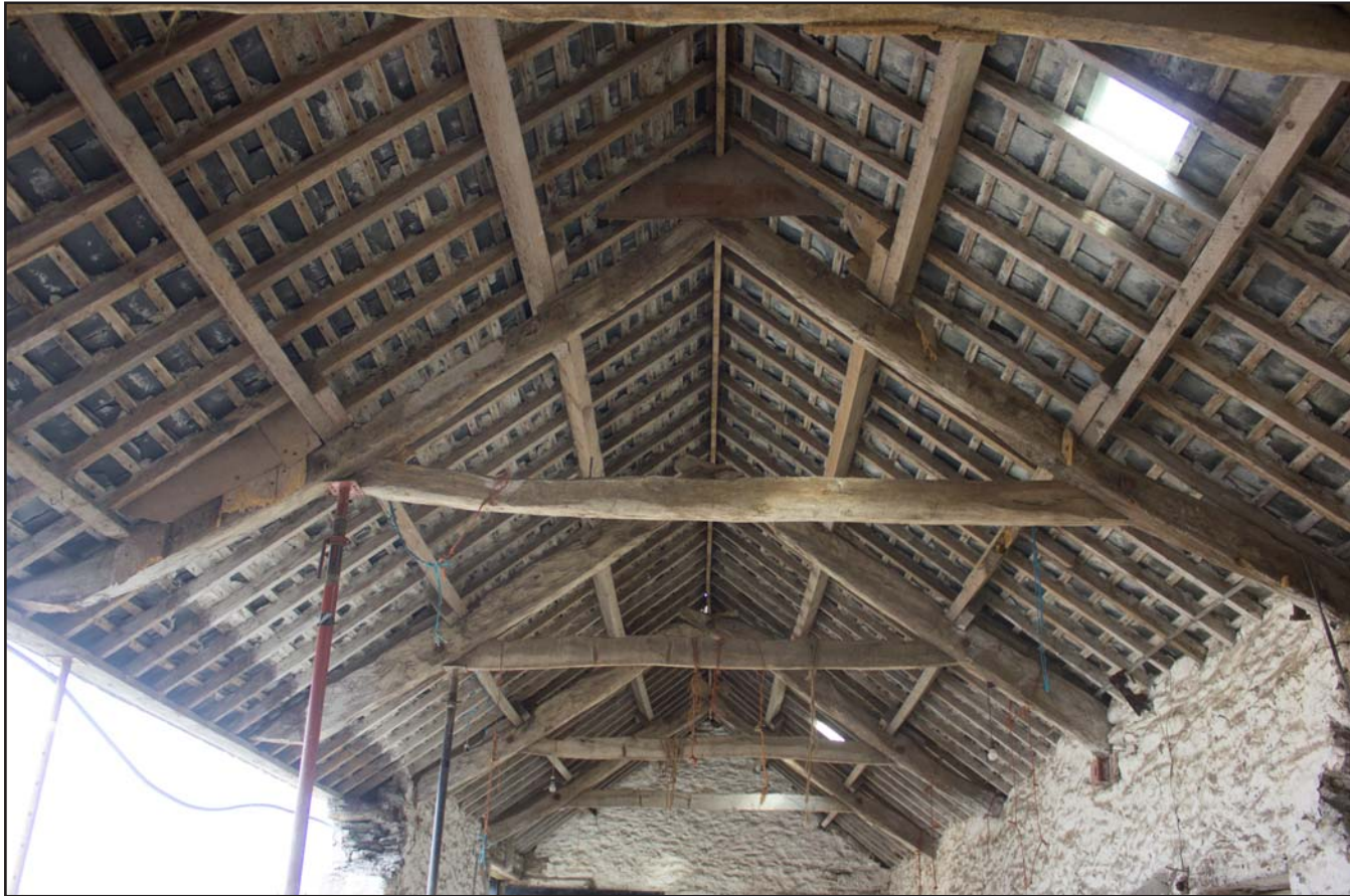
Plate 41: Internal shot of Room 4's ceiling, within outbuilding at Cefnhirfynydd Isa, Glasfryn, Conwy - from the south - no scale
