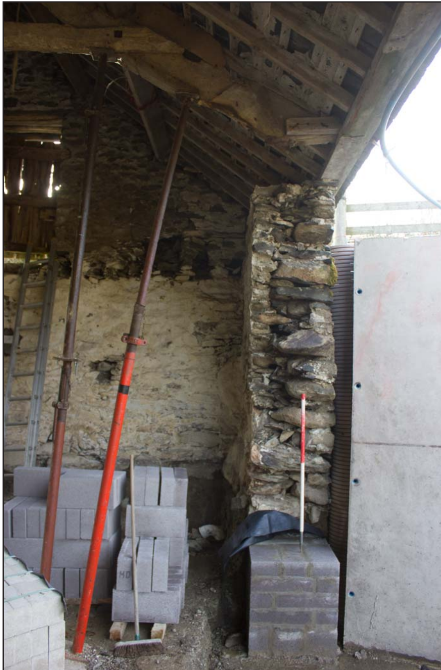
Plate 44: Breached western wall of Room 4 western elevation, within outbuilding at Cefnhirfynydd Isa, Glasfryn, Conwy - from the south - 1.00m scale
