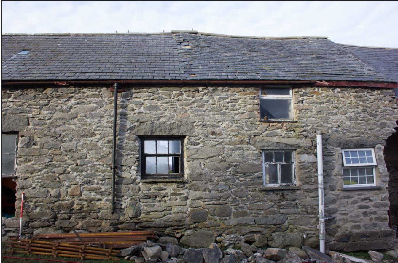
Plate 23: East facing elevation (centre/rooms 3/4) of outbuilding, at Cefnhirfynydd Isa, Glasfryn, Conwy - from the east - 1.00m scale
