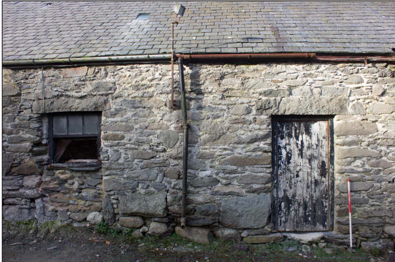
Plate 25: East facing elevation (external door room 4) of outbuilding, at Cefnhirfynydd Isa, Glasfryn, Conwy - from the east - 1.00m scale
