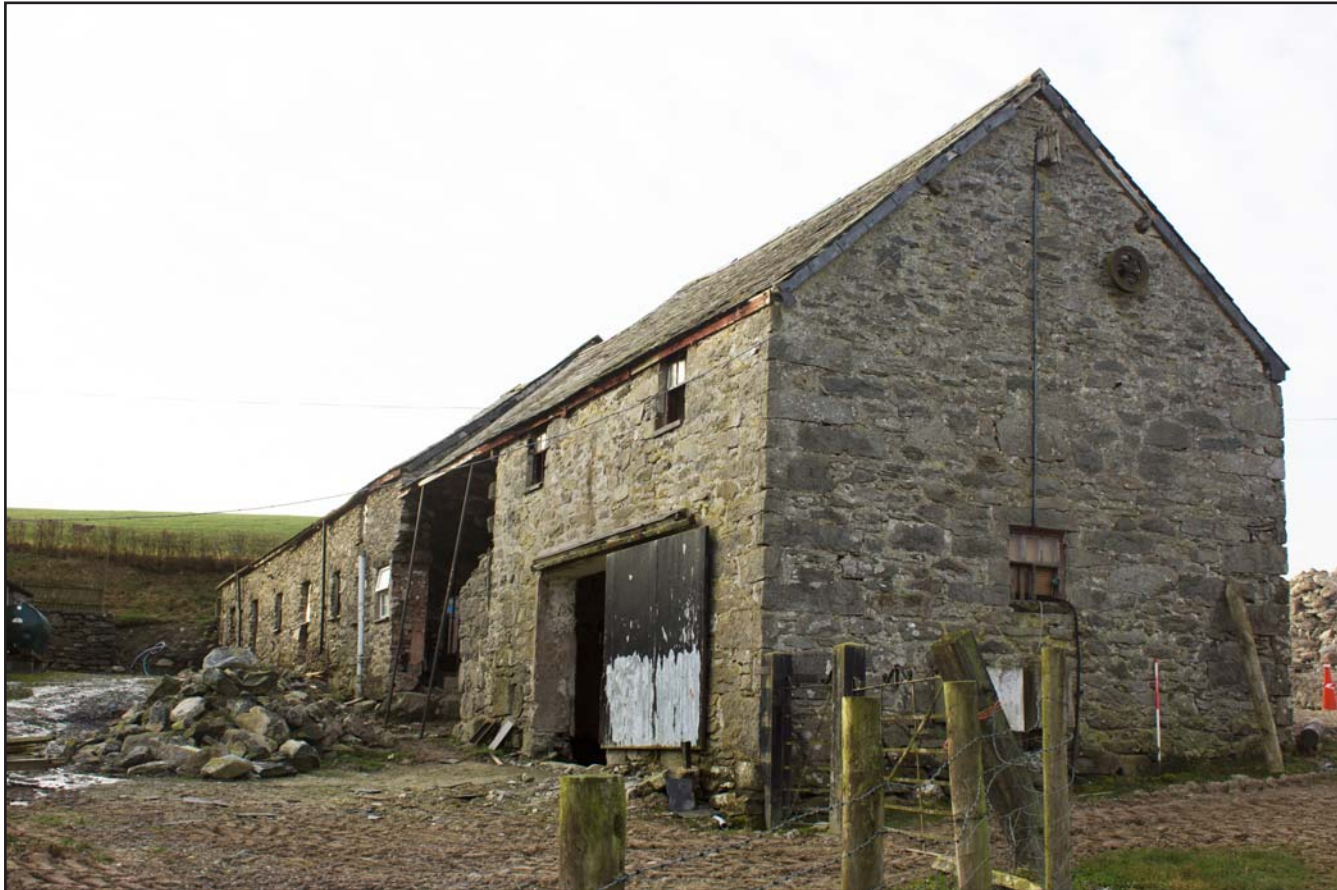
Plate 20: Oblique shot of eastern and northern elevations of outbuilding, at Cefnhirfynydd Isa, Glasfryn, Conwy - from the northeast - 1.00m scale
