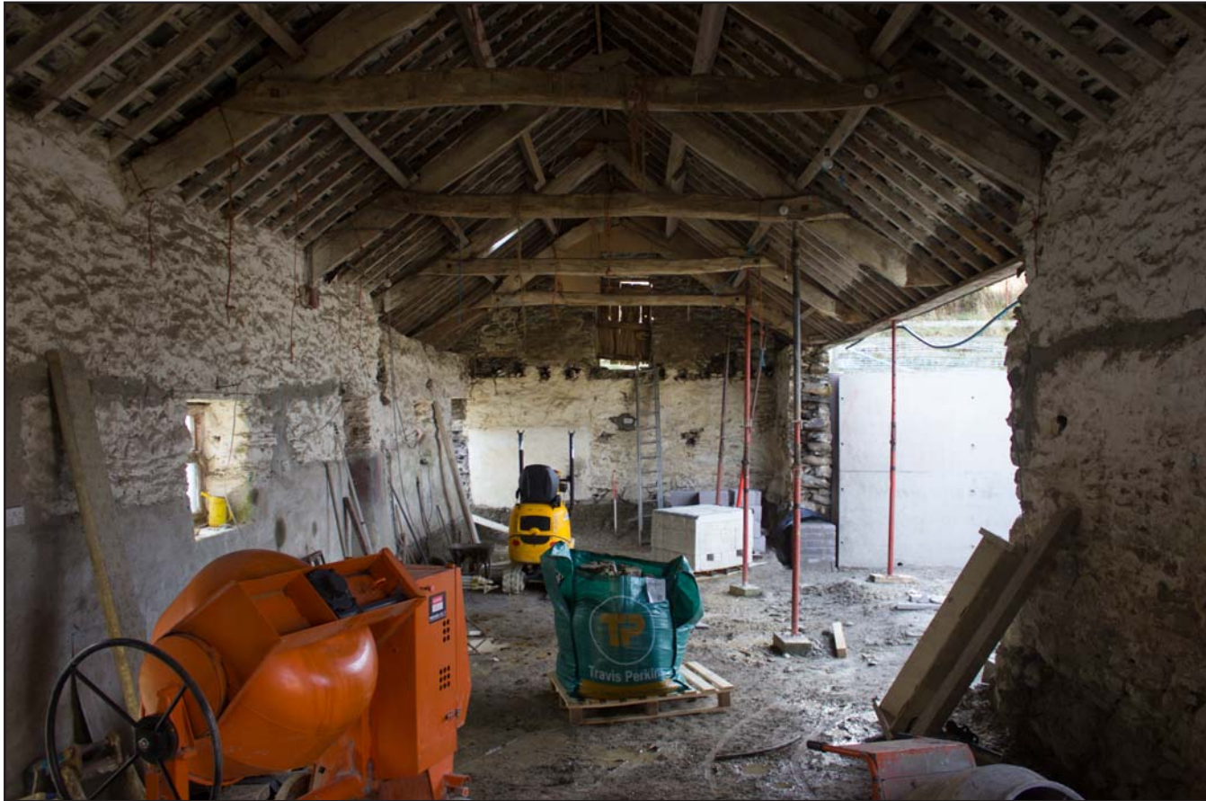
Plate 38: Internal shot of Room 4, within outbuilding at Cefnhirfynydd Isa, Glasfryn, Conwy - from the north - 1.00m scale
