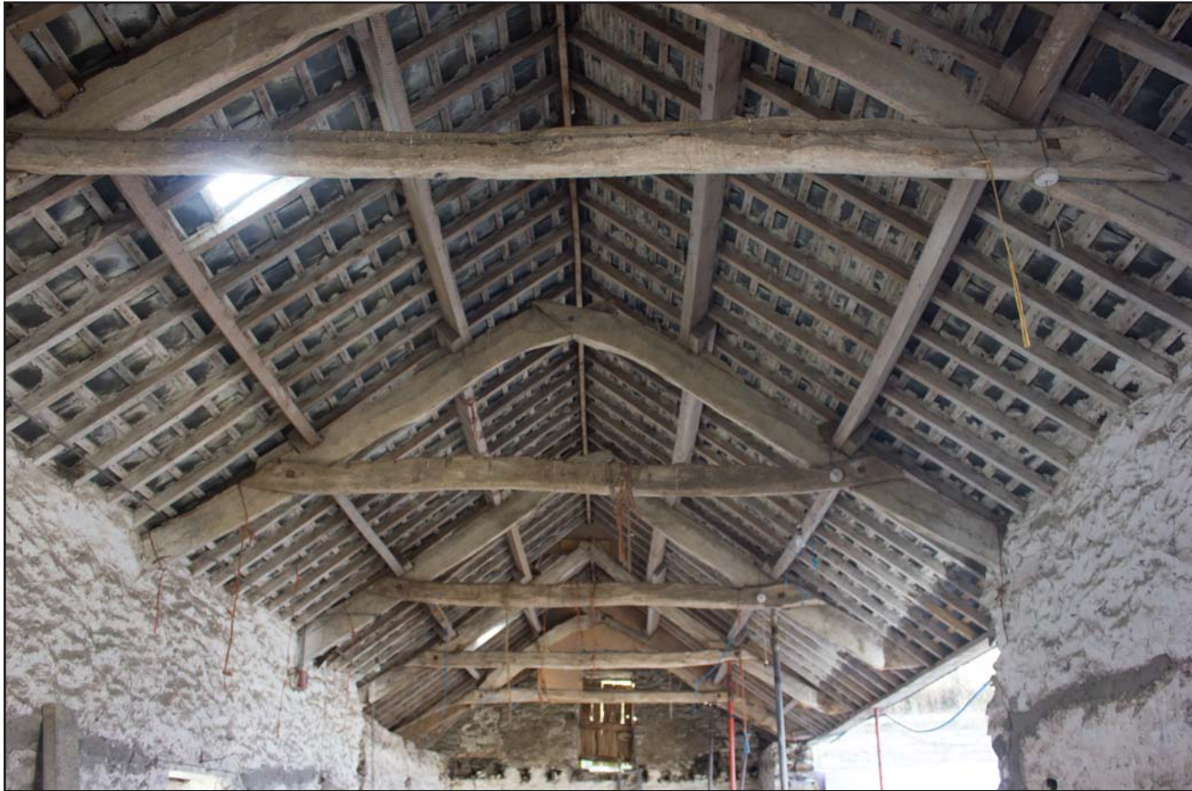
Plate 39: Internal shot of Room 4's ceiling, within outbuilding at Cefnhirfynydd Isa, Glasfryn, Conwy - from the north - no scale
