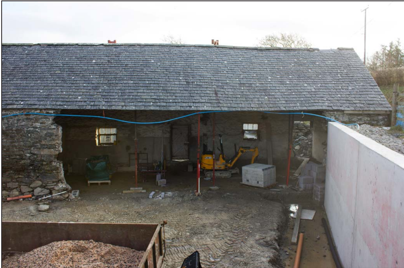
Plate 13: West facing elevation (right) of outbuilding, at Cefnhirfynydd Isa, Glasfryn, Conwy - from the west - 1.00m scale
