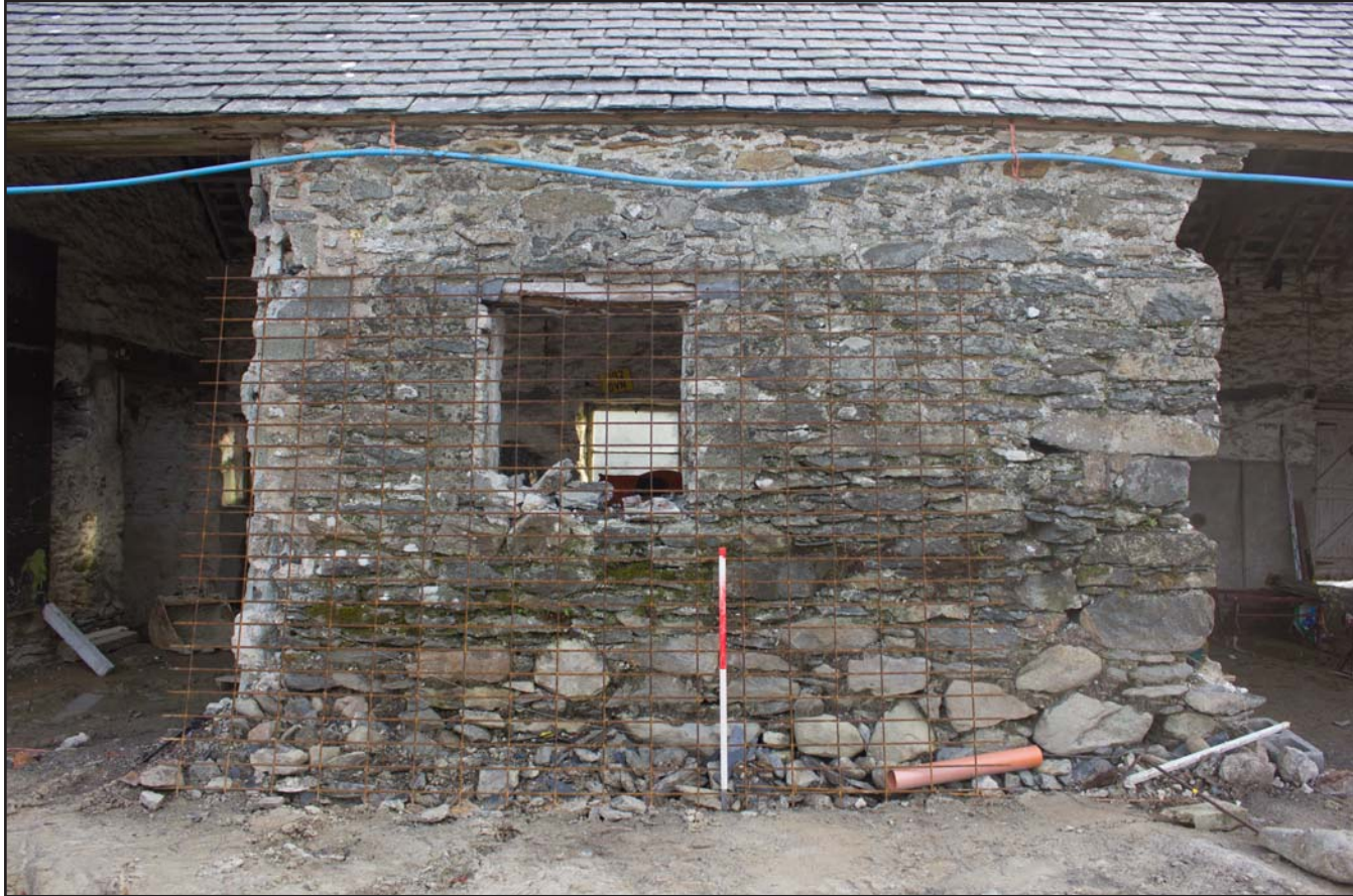
Plate 14: West facing elevation (centre-right) of outbuilding, at Cefnhirfynydd Isa, Glasfryn, Conwy - from the west - 1.00m scale
