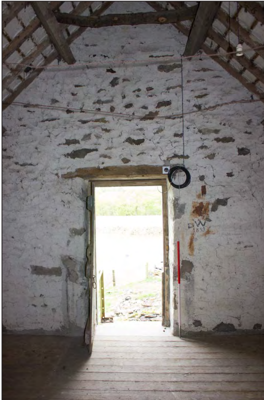
Plate 21: Store 1, First floor, within Building 1 - Cart and Threshing Barn at Gaer Gerrig, Llangwm, Conwy - from the southwest- 1.00m scale
