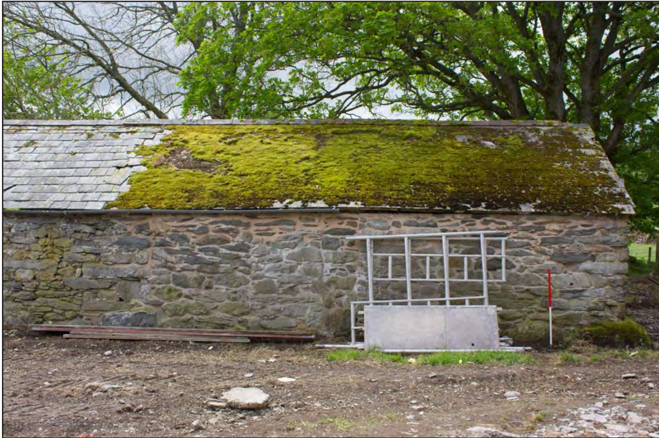
Plate 45: Northeast elevation (right) of Building 3 - Pigstiesat Gaer Gerrig, Llangwm, Conwy - from the northeast - 1.00m scale
