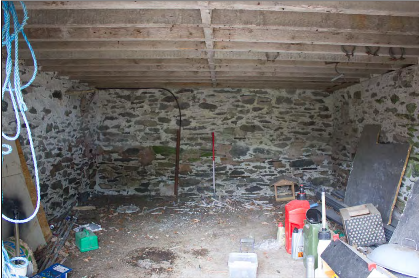
Plate 18: Cart Barn within Building 1 - Cart and Threshing Barn at Gaer Gerrig, Llangwm, Conwy - from the southeast - 1.00m scale
