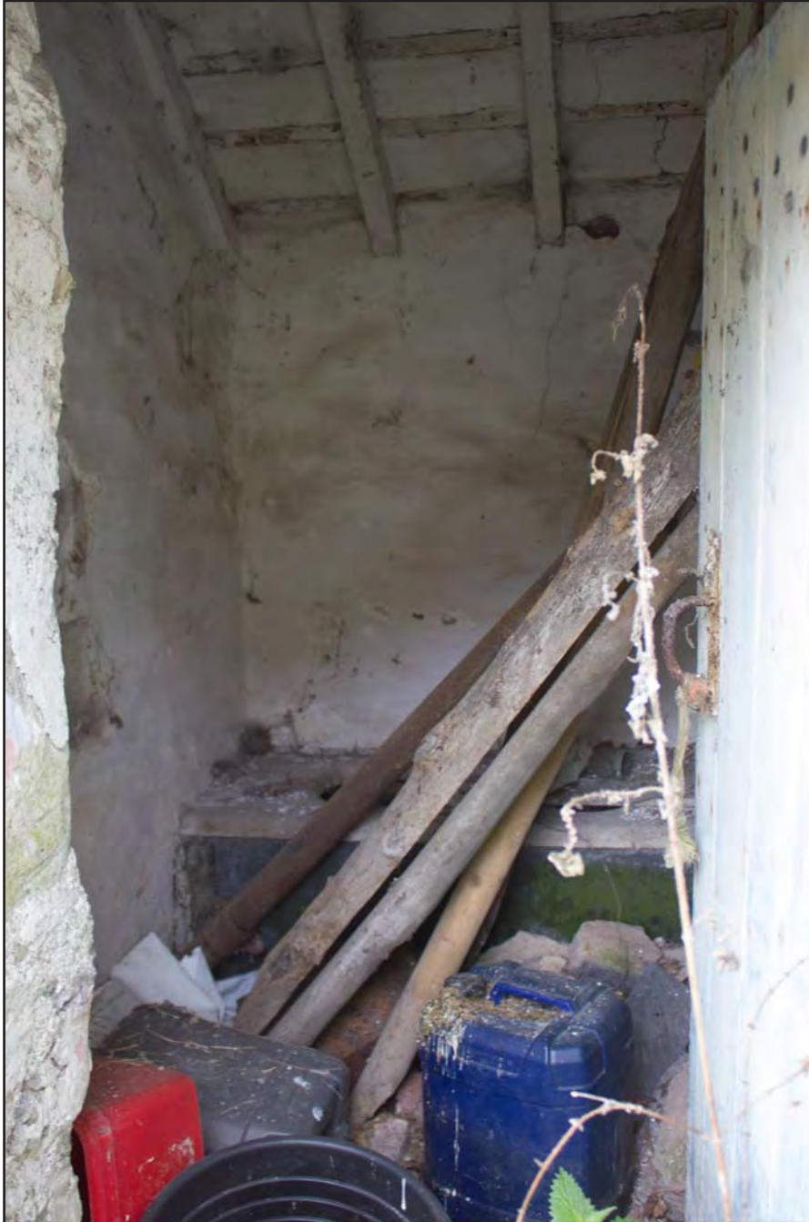
Plate 52: Internal shot outhouse within Building 3 - Pigsties at Gaer Gerrig, Llangwm, Conwy - from the north - 1.00m scale
