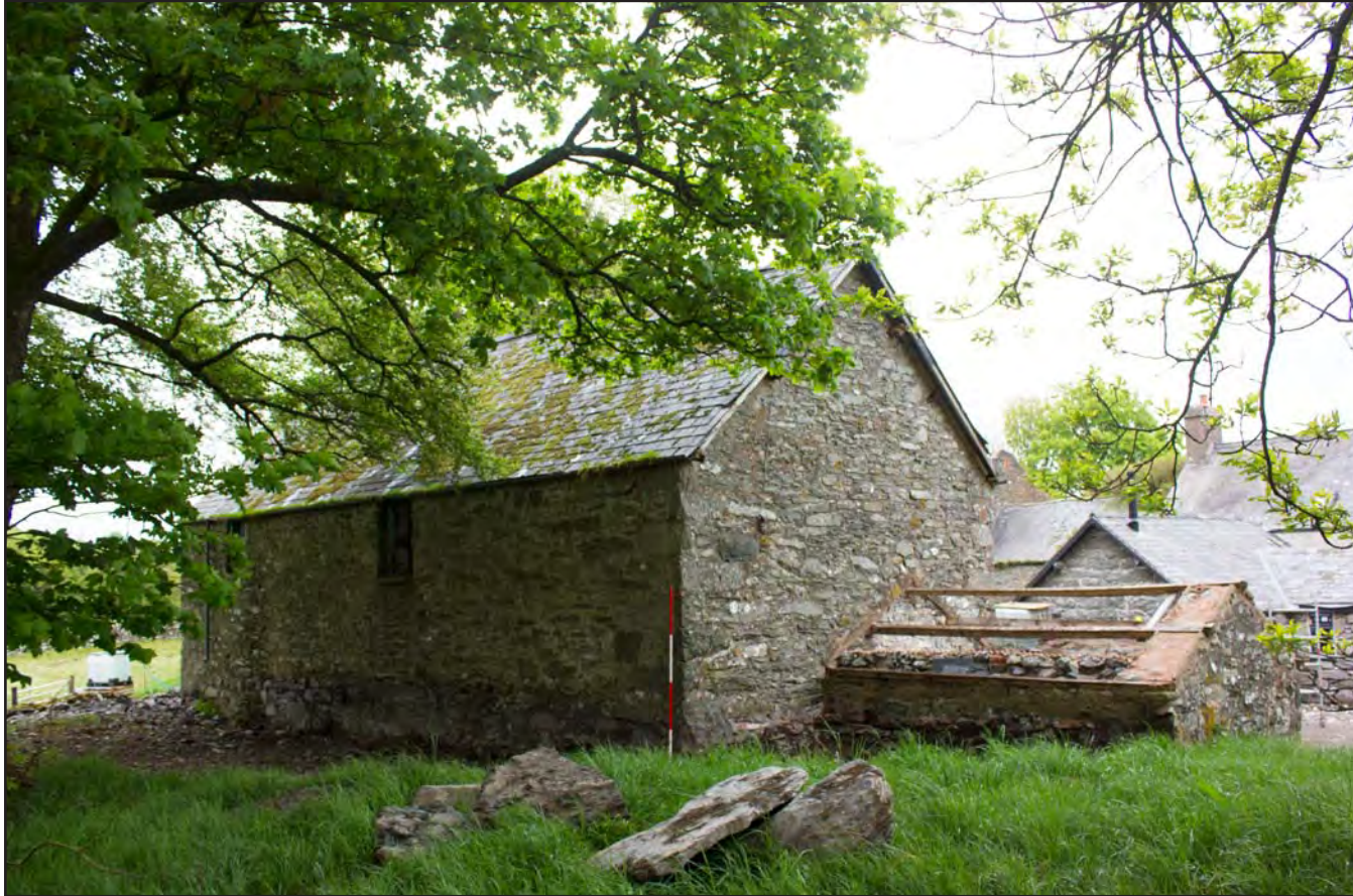
Plate 10: Oblique shot of northwest & southwest elevations of Building 1 - Cart and Threshing Barn at Gaer Gerrig, Llangwm, Conwy - from the west - 2.00m scale
