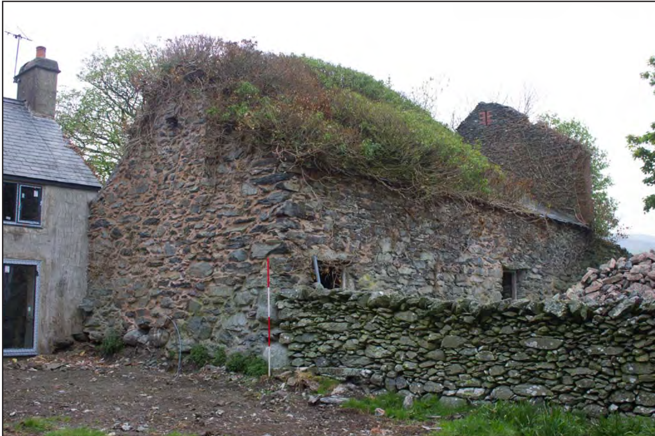
Plate 58: Oblique shot of southwest & northeast elevations of Building 4 - Cowhouse/Shippon at Gaer Gerrig, Llangwm, Conwy - from the south - 2.00m scale
