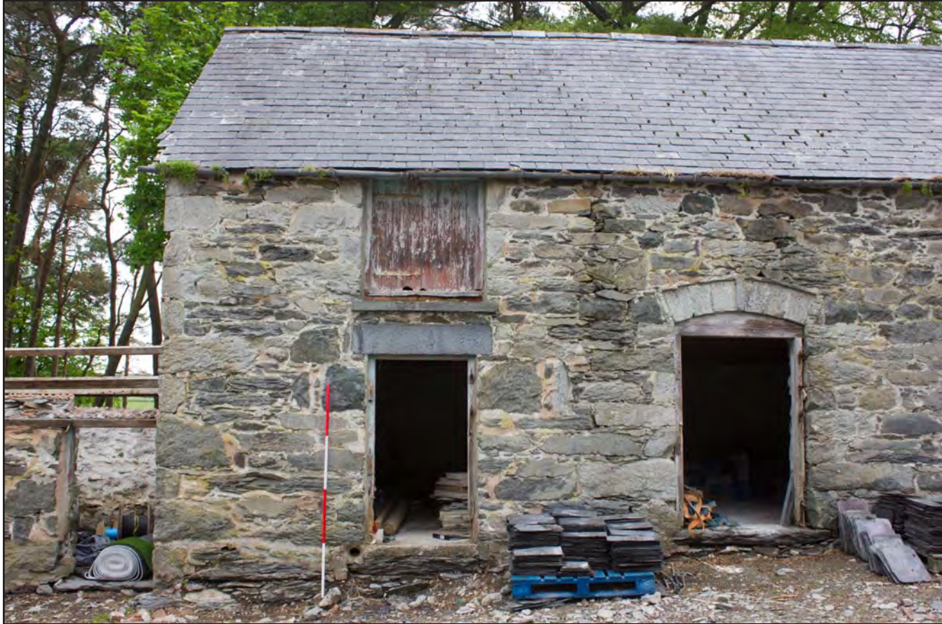
Plate 02: Southeast elevation (left) of Building 1 - Cart and Threshing Barn at Gaer Gerrig, Llangwm, Conwy - from the southeast - 2.00m scale
