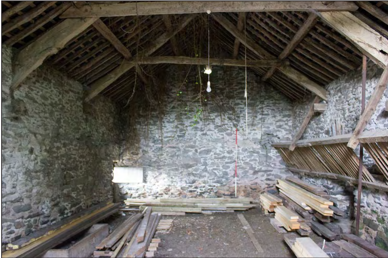
Plate 64: Internal shot of Building 4 - Cowhouse/Shippon at Gaer Gerrig, Llangwm, Conwy - from the northeast - 2.00m scale
