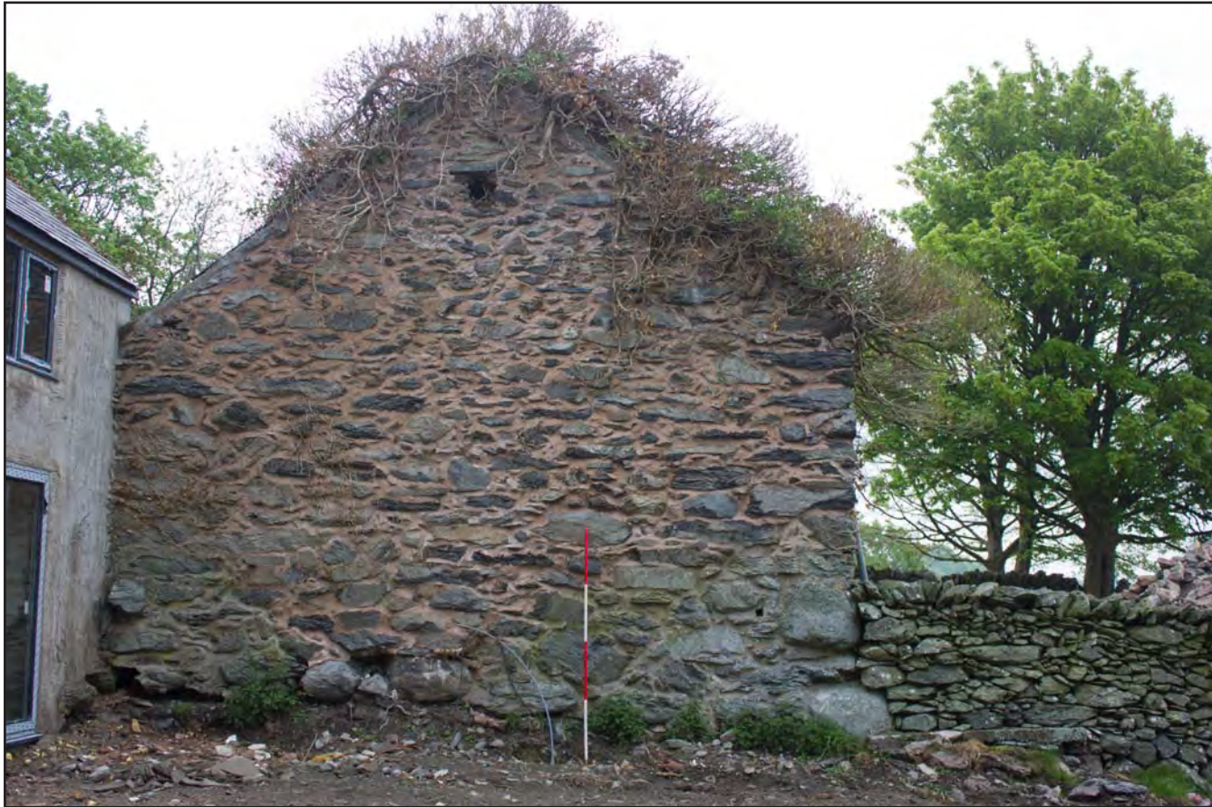
Plate 59: Southwest elevation of Building 4 - Cowhouse/Shippon at Gaer Gerrig, Llangwm, Conwy - from the southwest - 2.00m scale
