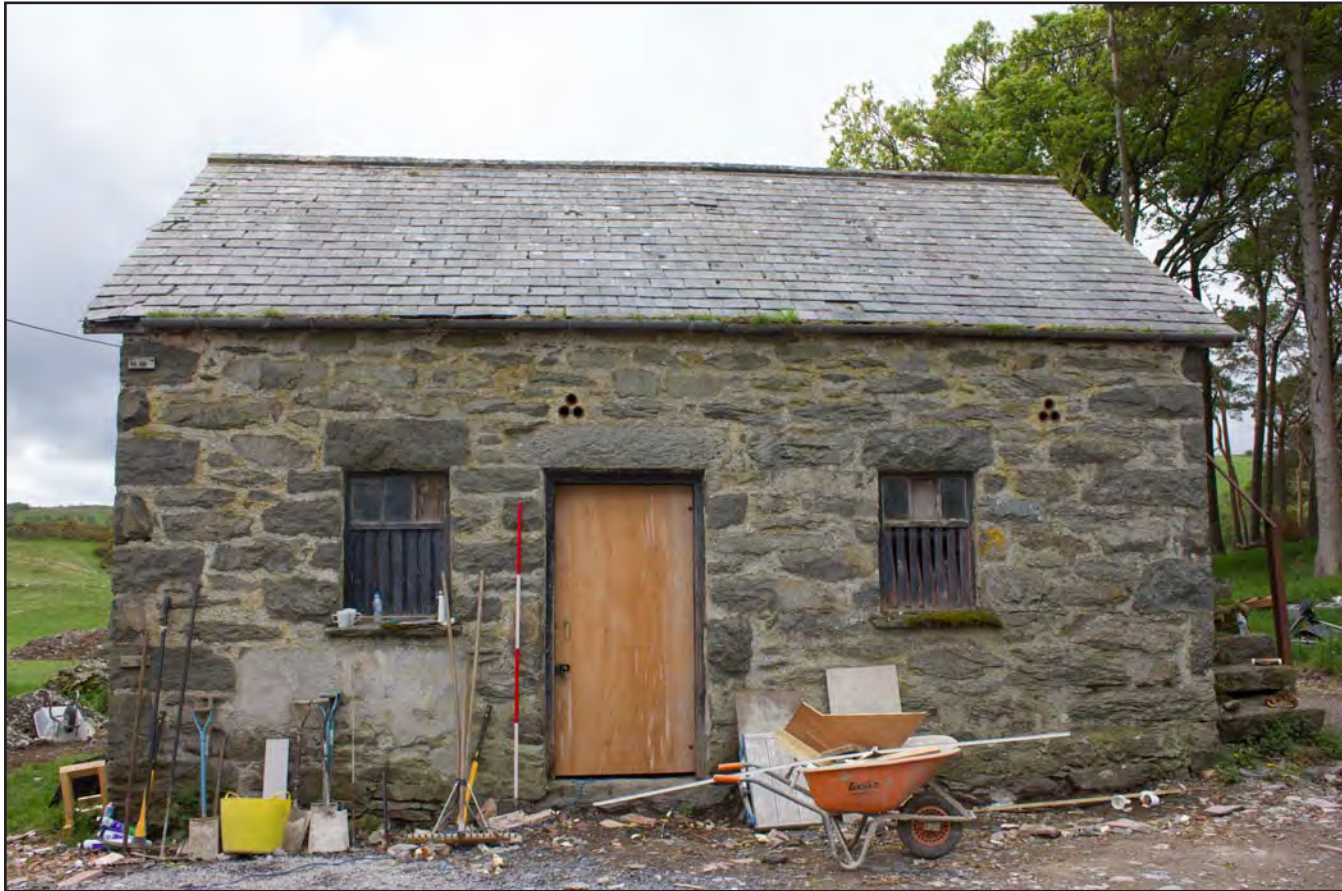
Plate 24: Northeast elevation of Building 2 - Horse/Pony Stable at Gaer Gerrig, Llangwm, Conwy - from the northeast - 2.00m scale
