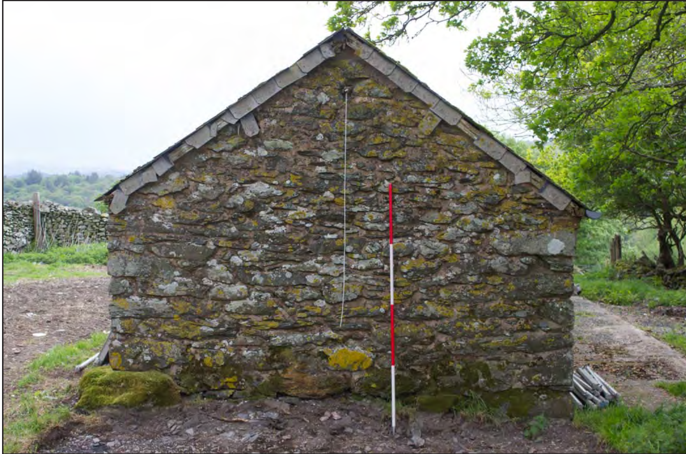
Plate 47: Northwest elevation of Building 3 - Pigsties at Gaer Gerrig, Llangwm, Conwy - from the northwest - 2.00m scale
