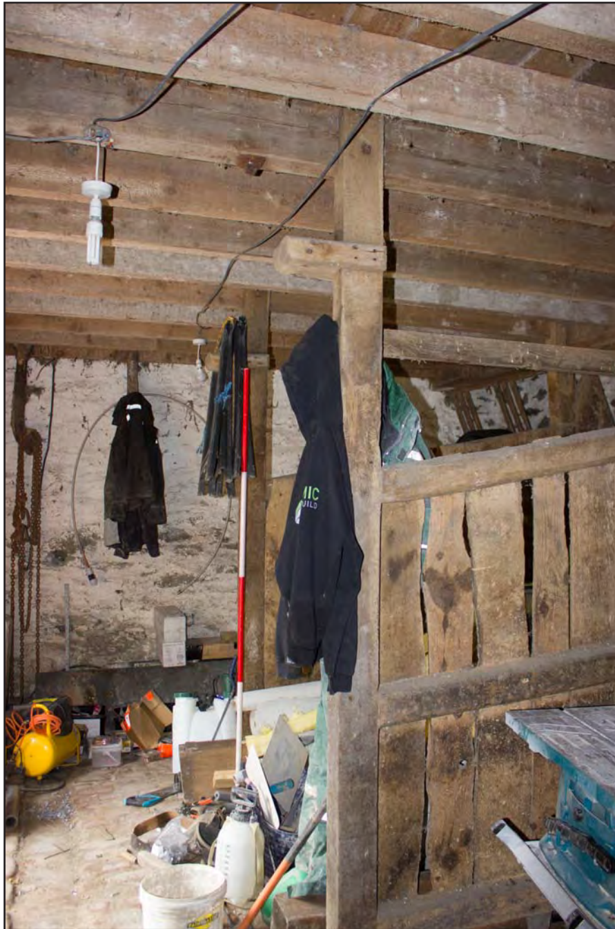
Plate 32: Oblique shot of interior of Building 2 - Horse/Pony Stable at Gaer Gerrig, Llangwm, Conwy - from the northwest - 2.00m scale
