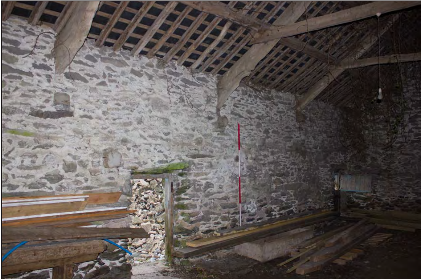
Plate 67: Oblique internal shot of Building 4 - Cowhouse/Shippon at Gaer Gerrig, Llangwm, Conwy - from the northeast - 2.00m scale
