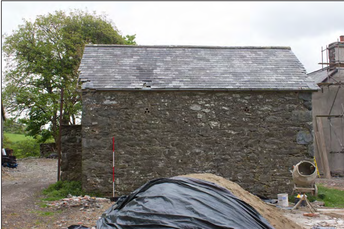
Plate 28: Southwest elevation of Building 2 - Horse/Pony Stable at Gaer Gerrig, Llangwm, Conwy - from the southwest - 2.00m scale
