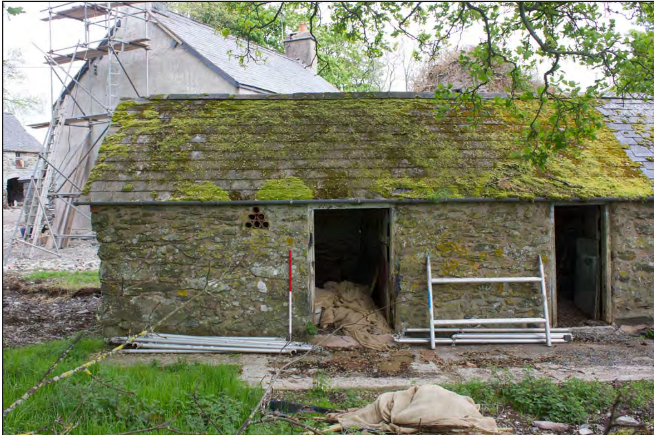
Plate 38: Southwest elevation (left) of Building 3 - Pigsties at Gaer Gerrig, Llangwm, Conwy - from the southwest - 1.00m scale
