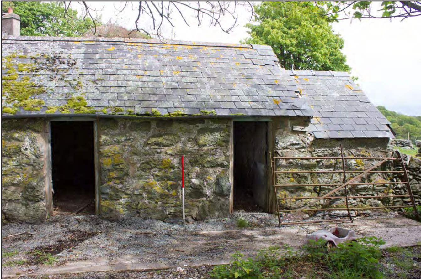
Plate 40: Southwest elevation (right) of Building 3 - Pigsties at Gaer Gerrig, Llangwm, Conwy - from the southwest - 1.00m scale
