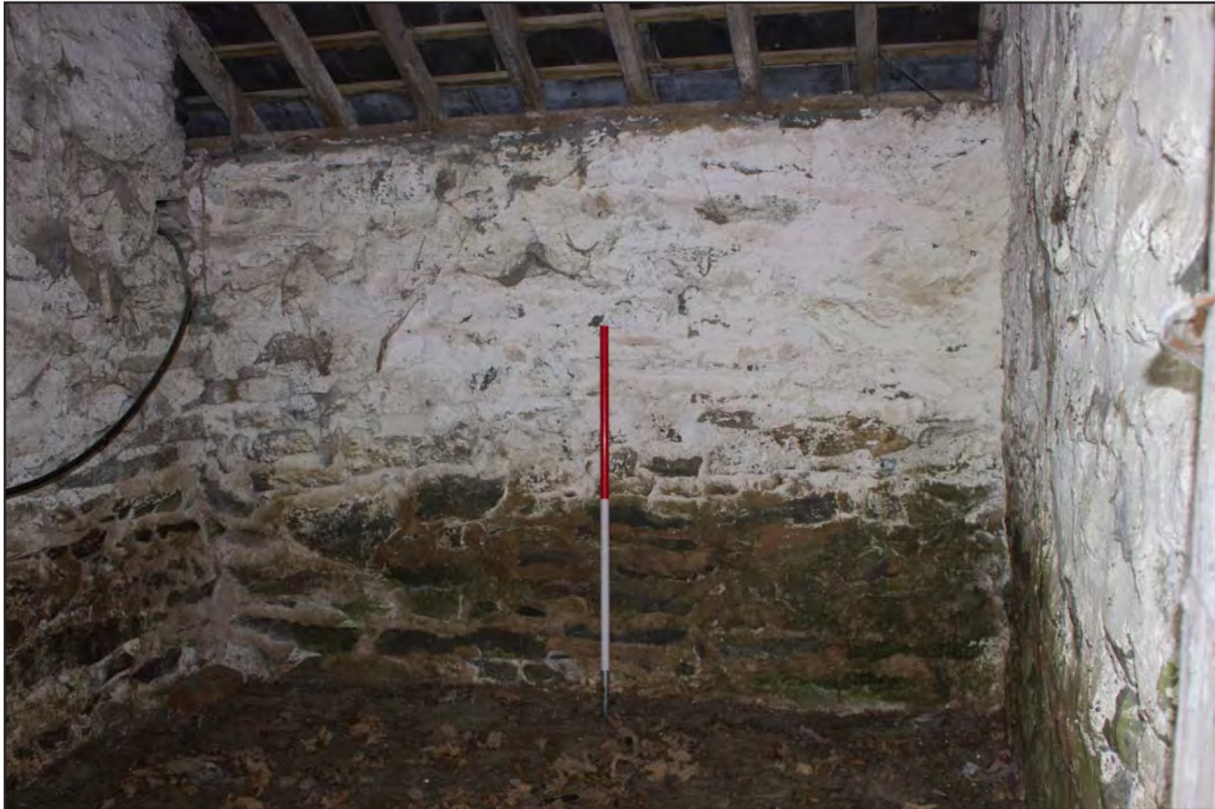
Plate 51: Internal shot Pigsty 4 within Building 3 - Pigsties at Gaer Gerrig, Llangwm, Conwy - from the south - 1.00m scale
