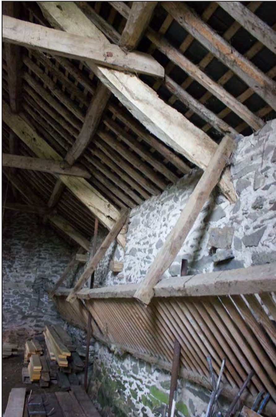
Plate 69: Wooden feeder in Building 4 - Cowhouse/Shippon at Gaer Gerrig, Llangwm, Conwy - from the northeast - 2.00m scale
