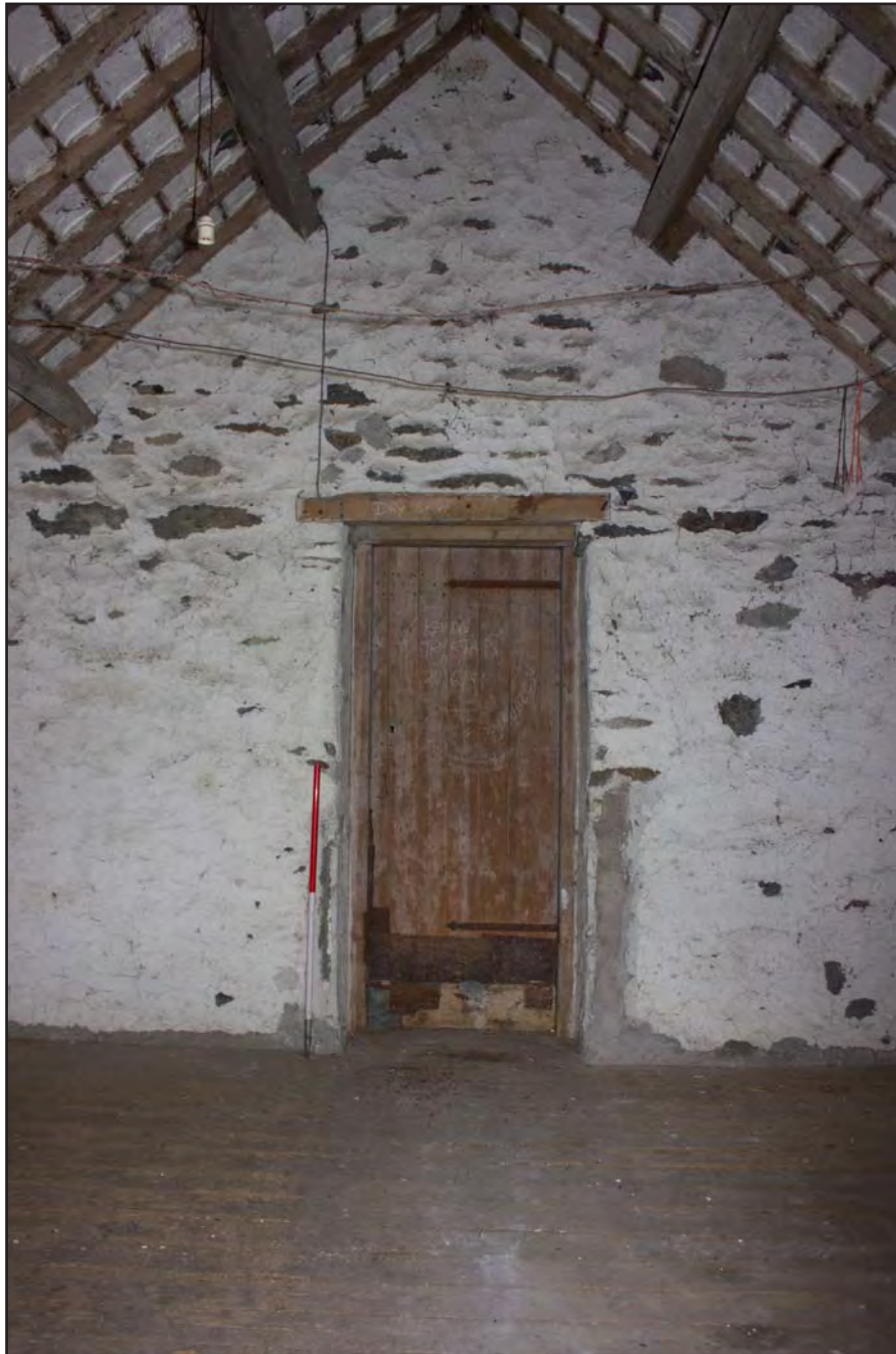
Plate 20: Store 1 on first floor within Building 1 - Cart and Threshing Barn at Gaer Gerrig, Llangwm, Conwy - from the northeast - 1.00m scale
