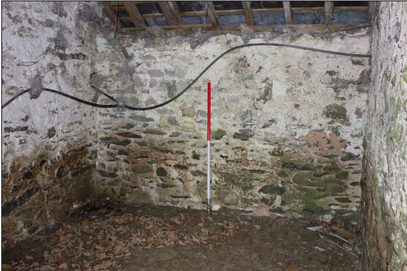
Plate 50: Internal shot Pigsty 3 within Building 3 - Pigsties at Gaer Gerrig, Llangwm, Conwy - from the south - 1.00m scale
