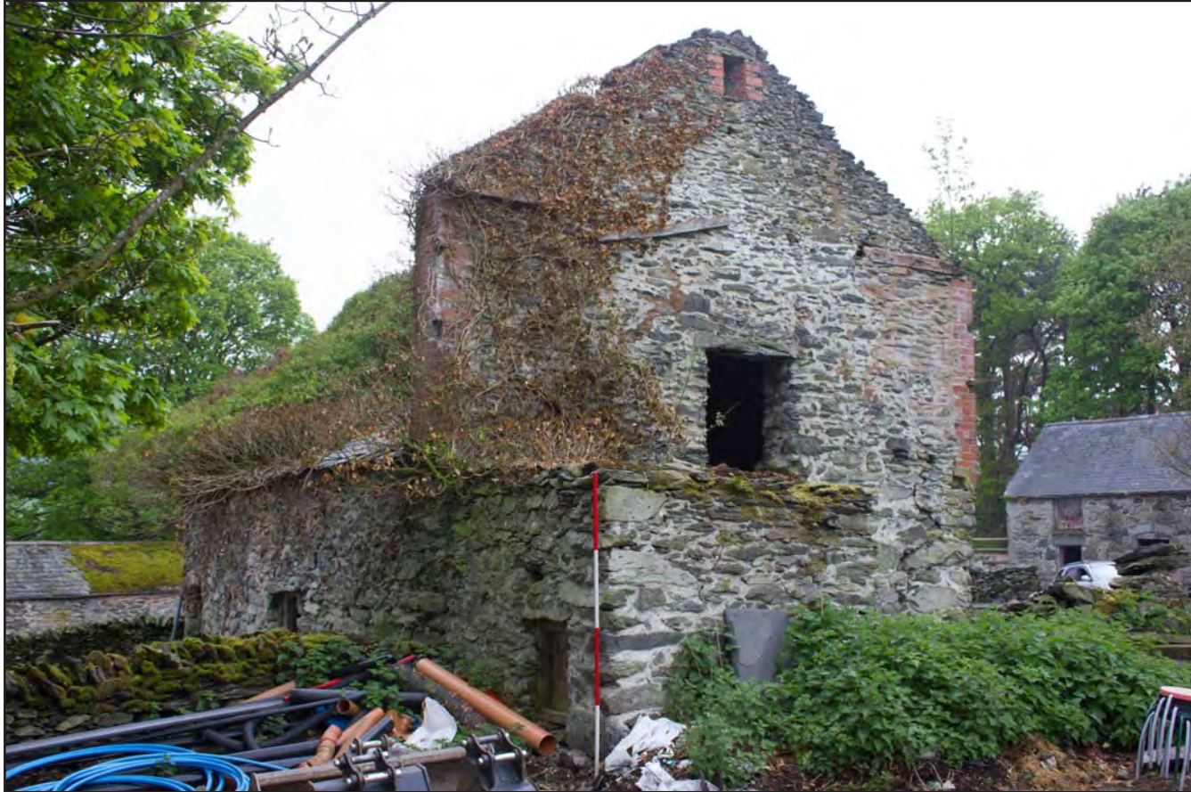
Plate 54: Oblique shot of northeast & southeast elevations of Building 4 - Cowhouse/Shippon at Gaer Gerrig, Llangwm, Conwy - from the north-northeast - 2.00m scale
