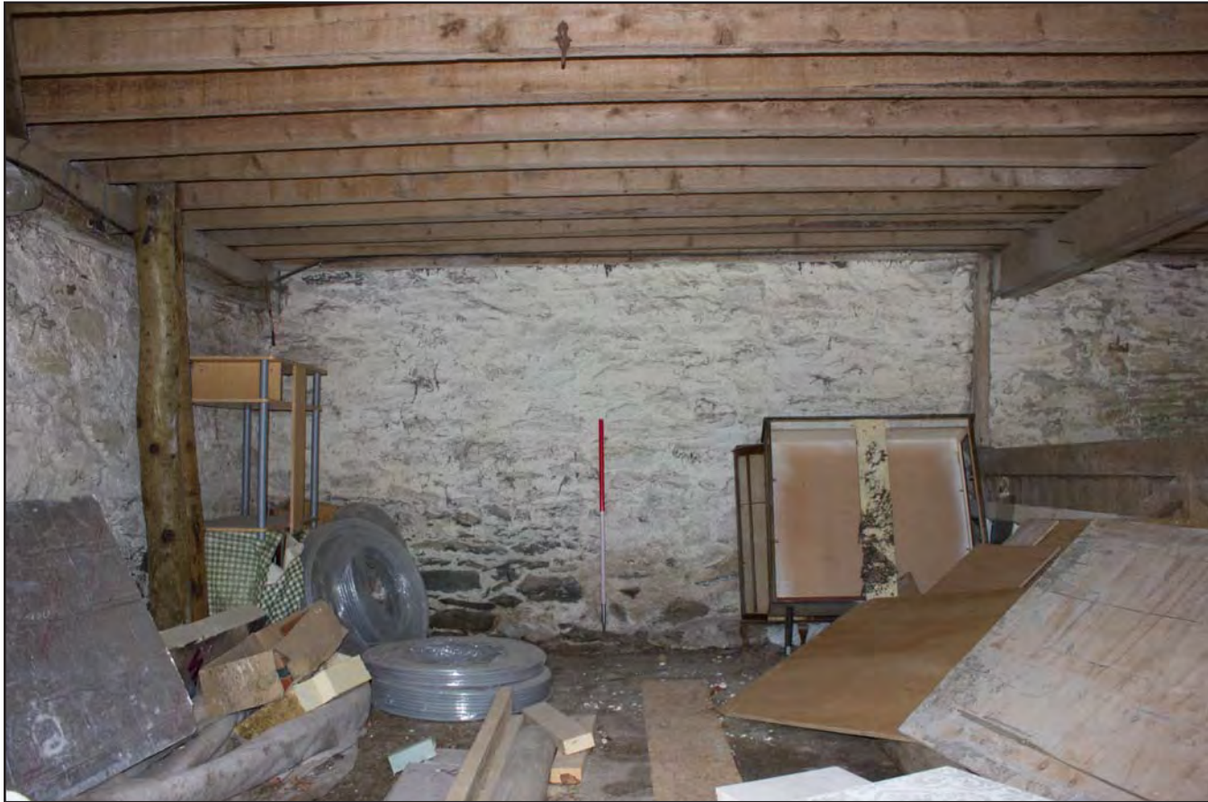
Plate 14: Former threshing floor (south western room) within Building 1 - Cart and Threshing Barn at Gaer Gerrig, Llangwm, Conwy - from the southeast - 1.00m scale
