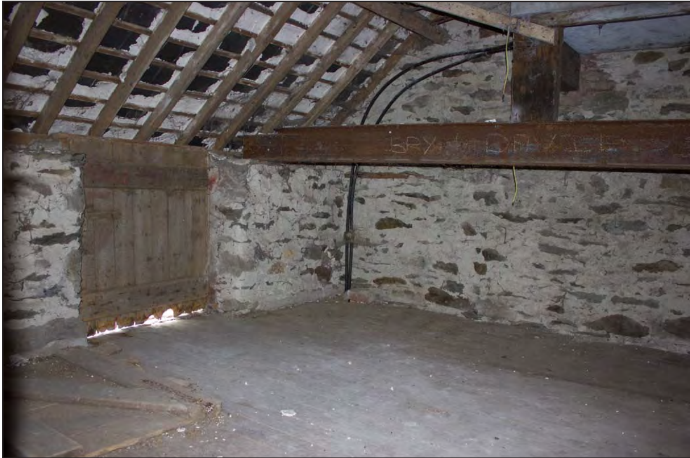
Plate 23: Store 3, First Floor, within Building 1 - Cart and Threshing Barn at Gaer Gerrig, Llangwm, Conwy - from the west - 1.00m scale
