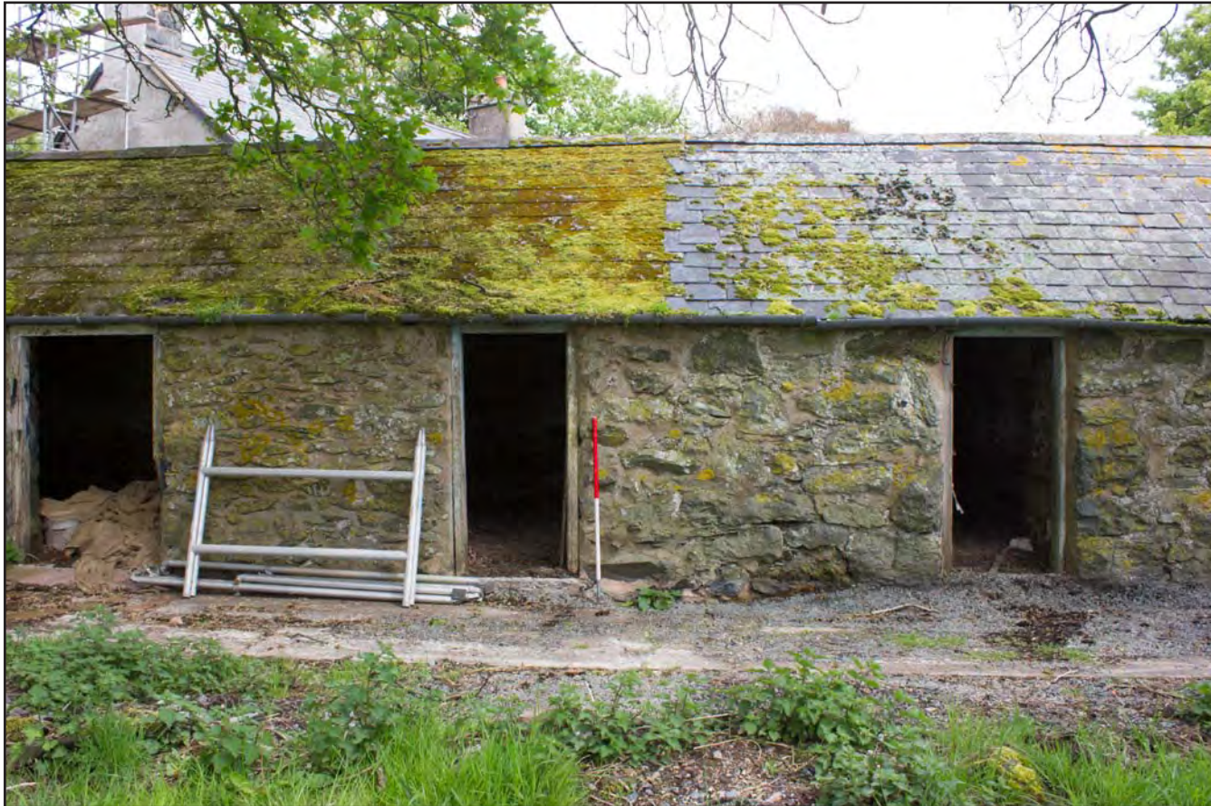
Plate 39: Southwest elevation (centre) of Building 3 - Pigsties at Gaer Gerrig, Llangwm, Conwy - from the southwest - 1.00m scale
