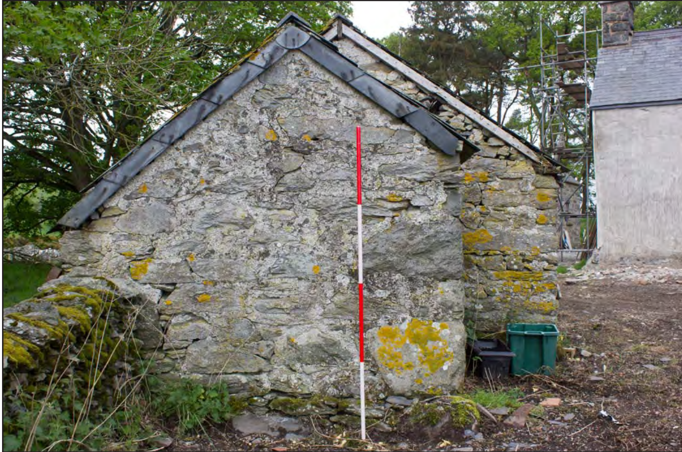
Plate 42: Southeast elevation of Building 3 - Pigsties at Gaer Gerrig, Llangwm, Conwy - from the southeast - 2.00m scale
