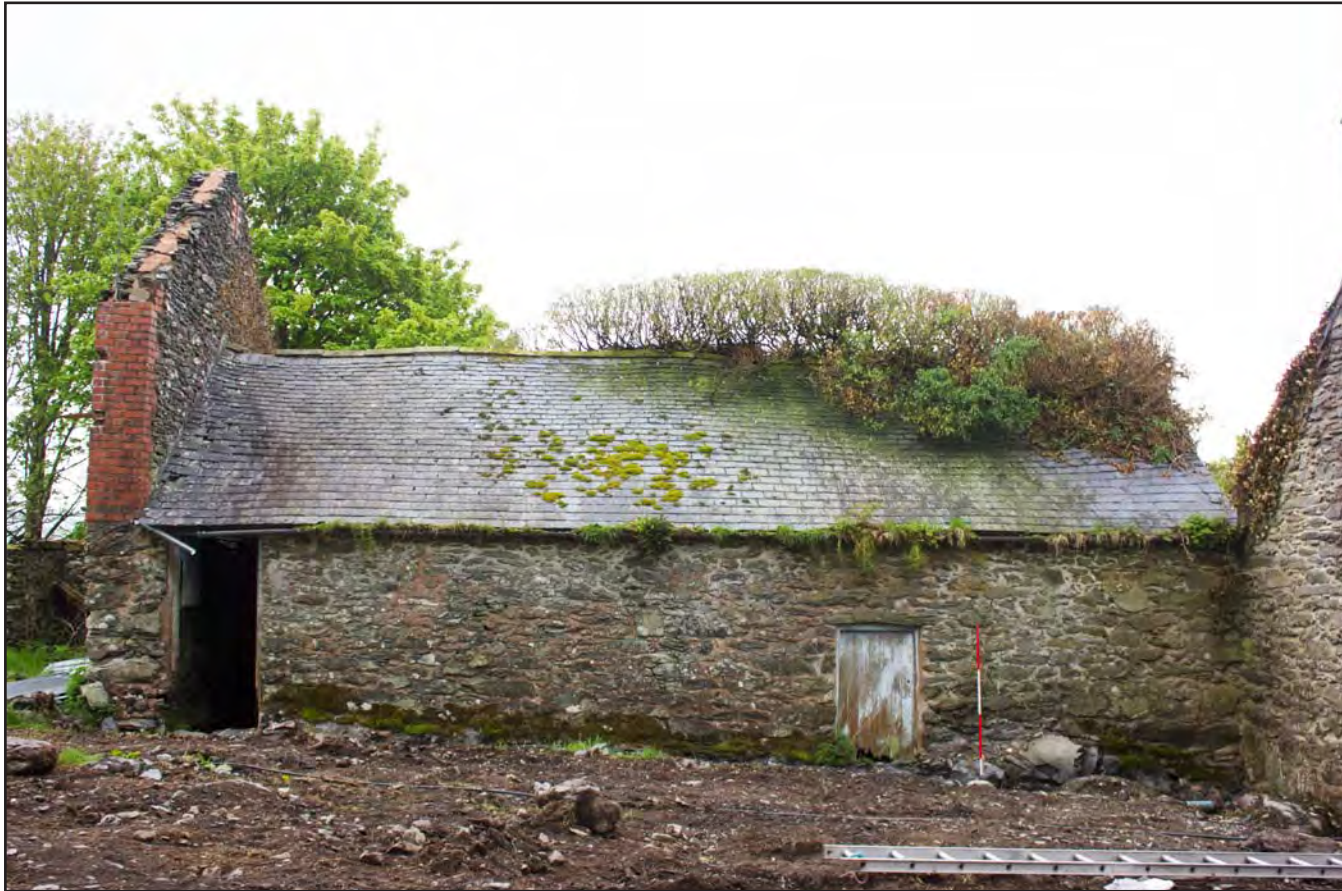
Plate 60: Northwest elevation of Building 4 - Cowhouse/Shippon at Gaer Gerrig, Llangwm, Conwy - from the northwest - 2.00m scale
