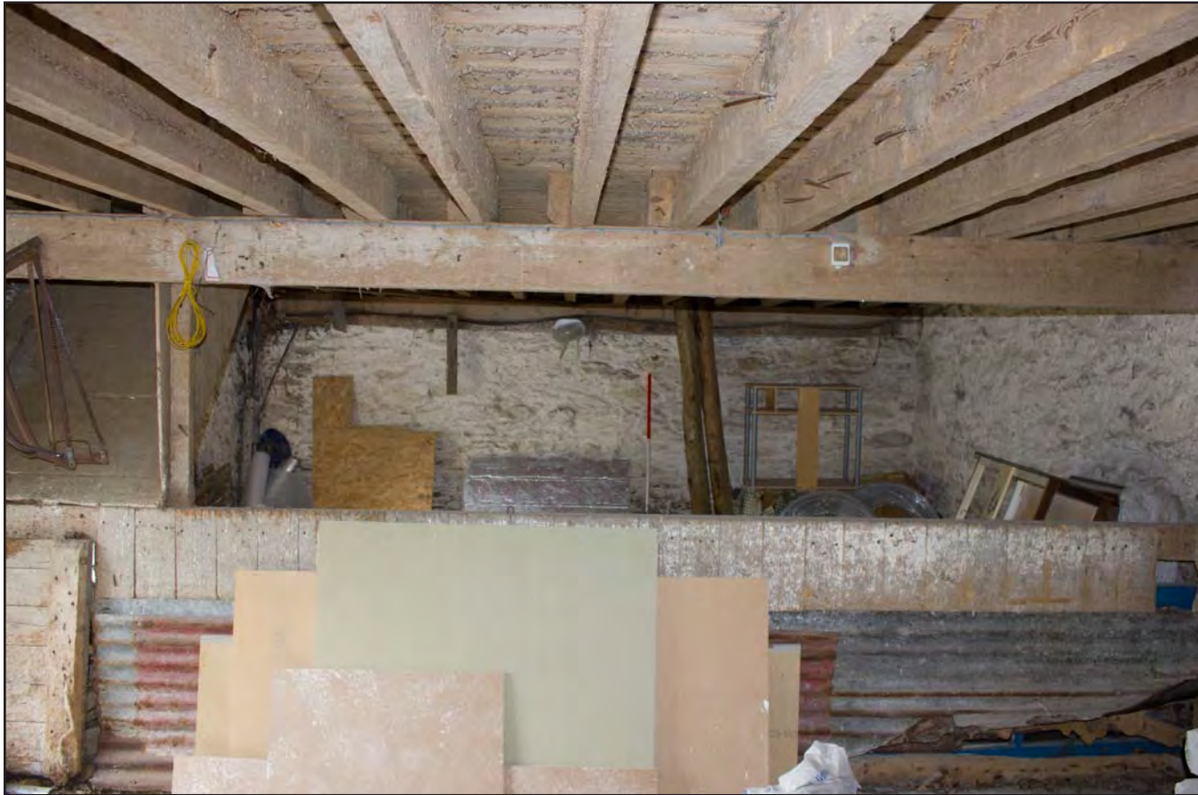
Plate 17: Former threshing floor within Building 1 - Cart and Threshing Barn at Gaer Gerrig, Llangwm, Conwy - from the northeast - 1.00m scale
