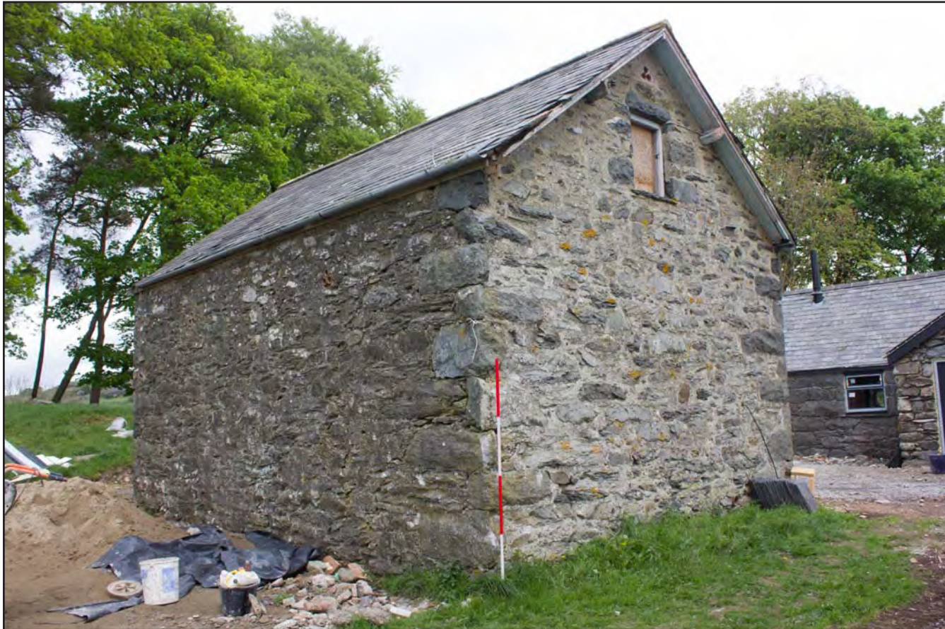
Plate 29: Oblique shot of southwest & southeast elevations of Building 2 - Horse/Pony Stable at Gaer Gerrig, Llangwm, Conwy - from the south - 2.00m scale
