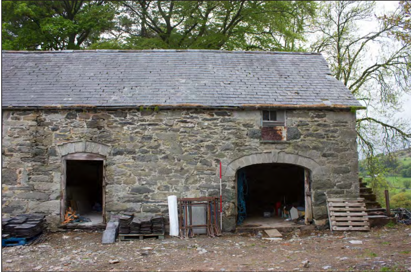
Plate 03: Southeast elevation (right) of Building 1 - Cart and Threshing Barn at Gaer Gerrig, Llangwm, Conwy - from the southeast - 2.00m scale
