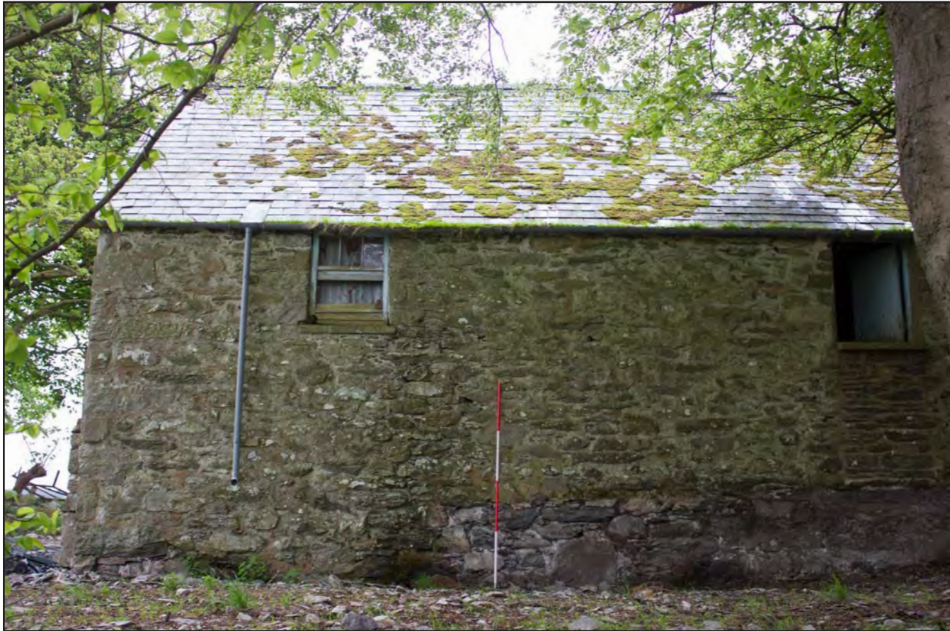
Plate 08: Northwest elevation (left) of Building 1 - Cart and Threshing Barn at Gaer Gerrig, Llangwm, Conwy - from the northwest - 2.00m scale
