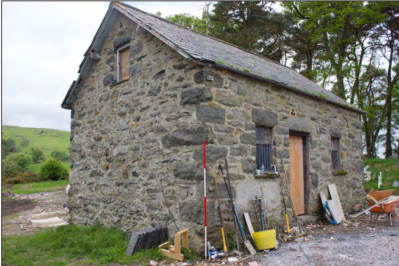
Plate 31: Oblique shot of southeast & northeast elevations of Building 2 - Horse/Pony Stable at Gaer Gerrig, Llangwm, Conwy - from the east- 2.00m scale
