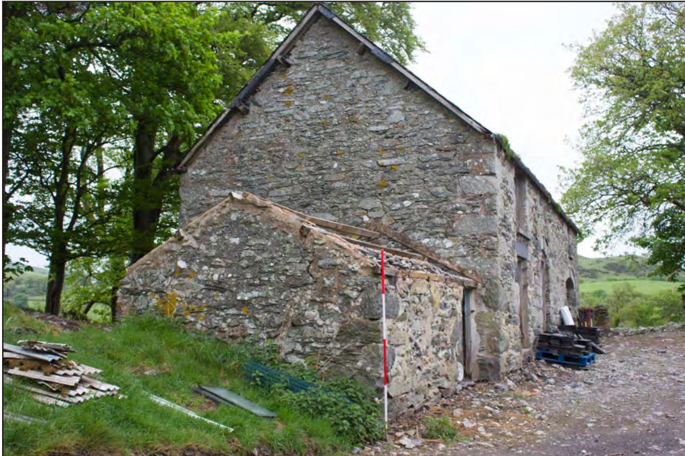
Plate 12: Oblique shot of southwest & southeast elevations of Building 1 - Cart and Threshing Barn at Gaer Gerrig, Llangwm, Conwy - from the south-southeast - 2.00m scale
