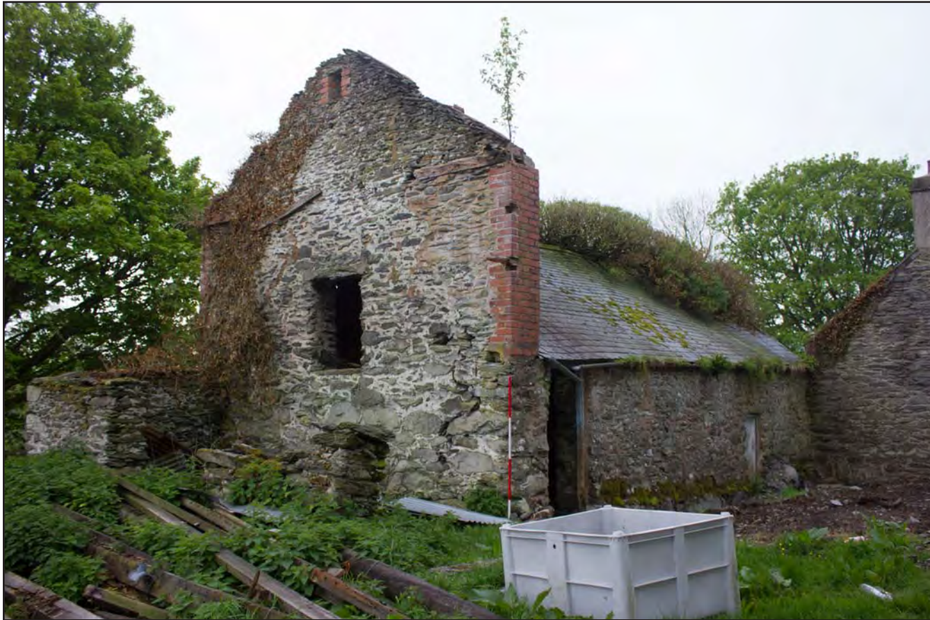
Plate 61: Oblique shot of northeast & northwest elevations of Building 4 - Cowhouse/Shippon at Gaer Gerrig, Llangwm, Conwy - from the east - 2.00m scale
