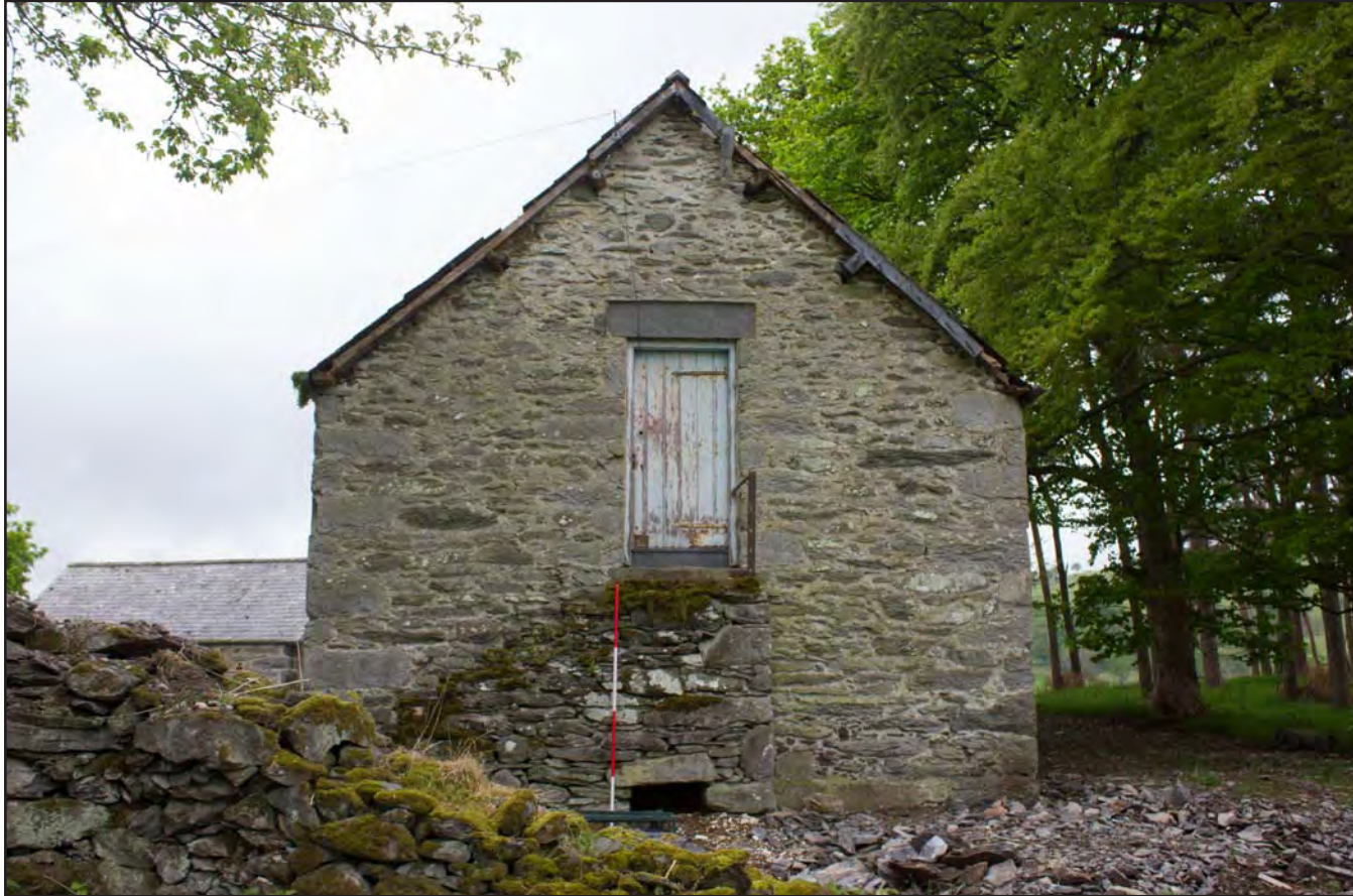
Plate 06: Northeast elevation of Building 1 - Cart and Threshing Barn at Gaer Gerrig, Llangwm, Conwy - from the north - 2.00m scale
