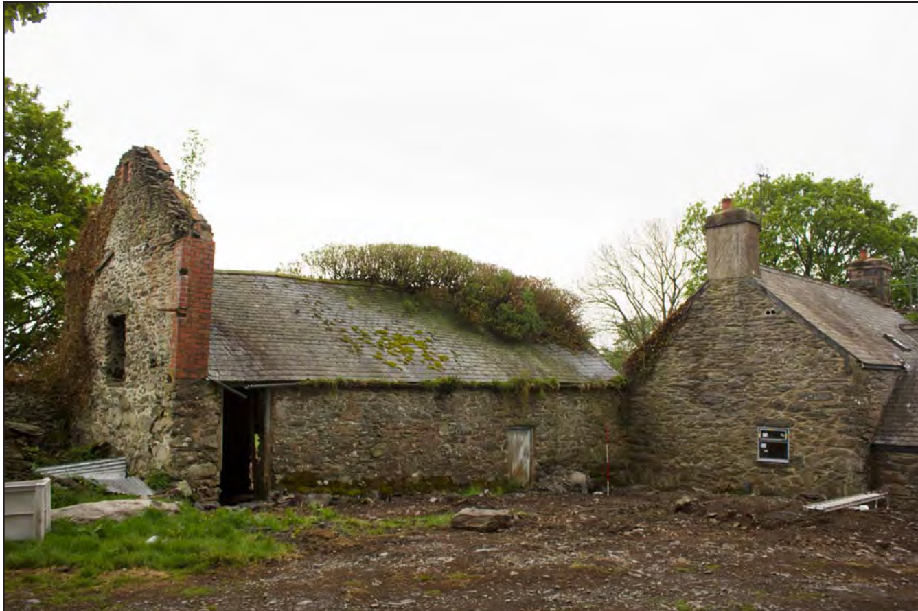
Plate 62: Context shot of Farmhouse and Building 4 - Cowhouse/Shippon at Gaer Gerrig, Llangwm, Conwy - from the north - 2.00m scale
