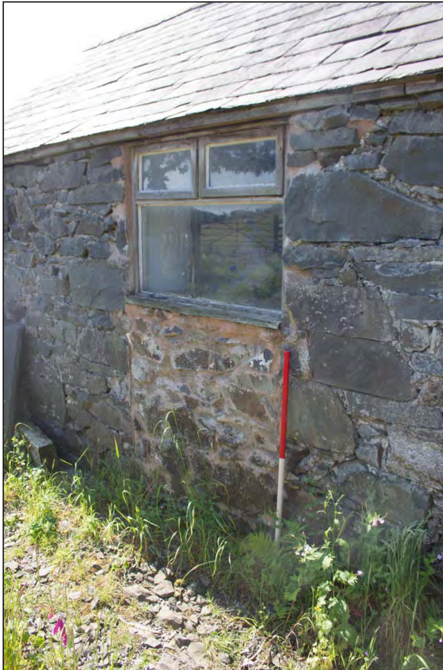
Plate 09: North facing external elevation showing blocked doorway, from the northwest. Scale 1.0m.
