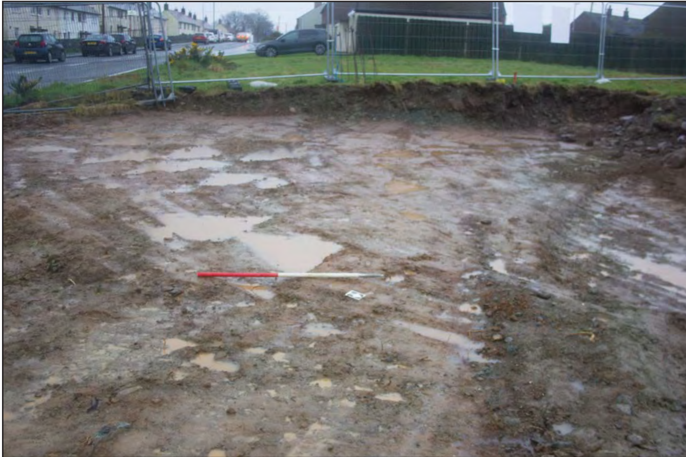
Plate 06: Stripped compound area at southwest end of Site, from the northeast. Scale 1.0m.
