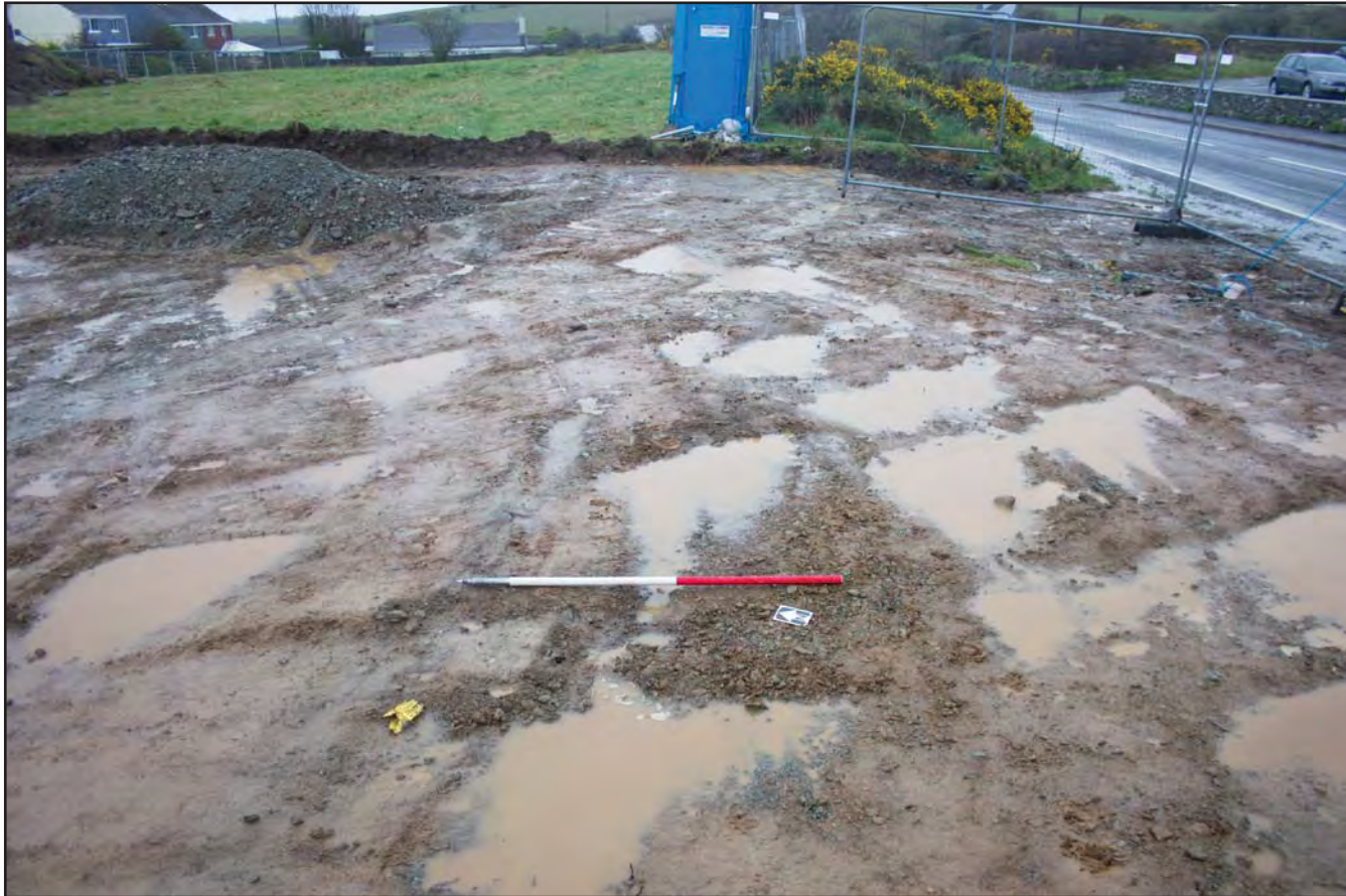
Plate 07: Stripped compound area at southwest end of Site, from the southwest. Scale 1.0m.
