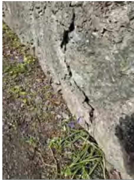
Detailed view of an area of cracking
