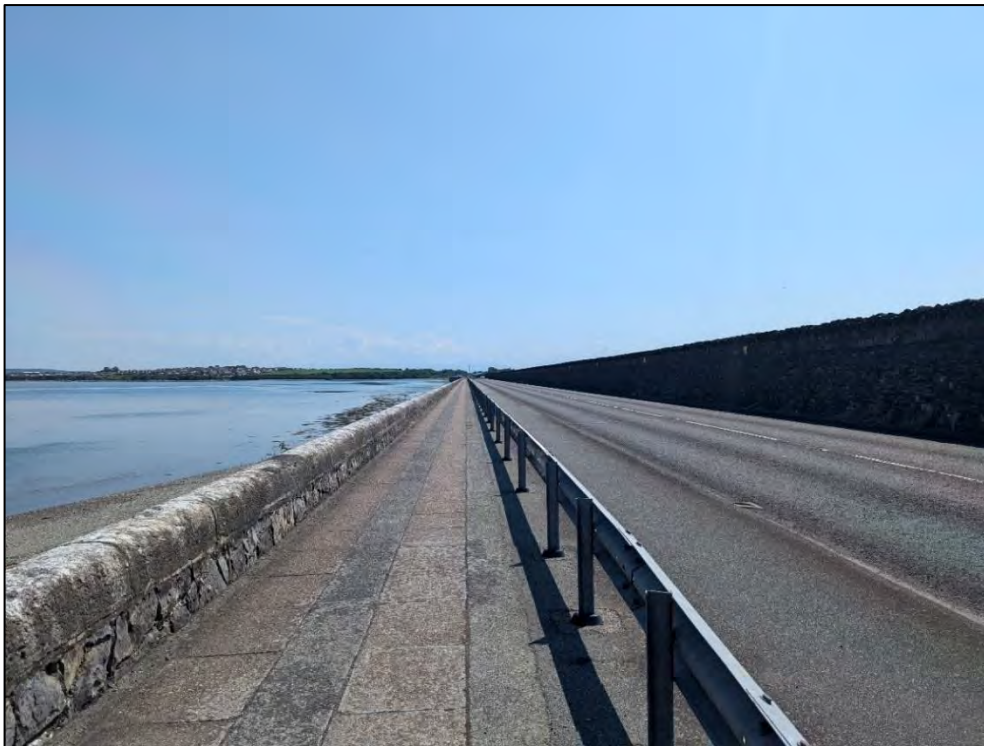
Figure 3 View facing south-east of Stanley Embankment (LB1) from the western extent of the proposed cable route.
