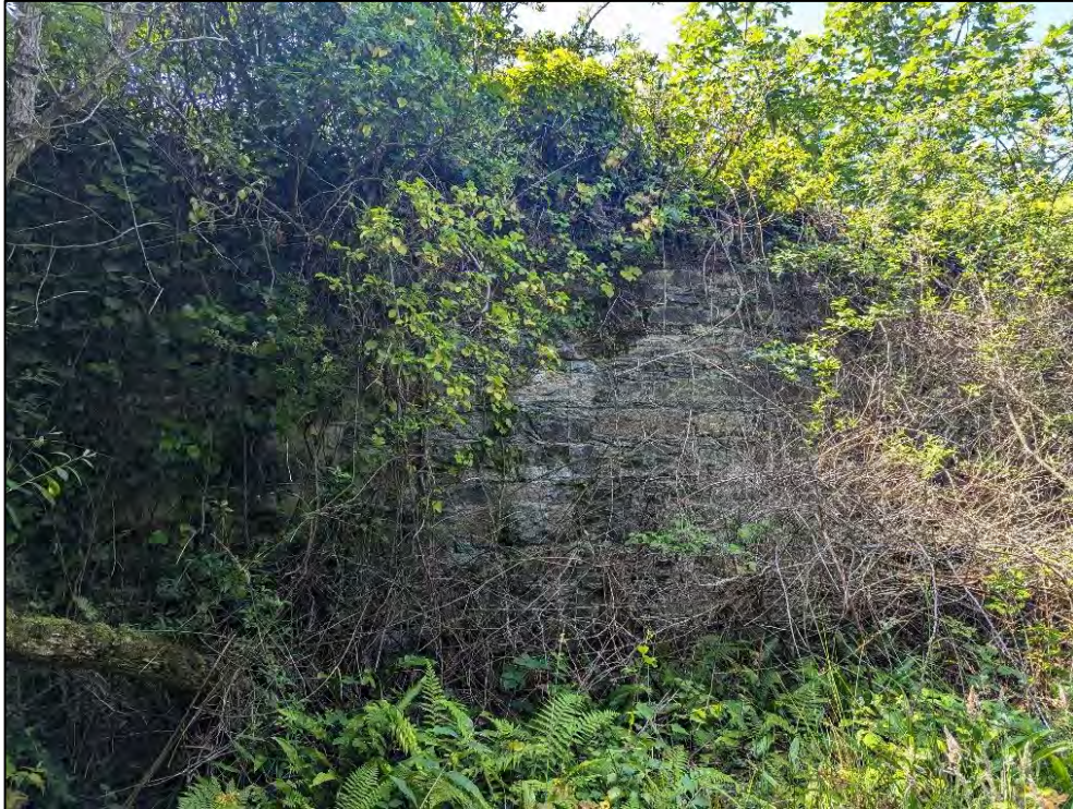
Figure 10 View of drystone wall, the upstanding remains of the section of Stanley Embankment Wall (NDHA19)
