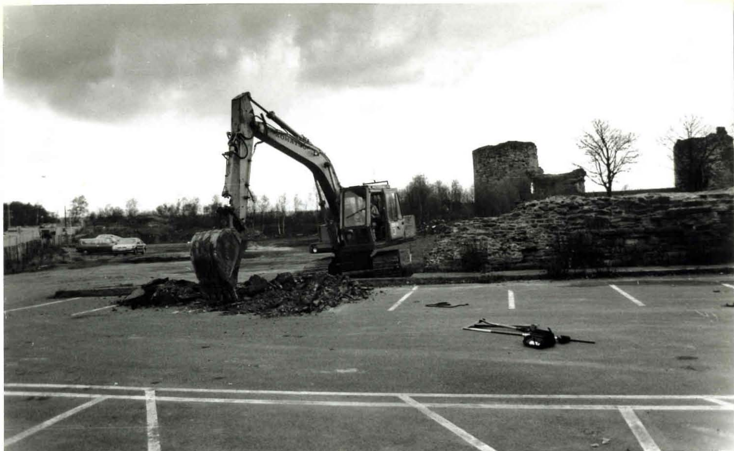
FIGURE 7: surface of carpark being removed by machine adjacent to the isolated stretch of sandstone wall to the southwest of the castle
