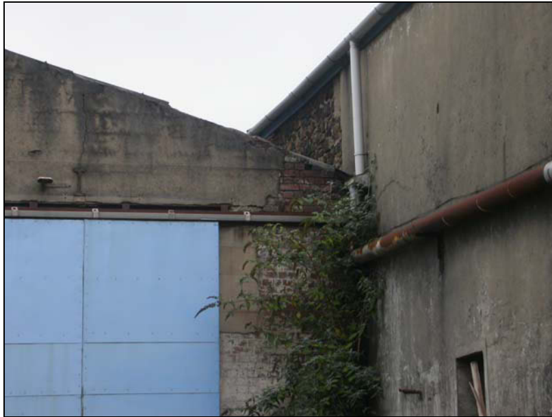
Plate 5. View of HMR3 showing differing construction of stone (central structure) and brick (structure adjoining to south)
