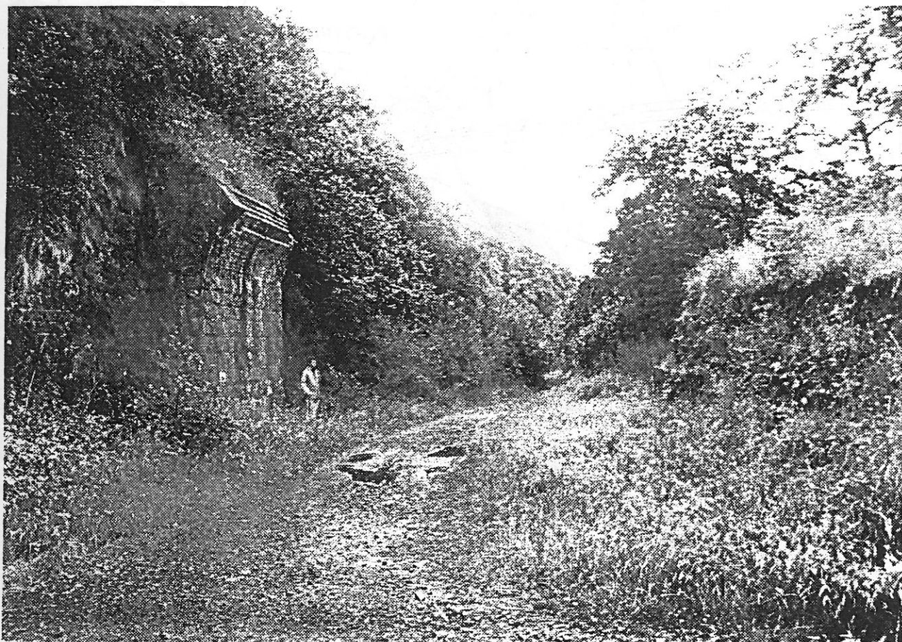
Course of Vale of Neath Railway: remains of footbridge near Blaengwrach, looking south.
