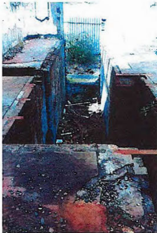
P28: Vivian Engine House. Unprotected drops, risk of falling structure.
