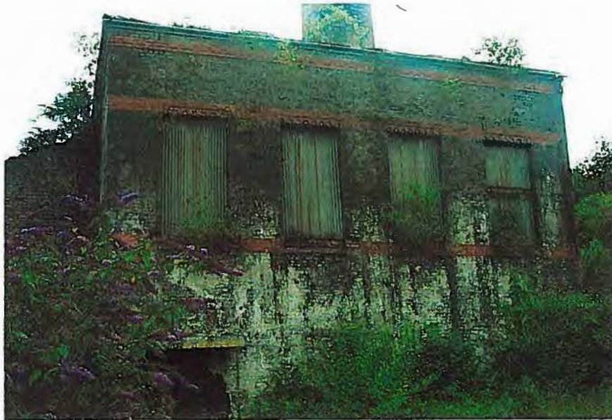
Left upper: north elevation, the large rectangular windows to the upper ground floor of the engine house have been boarded over.
