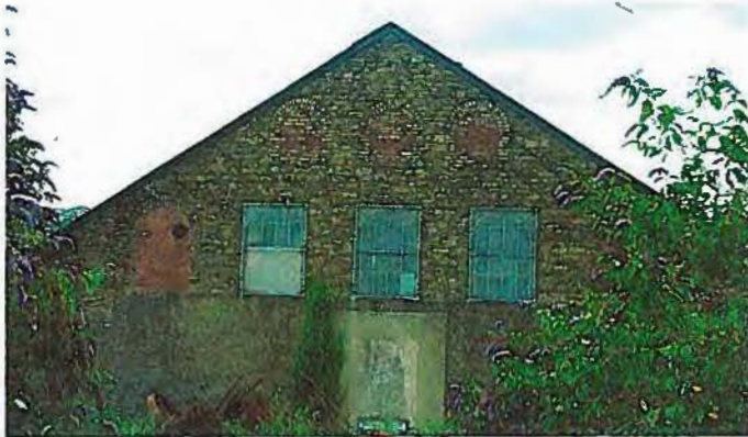
Left upper: south gable of the stores, five of the original eight windows have been bricked in.
