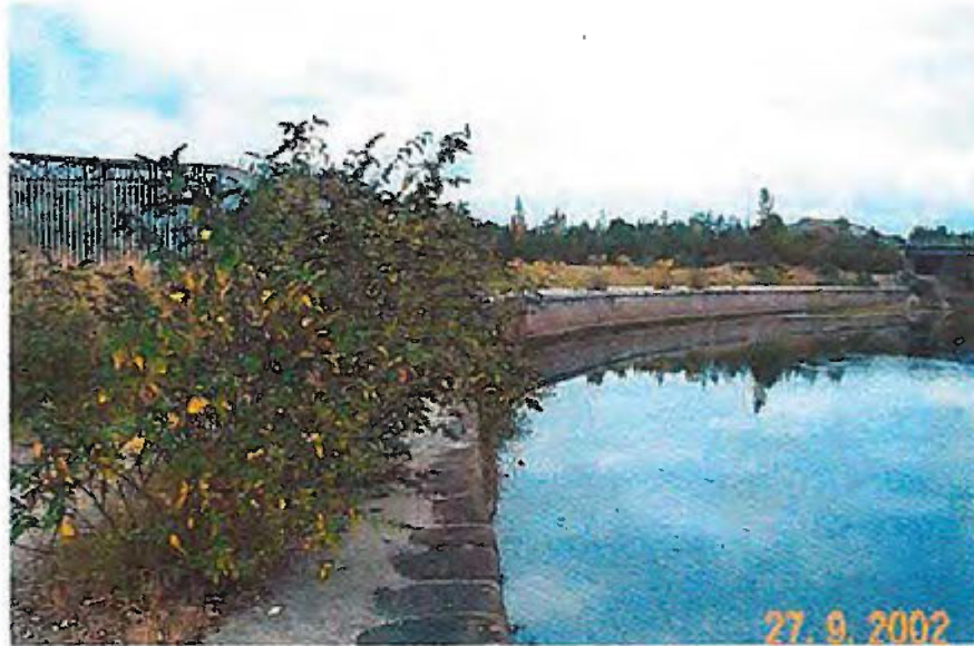
P15: Unprotected drop to River Tawe.
