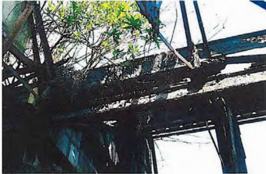
P35: Dilapidated condition of roof structure to Locomotive Shed
