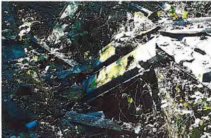
P40: Broken asbestos sheets lying in Locomotive Shed
