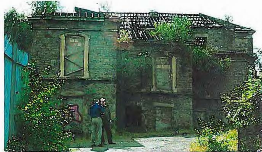
Right upper: east elevation, the centre portion has subsided towards its north corner causing cracking and distortion of stonework, most pronounced in the sills and lintols of window openings.
