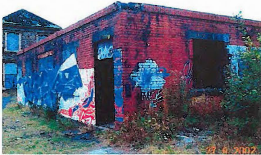
P23: Flat roofed building adjacent to Laboratory building. Unauthorised entry and building debris – trip hazard.
