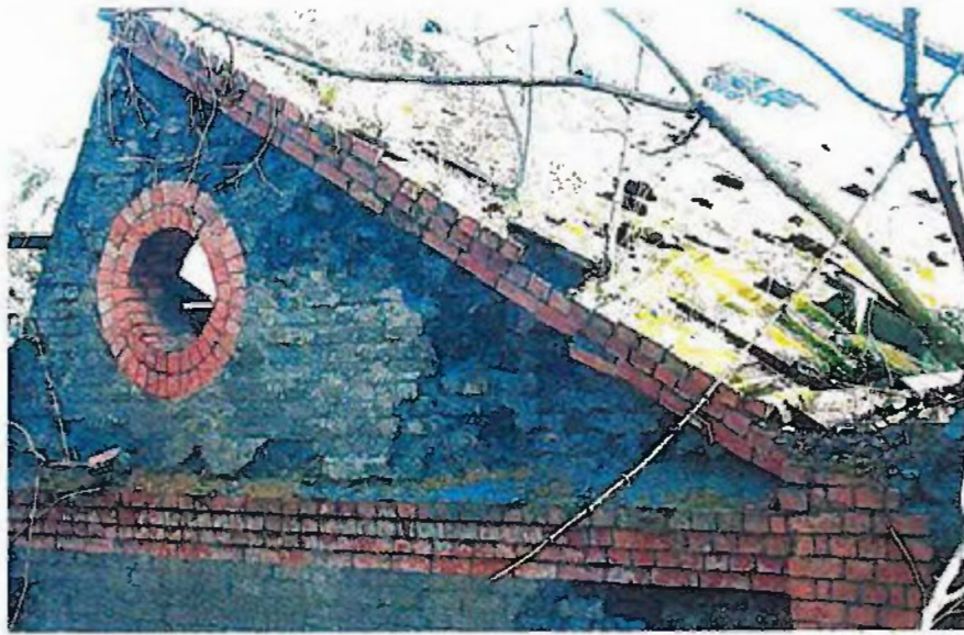
P37: Poor condition of brickwork to Locomotive Shed
