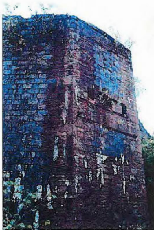
P25: Copper slag abutment and adjacent walls. Unprotected drop from the wall, risk of falling masonry.
