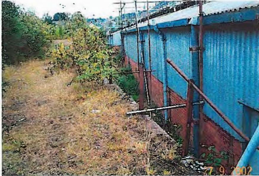
P1: Unprotected drop at structure 10.
