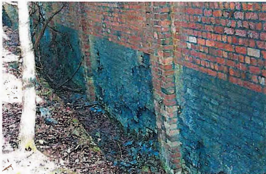
P30: Unprotected drop to rear of Locomotive Shed
