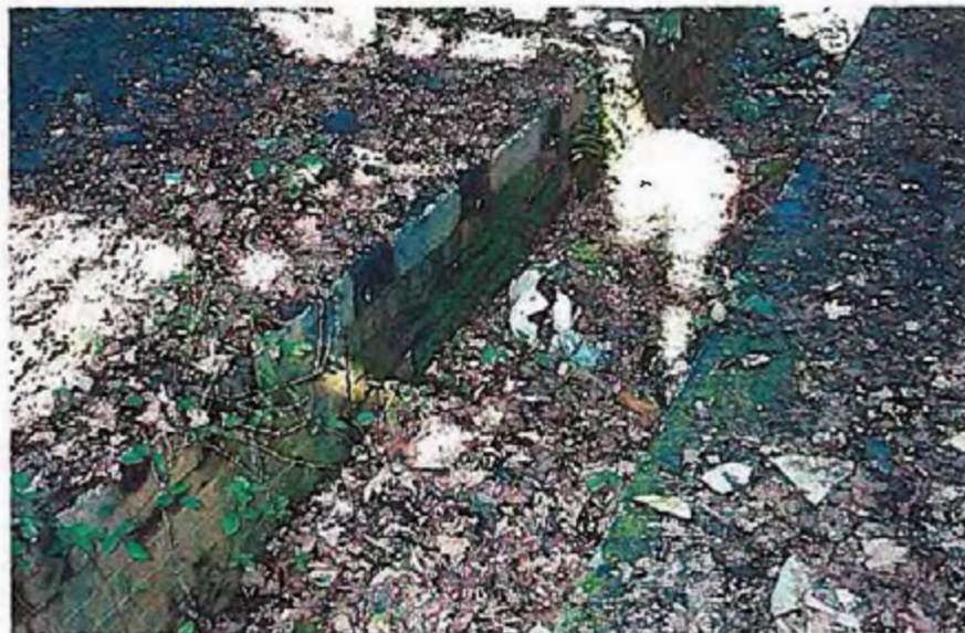
P32: Unprotected drop to pit in Locomotive Shed
