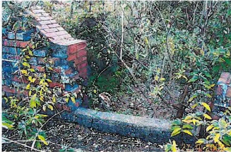
P7: Unprotected drop to west of structure 1.
