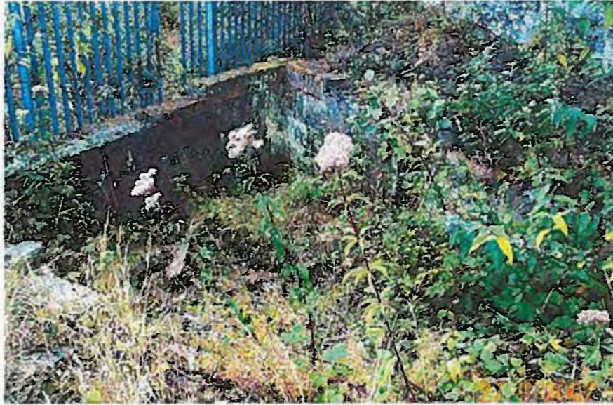
P9: Unprotected drop (pit) to south of structure 2.
