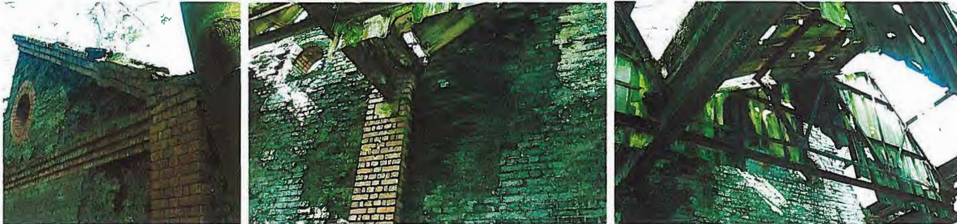
Above left: brickwork deterioration and roof structure failure has caused several of the gables to lean outward resulting in the loss of brickwork from the cornices.
