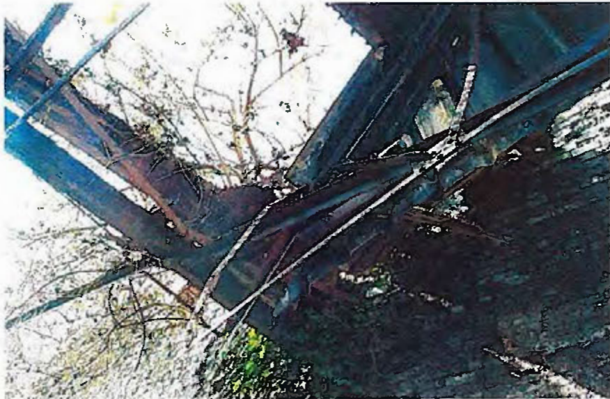
P34: Dilapidated condition of roof structure to Locomotive Shed
