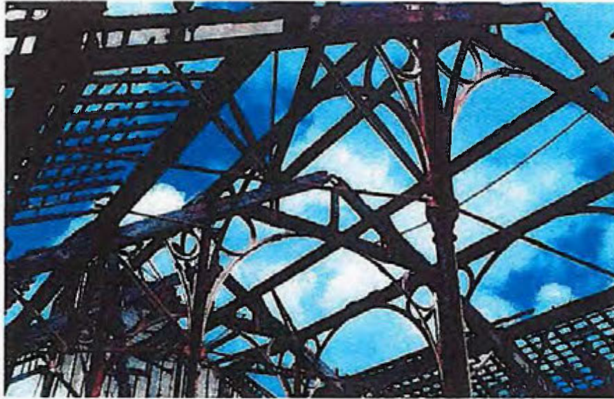
P27: Former Canteen Building. Risk of falling structure.
