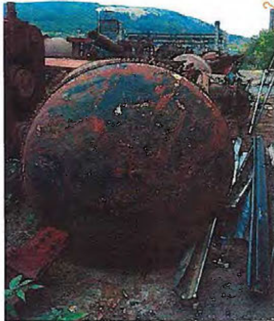
P6: Stored material adjacent structure 10.
