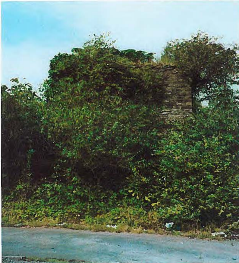
Above: South face of the lime kiln viewed from the adjoining car park. The kiln is constructed of random rubble masonry and is heavily overgrown, in particular on the north face.
