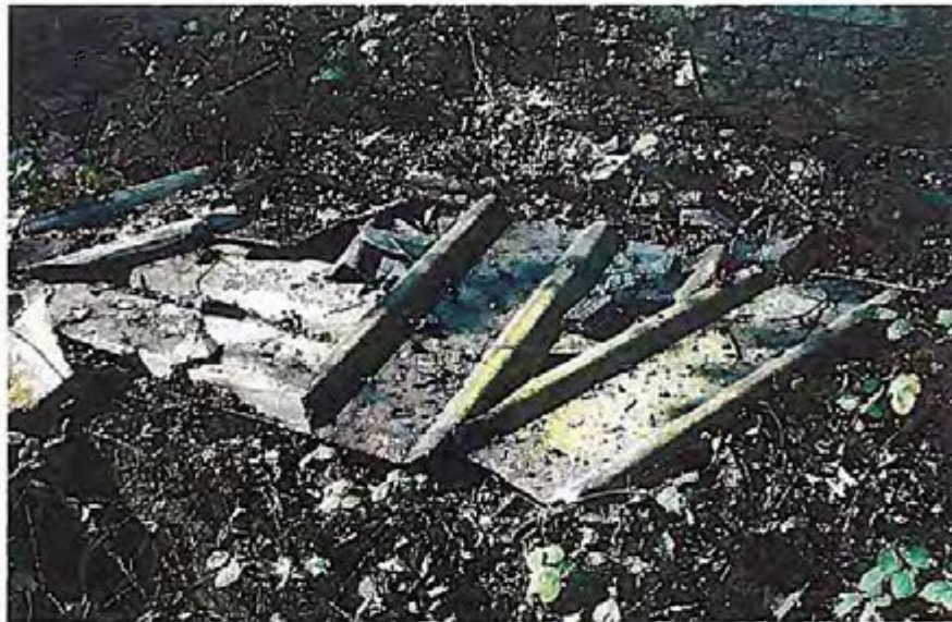
P39: Broken asbestos sheets lying in Locomotive Shed
