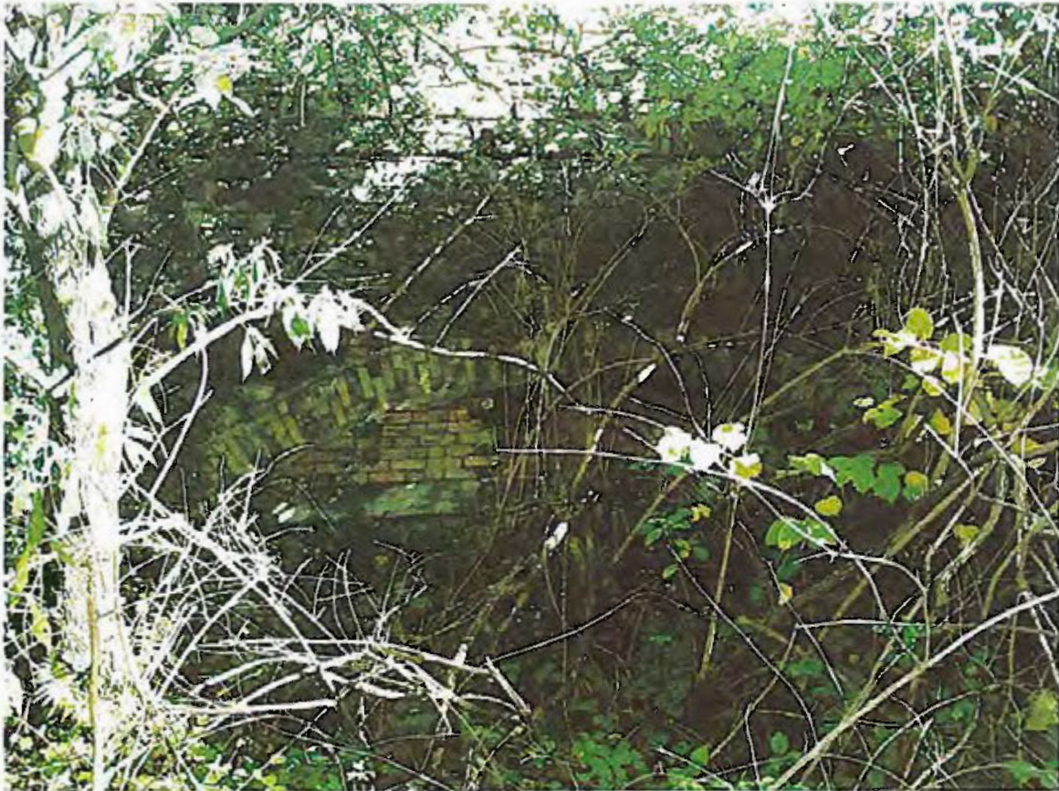
Photo 7 - Building 6.0 (Hafod canal boundary wall) from the west, showing blocked archway to canal basin YIM 20
