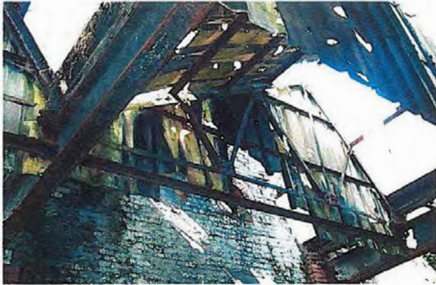
P33: Dilapidated condition of roof structure to Locomotive Shed
