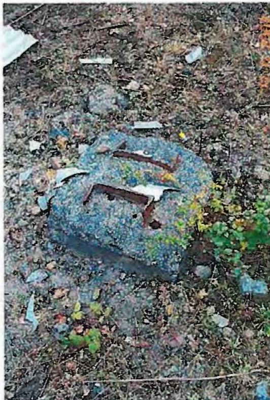
P2: Protruding column at structure 10.
