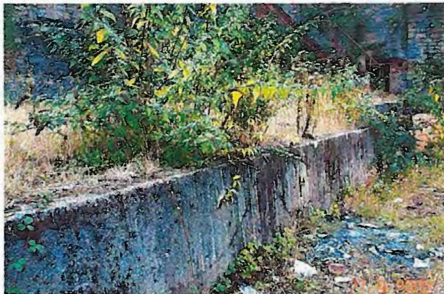
P8: Unprotected drop to south of structure 2.
