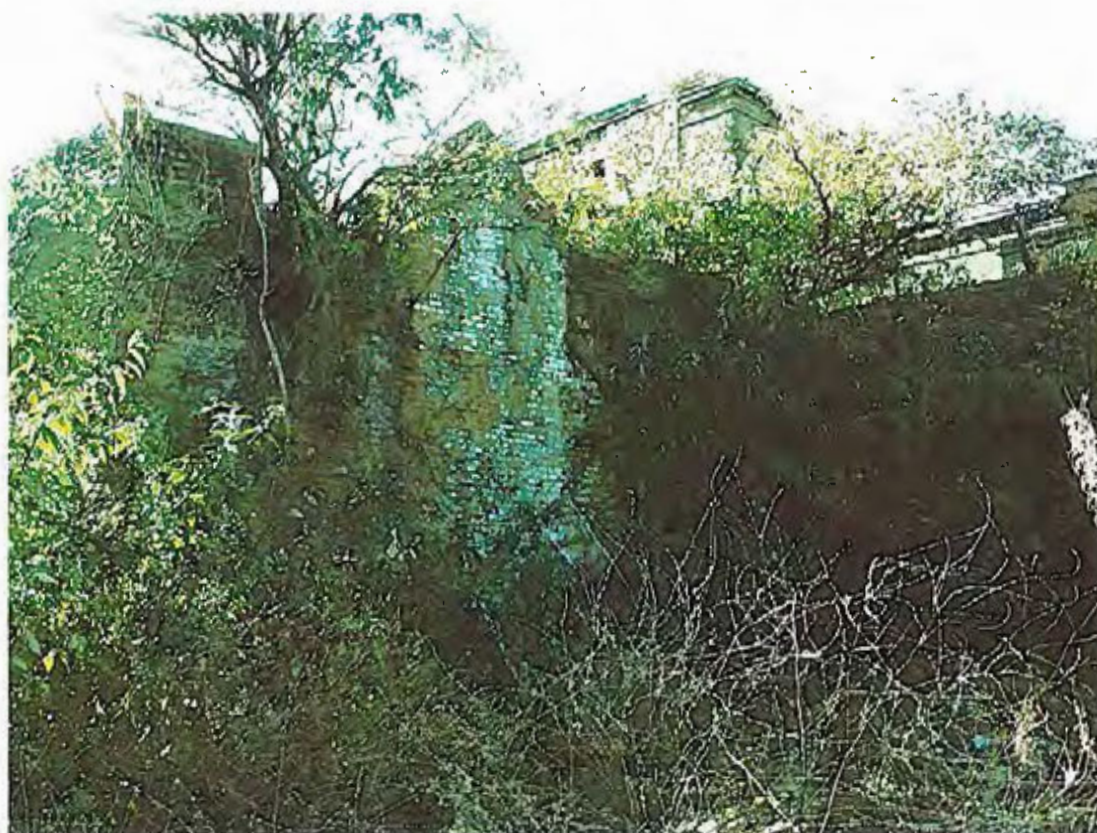
Photo 11d - Area 1E, south wall of YIM 28 and revetment wall YIM 8 from the NE
