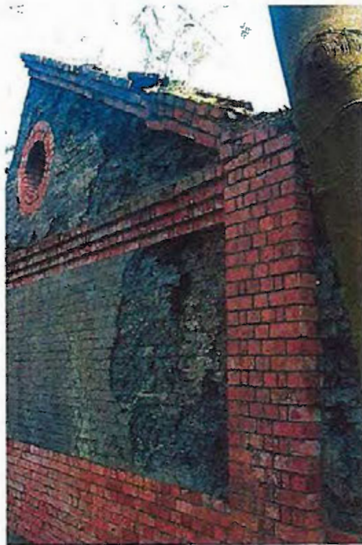
P38: Poor condition of brickwork to Locomotive Shed
