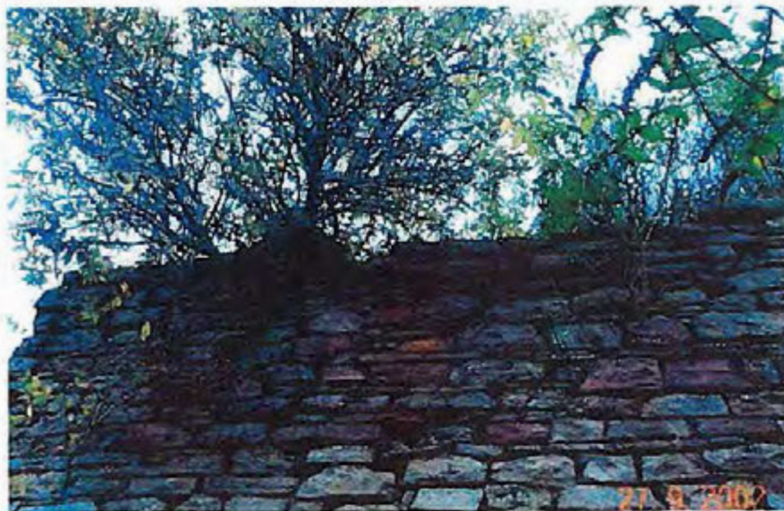
P26: Lime Kiln. Risk of falling masonry.
