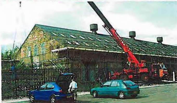
Left centre: view of east elevation with over-cladding of the roof in progress.
