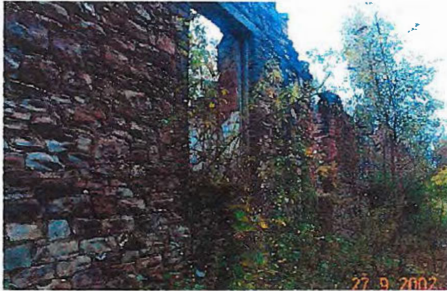
P21: Former Copperworks boundary wall. Risk of falling masonry.
