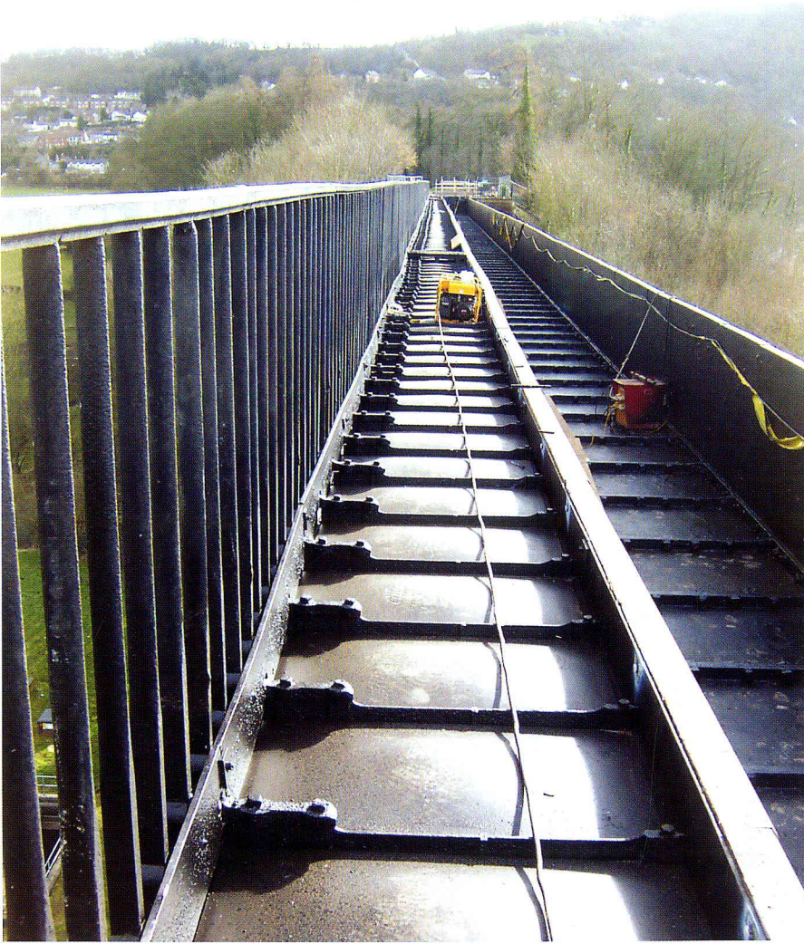
The cast-iron trough was drained while contractors carried out the conservation work
