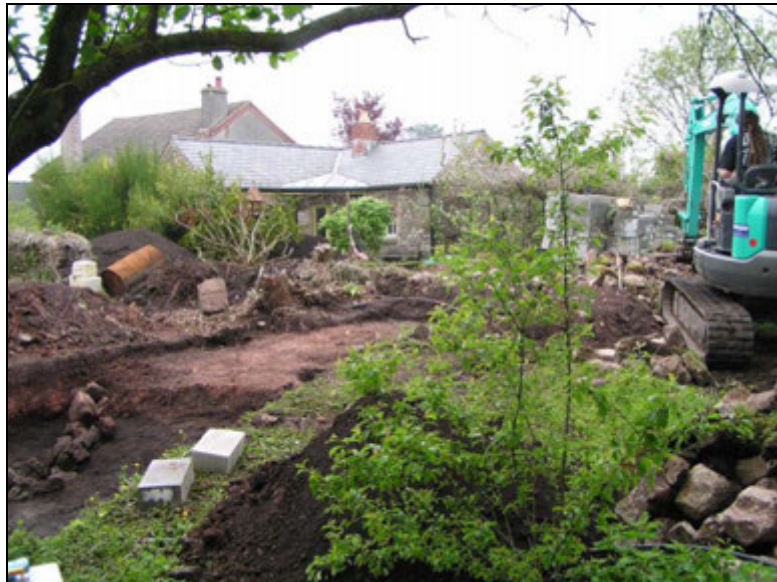
The evaluation area showing Trench 1 to the left of foreground. View to the north © GGAT
