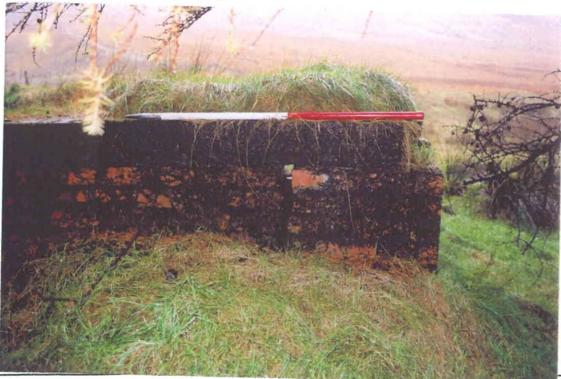
BELOW: CRACK AT S END OF W WALL
