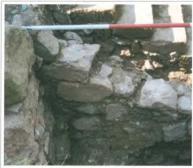
Figure 21 The stair wall [33] with terrace [32] to left and treads [35] behind. The section to the right has been altered and the cut into its footings is visible at bottom right. In the shadows next to the stairs brick rubble and mortar can be seen under the stone treads
