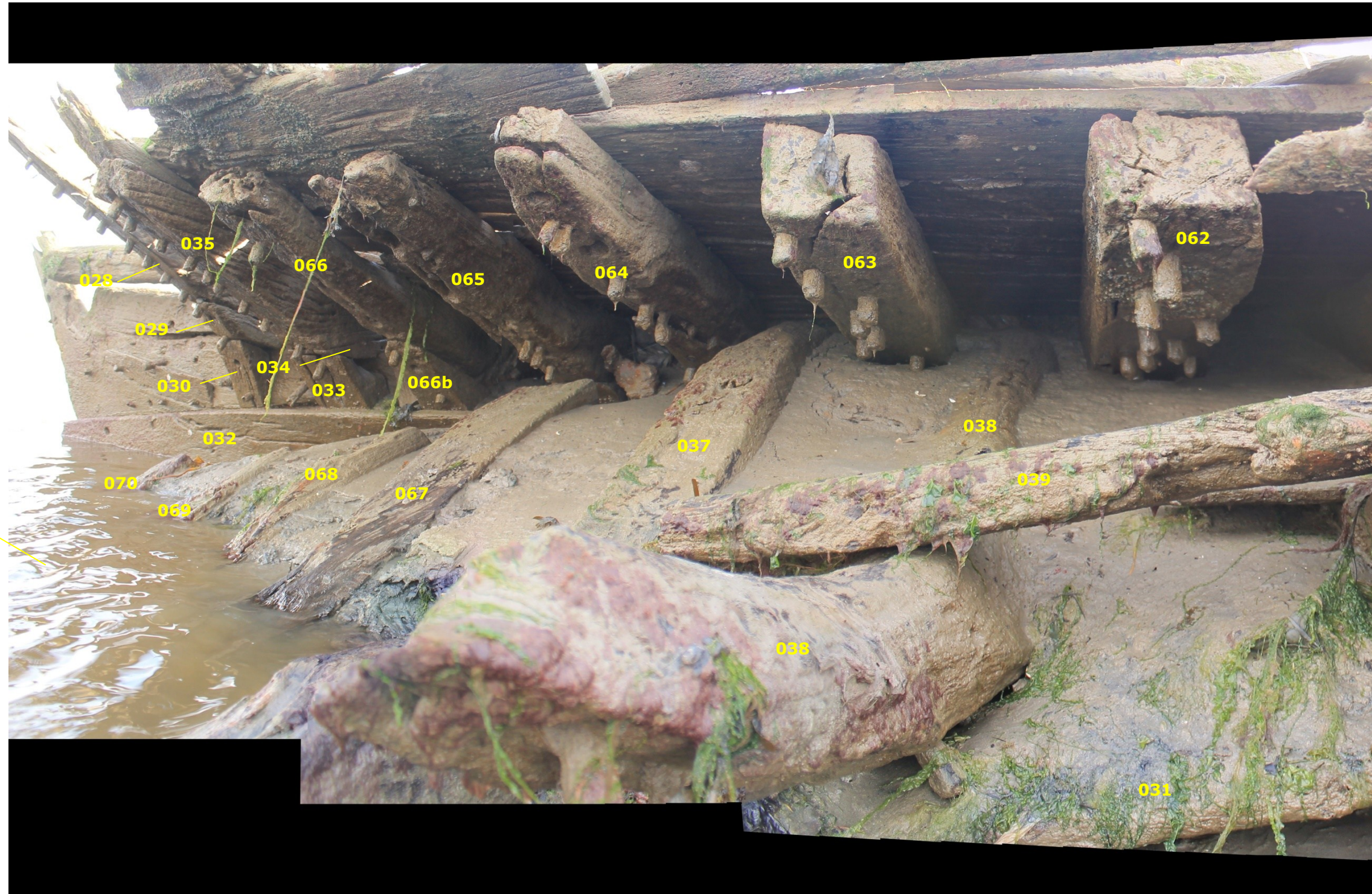
Photo 10: Frames on the starboard side (between Photo 11 and stern, Photo 9) (merged photographs from June 2015)
