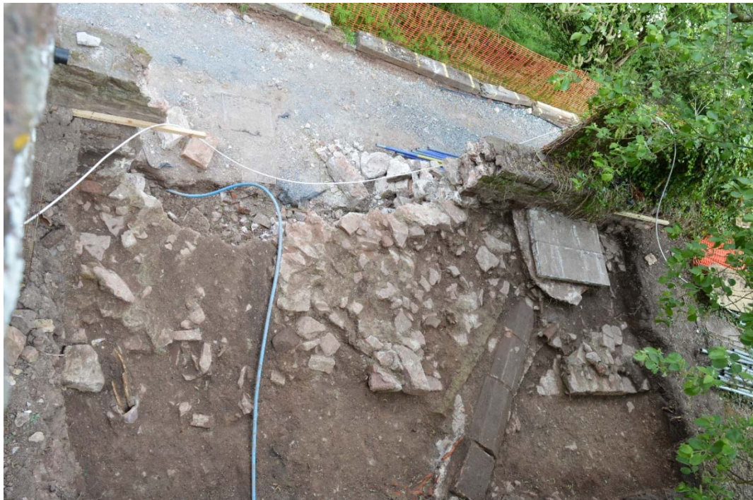
Fig. 5 The upper part of the medieval curtain wall showing recent disturbance by service trenches, viewed from the roof of the adjacent kitchen wing.
