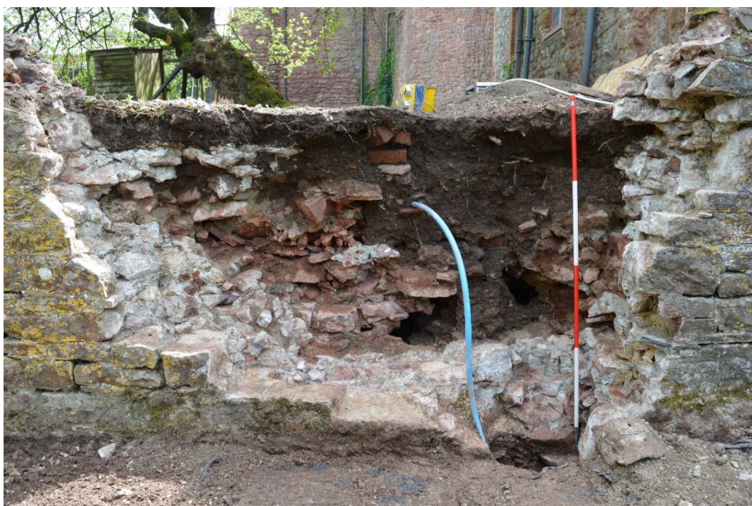
Fig. 4 The red conglomerate corework of the medieval curtain wall was gradually uncovered as the retaining wall was removed
