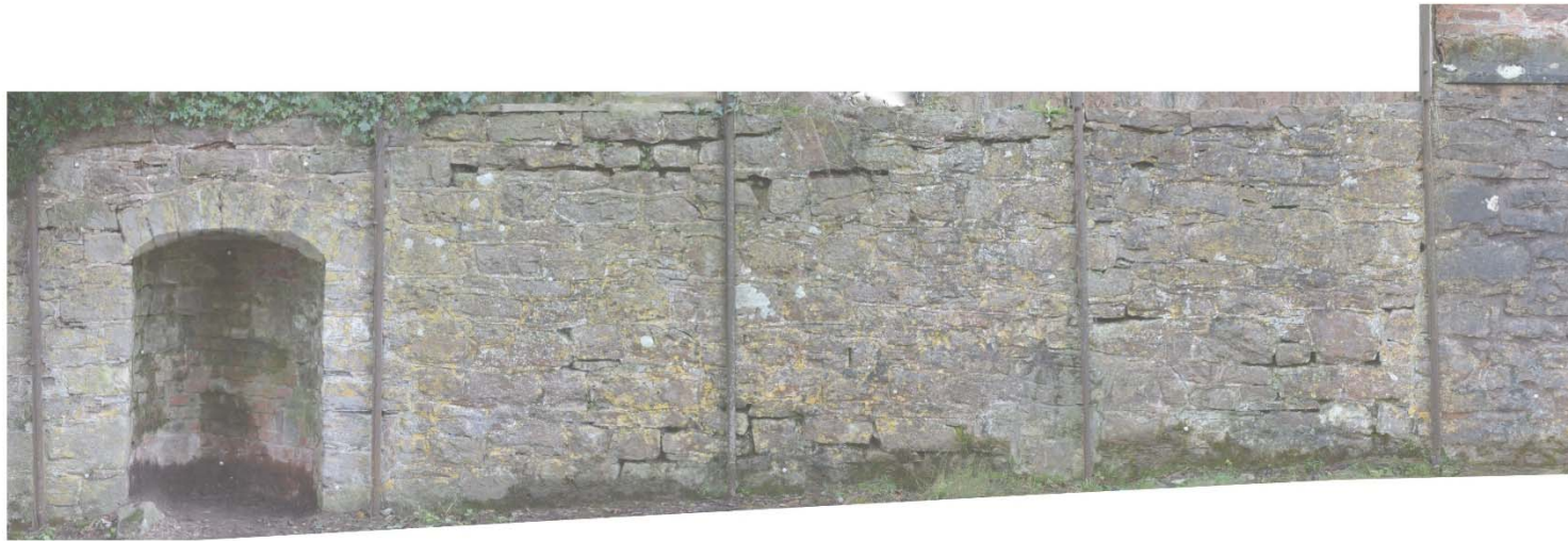
Fig. 11 Rectified photograph and stone-for-stone survey of the section of retaining wall on the north-western side of the Old Bowling Green
