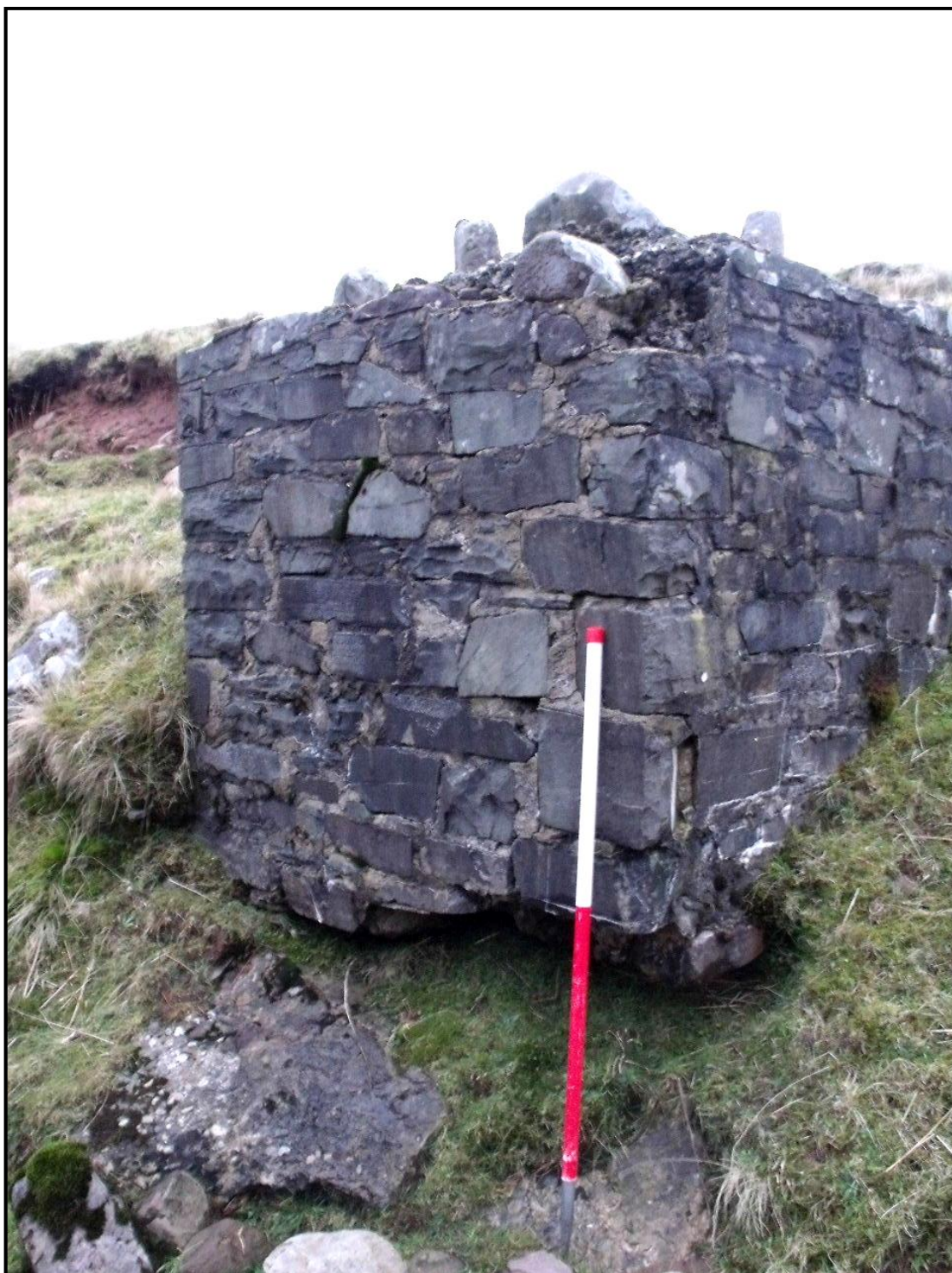
Photo 73. Typical undercutting by water of the anti tank blocks of BR337F CPAT 3798-0041
