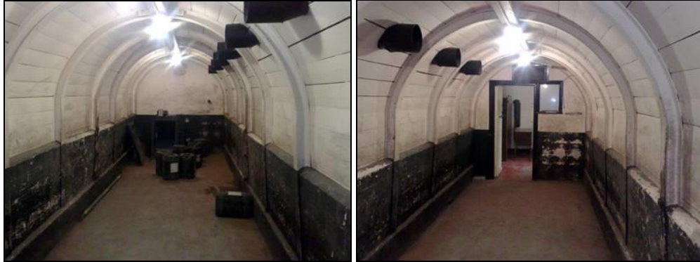
Humidity gallery with smoke inlets
