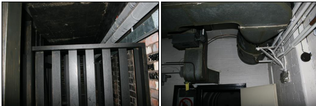
Section of gallery adapted by Fire Service Ductwork to smoke inlet system
