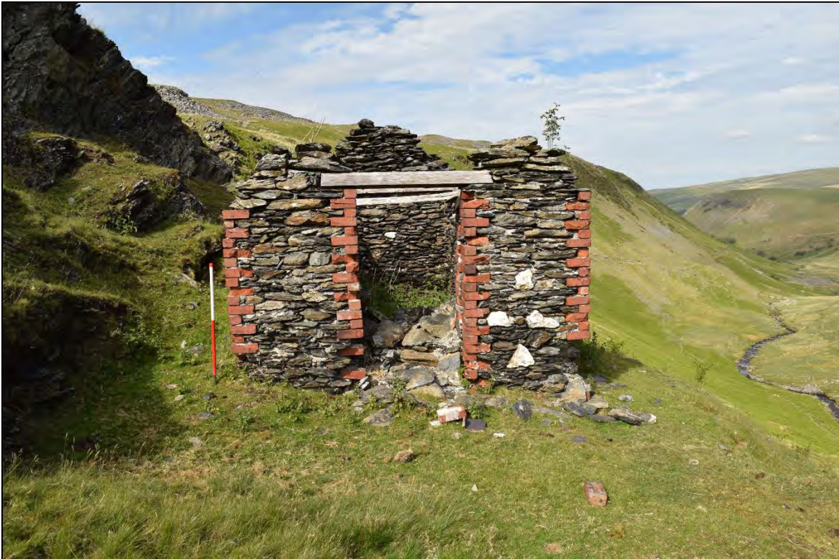
Plate 69: The Nant y Garw mine magazine building (ID number 804), high above the Rhiwnant valley. Looking northeast.
