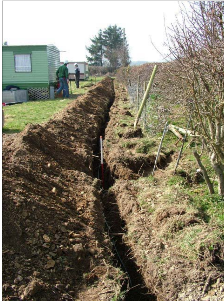
Fig. 4 View westwards along the cable trench, showing the position of the stanchion pit. Photo CPAT 2817.005
