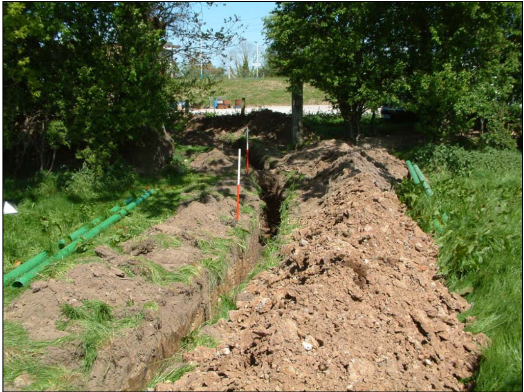
Plate 1 The curving pipe trench on western side of the hedge line. Scale rods mark the position of the edges of the ditch (5)
