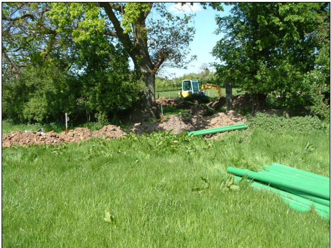
Plate 2 Pipe trench on western side of the hedge line viewed from south-south-west. Scale rods mark the position of the edges of the ditch (5)
