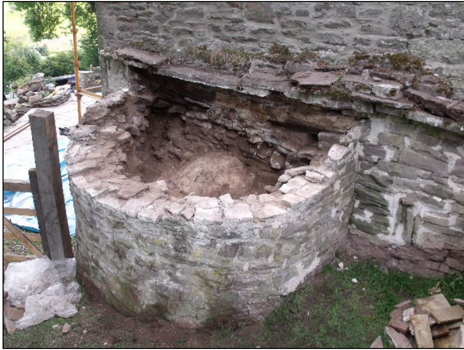
Fig. 2 The structure following the removal of infill, with the domed oven visible inside
