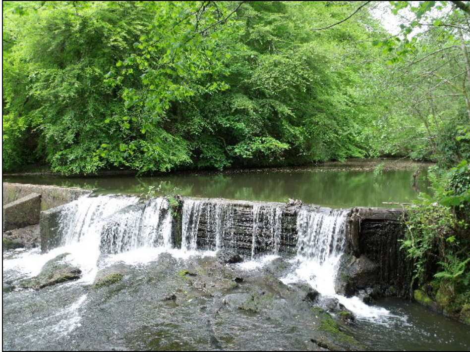
Fig. 4 The northern end of the weir showing the surviving original planking. Photo CPAT 3283.0001
