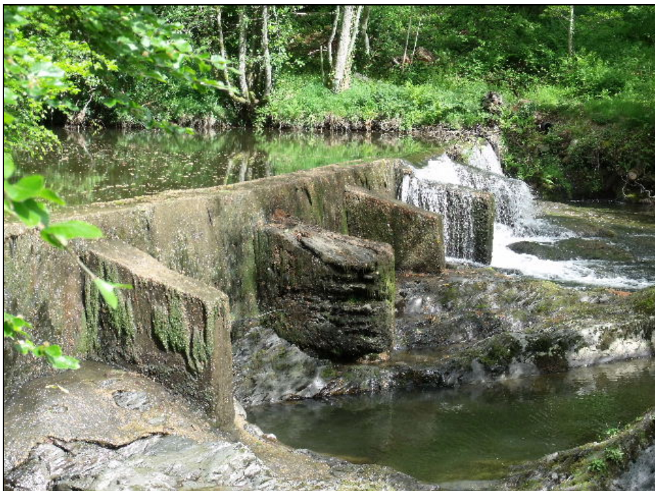
Fig. 5 The southern end of the weir showing the concrete section. Photo CPAT 3283.0015
