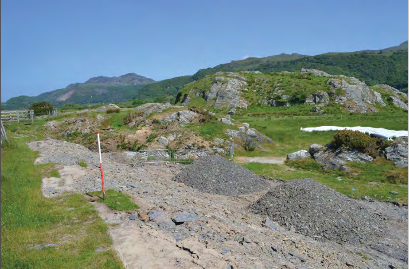
Plate 15: Stripped Topsoil showing clay and shale make-up of the embankment. View looking west. Scale 1m
