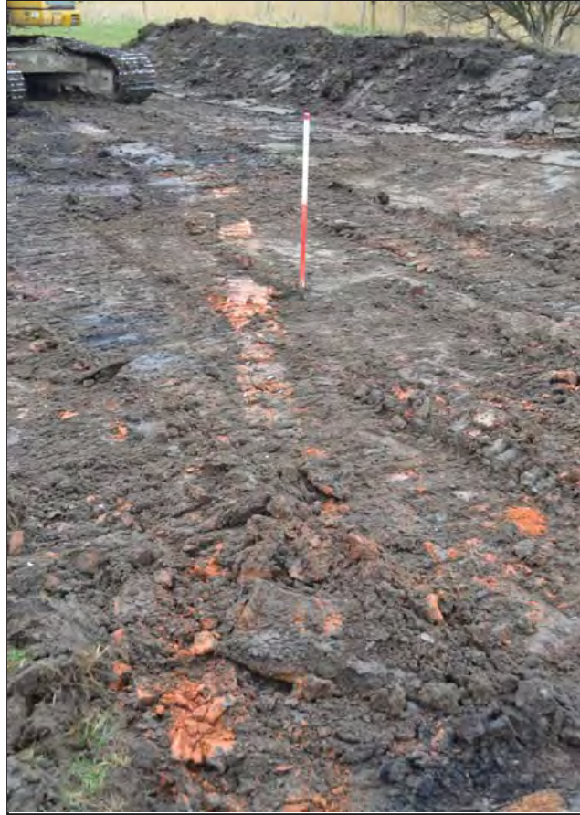
Plate 09: Excavation work on the borrow pit adjacent to the former brickworks site, showing double thickness of brickwork, which does not appear to be structural
