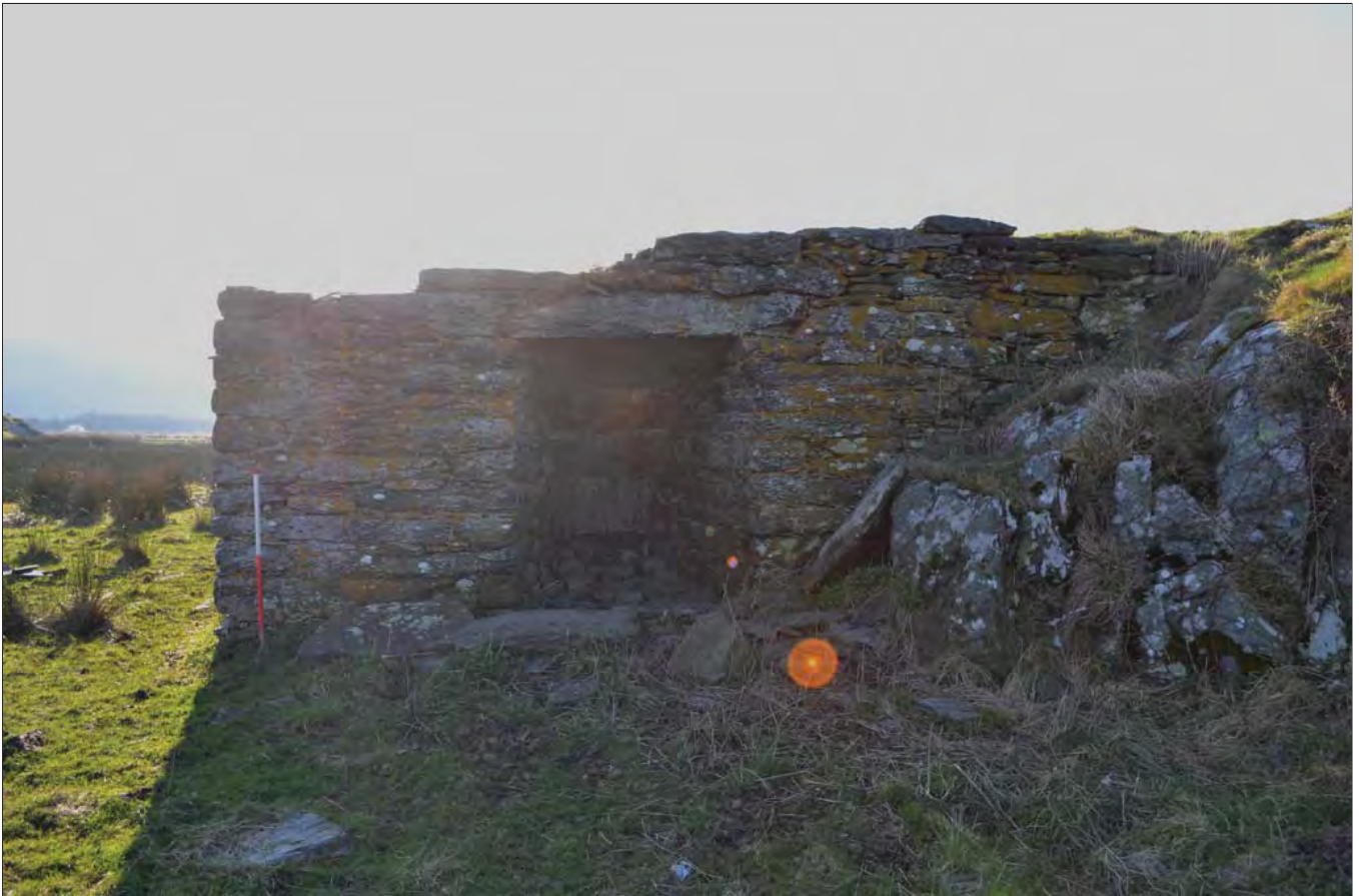
Plate 01: The Lime Kiln on the Fairbourne Embankment, viewed from the east. Scale 1m
