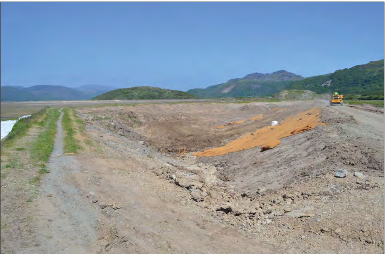
Plate 16: New section of Fairbourne Embankment removing the right-angled junction at the west end of the scheme.
