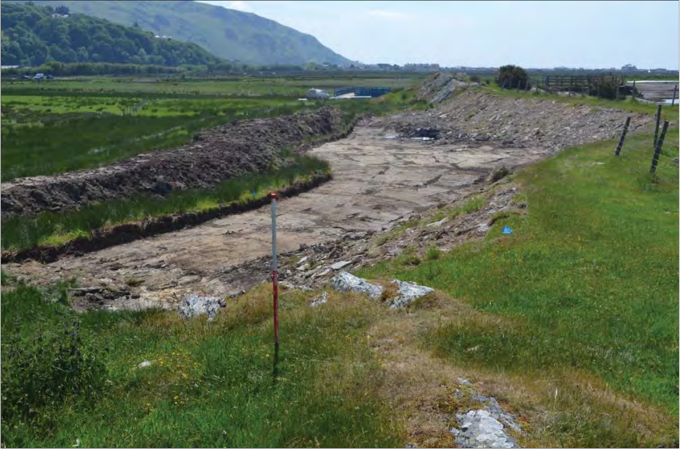
Plate 13: Topsoil strip of haul road east of the lime kiln. View looking west. Scale 1m
