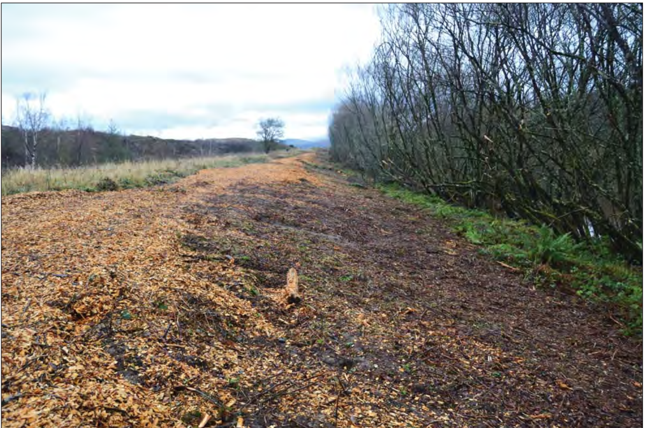
Plate 20. Gradually sloping eastern side of embankment; view from SE (photo ref: G2790_052)
