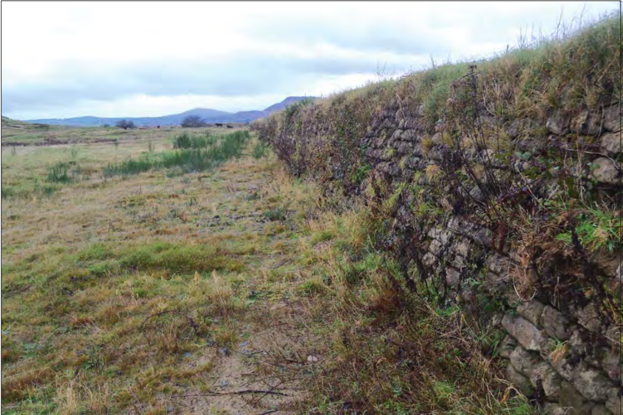
Plate 23. Revetment at northern end of embankment, showing the batter on the face of the revetment; view from S (photo ref: G2790_037)
