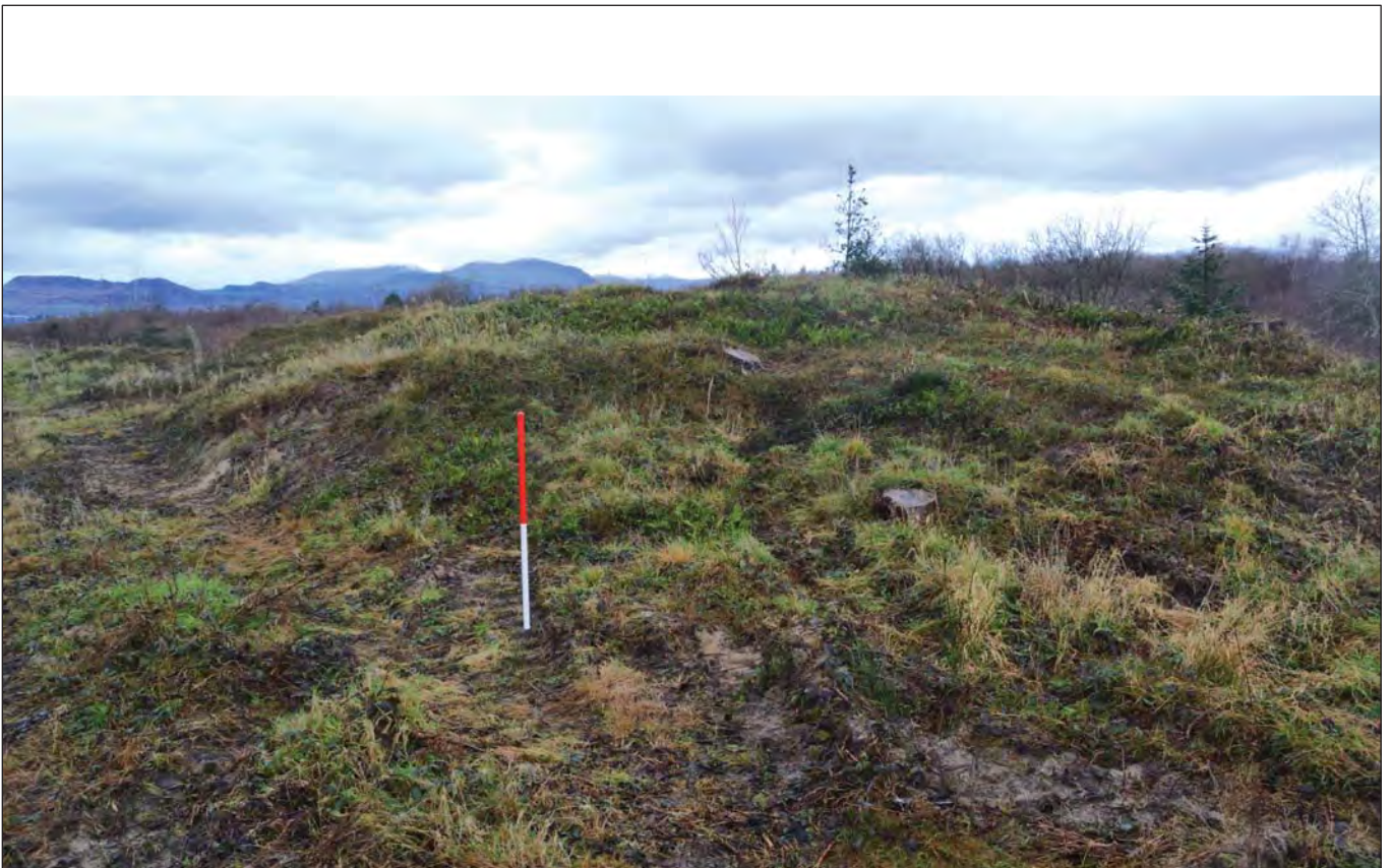
Plate 16. Small dunes built up over target railway embankment; scale 1m; view from SW (photo ref: G2790_027)
