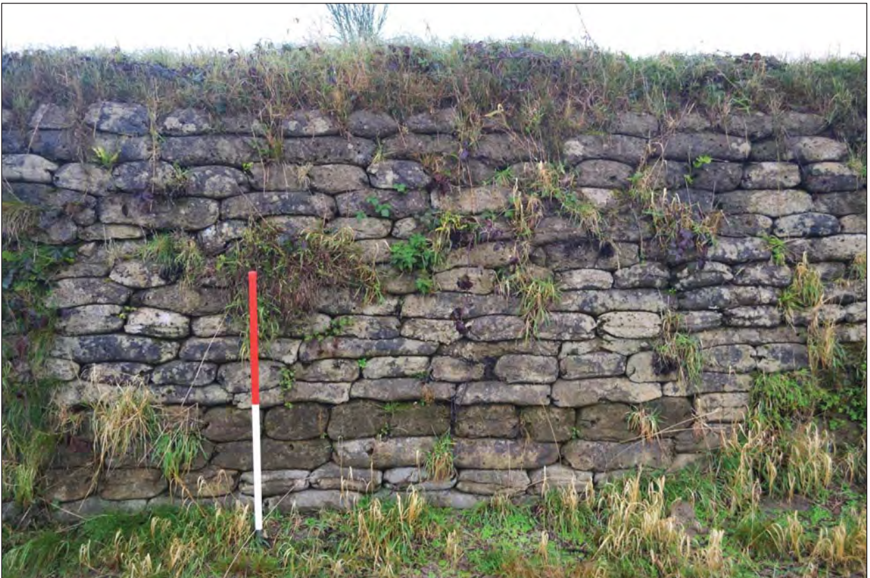
Plate 22. Revetment at northern end of embankment; scale 1m; view from S (photo ref: G2790_068)
