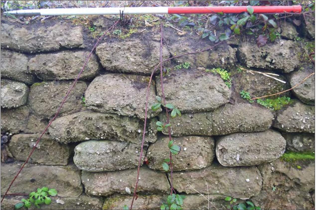
Plate 27. Example of concrete sandbags eroded to show stone content in the concrete; scale 1m; view from W (photo ref: G2790_013)
