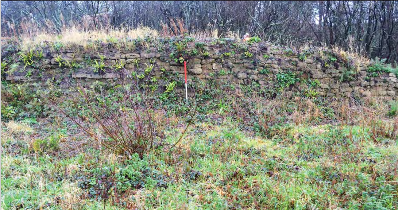
Plate 21. Revetment at southern end of embankment; scale 1m; view from SW (photo ref: G2790_010)
