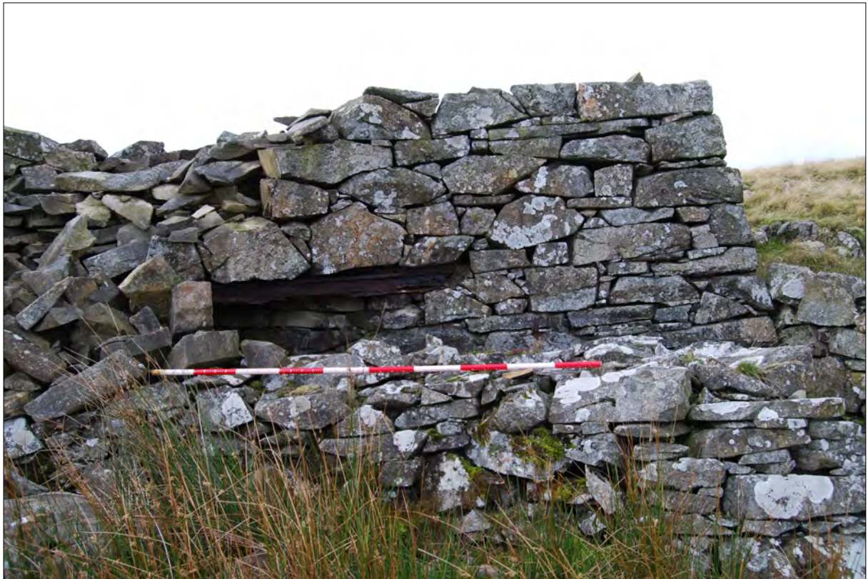
Plate 5. West facing image of the Observation building showing the collapsed canopy and railway I-beams.
