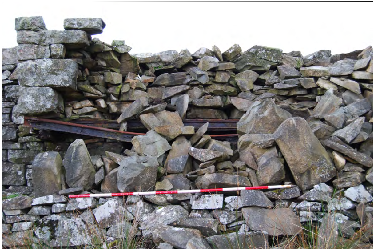
Plate 4. West facing image of the Observation building showing the collapsed canopy and railway I-Beams.
