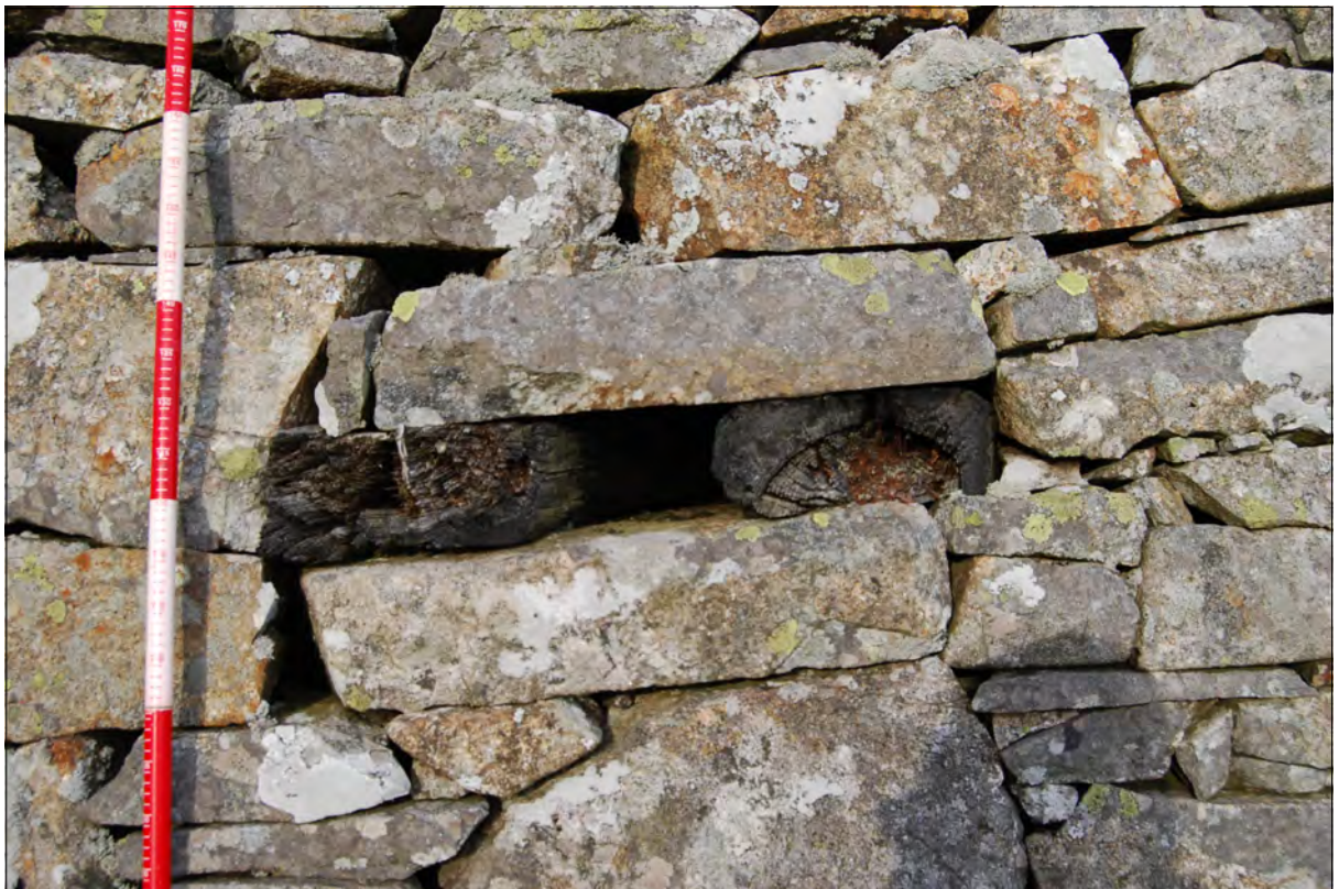
Plate 8. North facing image of observation hole presumably used to observe communications to the west
